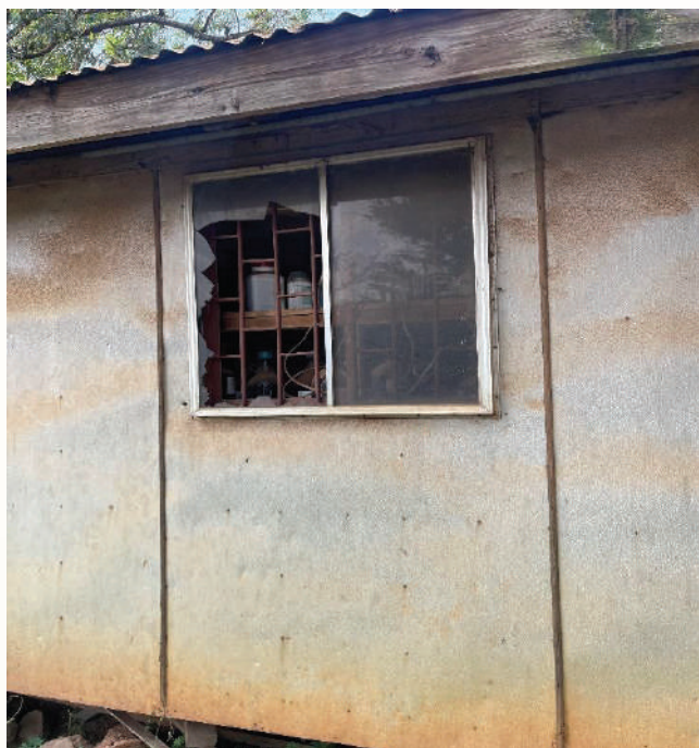
Broken window of the store containing equipment for disposal – Headquarters
