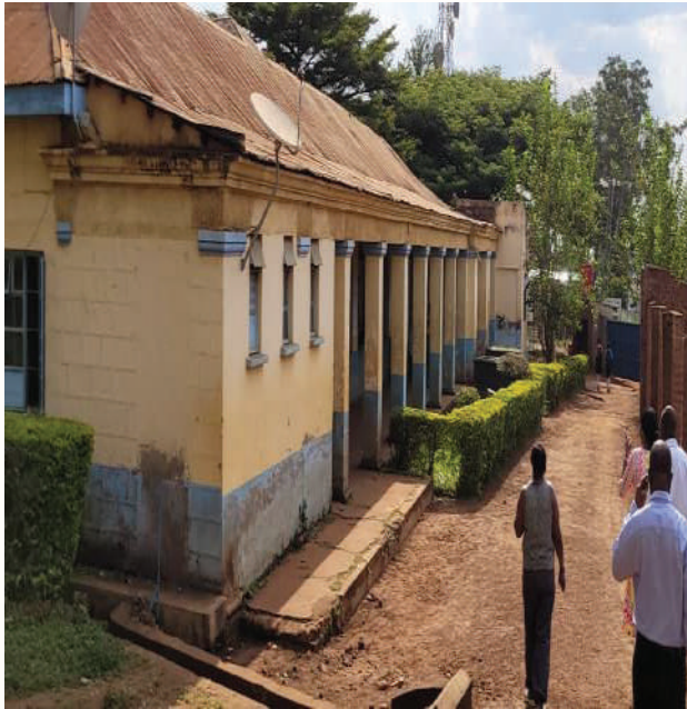
Abandoned school structure due to the laboratory at Rock HS falling ceiling to avoid damage to students- Rock High school – Tororo
