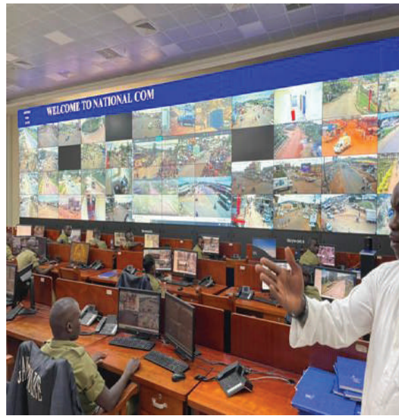
Surveillance room at NCCC Naguru.
