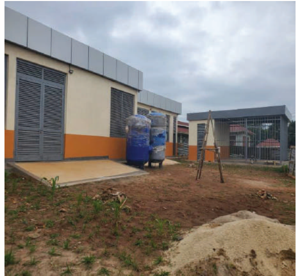
New Hospital Oxygen Plant
