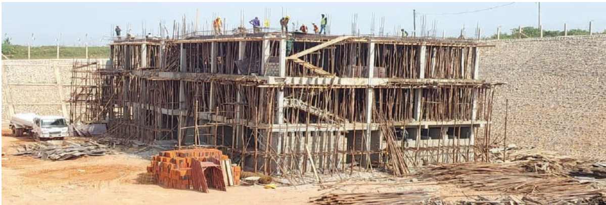
UFZA at Entebbe Airport Site Administrative Block with Stacked stock ready for use.
