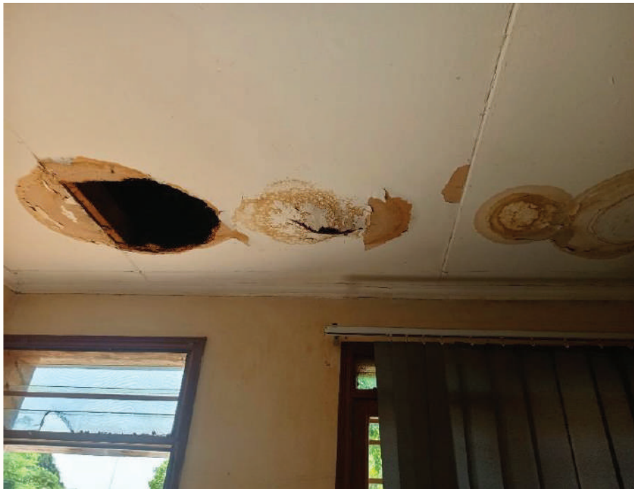
University Health Unit-Roof leaking and needs urgent renovation.
