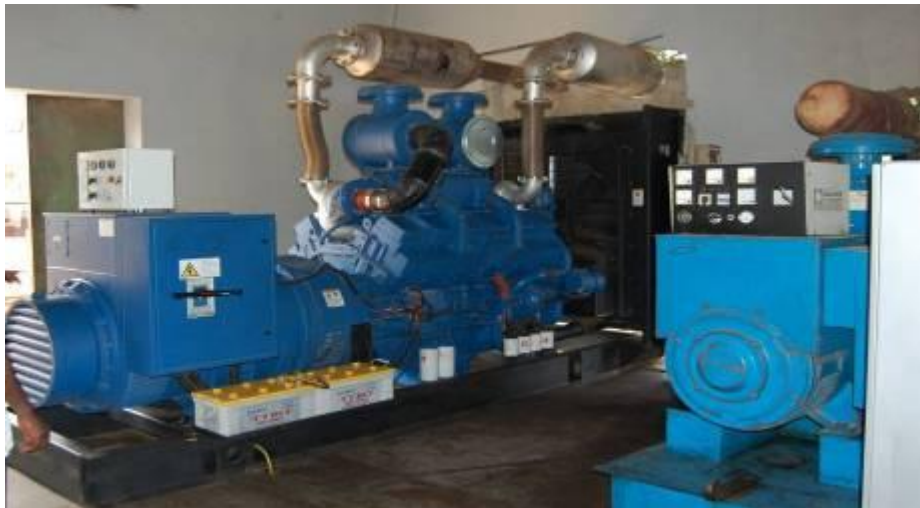
New 750KV generator (left) beside the old 350KV generator right in Adjumani UEDCL station
