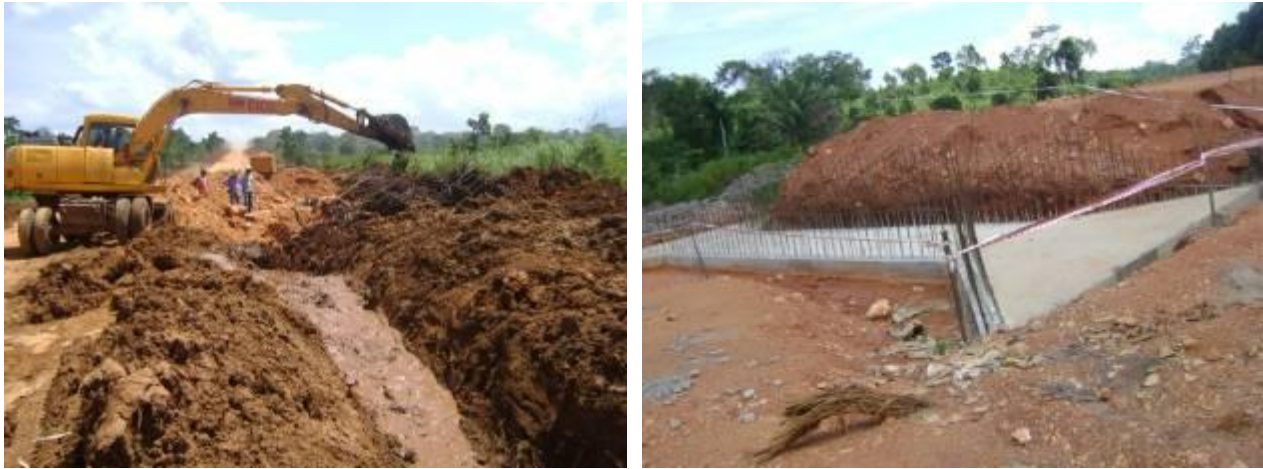
Picture shows on-going earthworks and construction of box culverts on Matugga – Semuto – Kapeka road.
