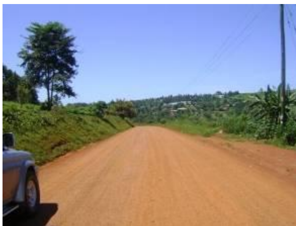
Picture shows a completed section done by force account on Lugazi – Buikwe road
