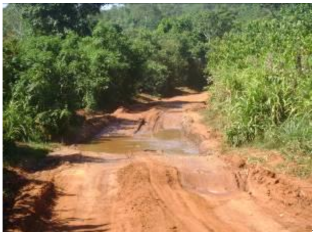
Picture shows a section of Lubugumu – Bugigi road in Mukono district where periodic maintenance was done
