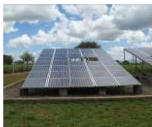
Energy package powering “24 hours water supply,” Cirofo SC
