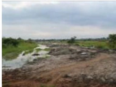
Impassable road leading to Olamia valley tank, which needs to be rectified by the contractor, Apac
