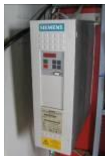
Mechanical problem with energy package, so no running water, Nyadri SC
