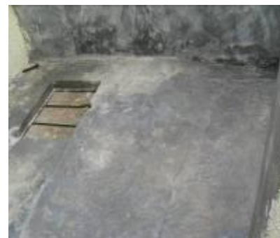
Newly constructed latrine with cracks, Isingiro District HQ
