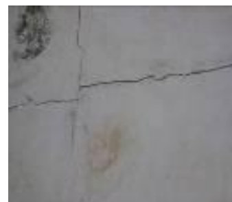
Eminent cracks in the ceiling of BugaboHC3
