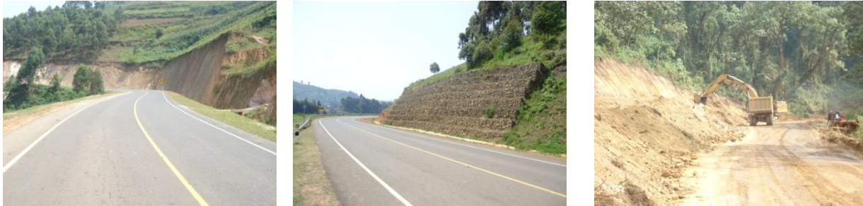
FIGURE 14 COMPLETED SECTIONS OF KABALE – KISORO, EROSION PROTECTION FOR THE EMBANKMENT AND EARTHWORKS ALONG THE INCOMPLETE SECTIONS OF THE ROAD.
