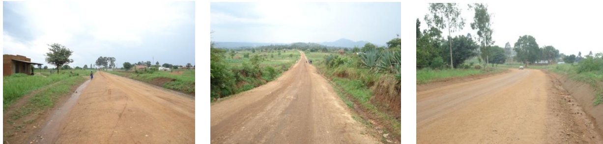
FIGURE 4 HEAVILY CORRUGATED SECTION AT 0+100 (KATRINI), COMPLETED GRADED SECTIONS OF THE ROAD AT 5+400 AND WIDE SECTION OF THE ROAD AT 19+500 ON THE APPROACH TO NYADRI
