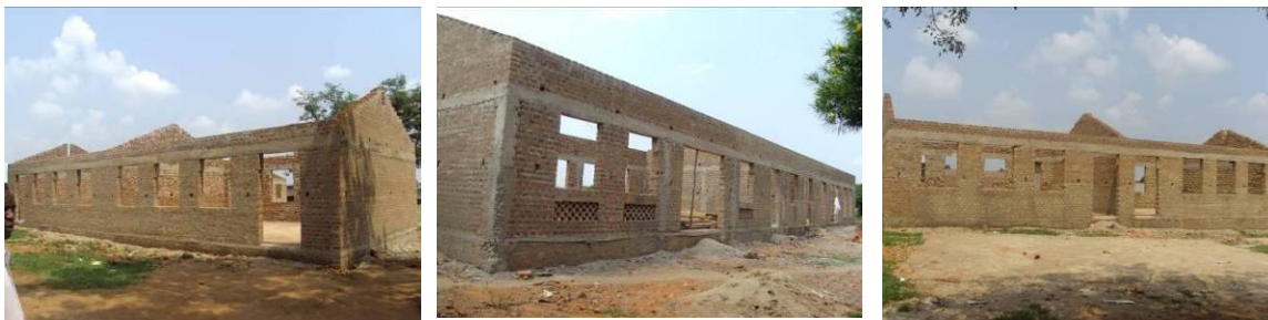
A 2 classroom block, a CJ and BCP workshop and another 2 classroom block at roofing level.
