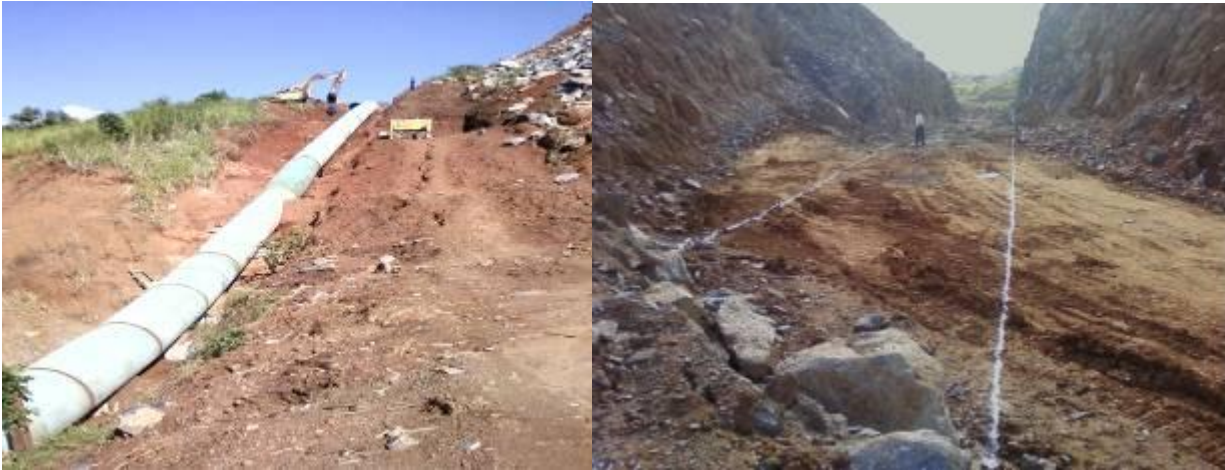
Nyagak HEP: ongoing works on the Penstock; Crushing of the rock almost complete
