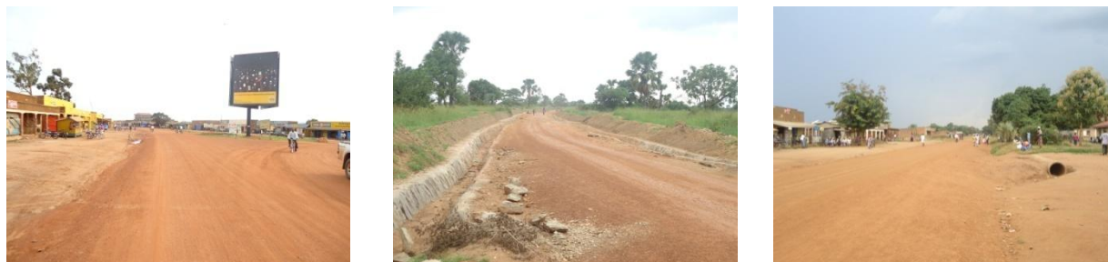
FIGURE 2 COMPLETED SECTION AT 0+000 (KOBOKO TOWN), STONE PITCHED DRAINS AT 7+400 AND INCOMPLETE ACCESS CULVERT INSTALLATION AT 28+300 (KURU TC)
