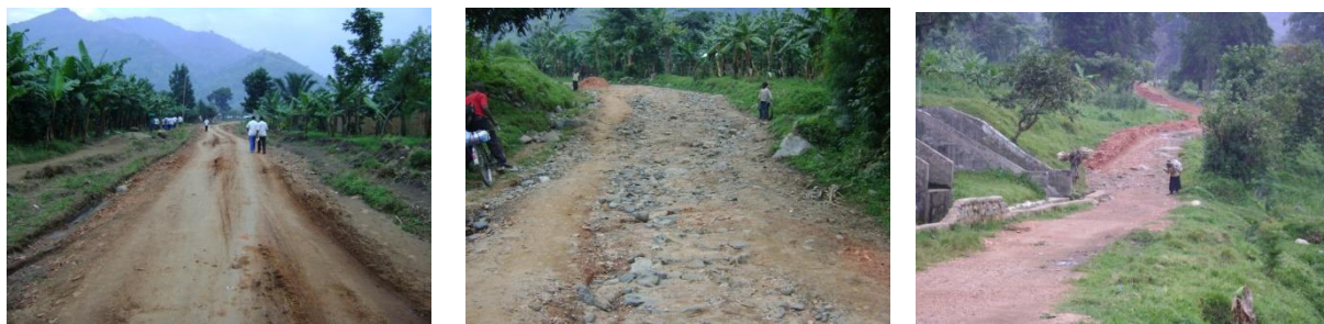
FIGURE 10 SECTIONS OF THE ROAD THAT ARE GRAVELLED BUT NOT WELL COMPACTED, ROCKY SECTIONS AND INCOMPLETE SECTIONS AFTER 14+300 AT THE KILEMBE HYDRO POER PLANT INTAKE.
