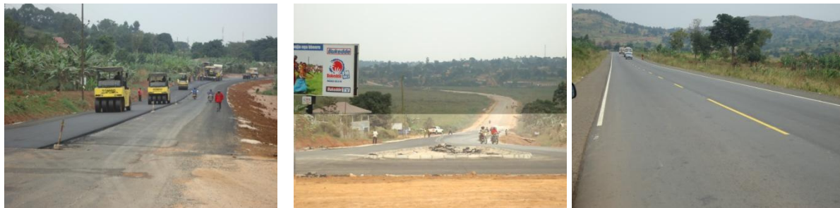
FIGURE 13 ASPHALT WORKS AT KM 120+200, IMPROVEMENTS DONE ON JUNCTION AT THE END OF THE BYPASS AND COMPLETED SECTIONS OF THE ROAD
