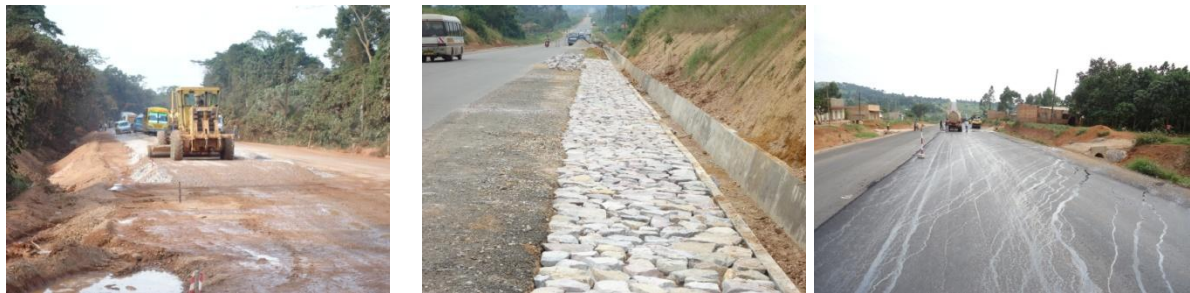
FIGURE 12: SWAMP RAISING, DRAINE WORKS AND CONSTRUCTION OF THE ASPHALT WEARING COURSE ALONG KAMENGO TO LUKAYA SECTION
