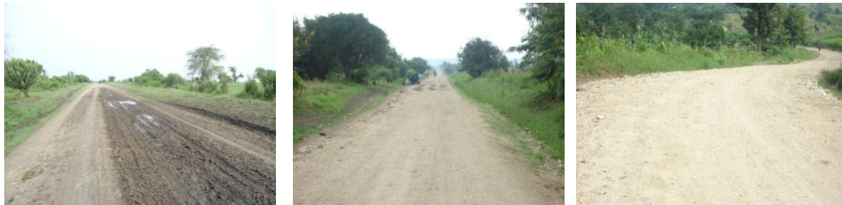
FIGURE 9 LACK OF COMPACTION HAS COMPROMISED THE VALUE OF THE MAINTENANCE INTERVENTIONS ON THIS KATWE – KATOJO – BWERA ROAD
