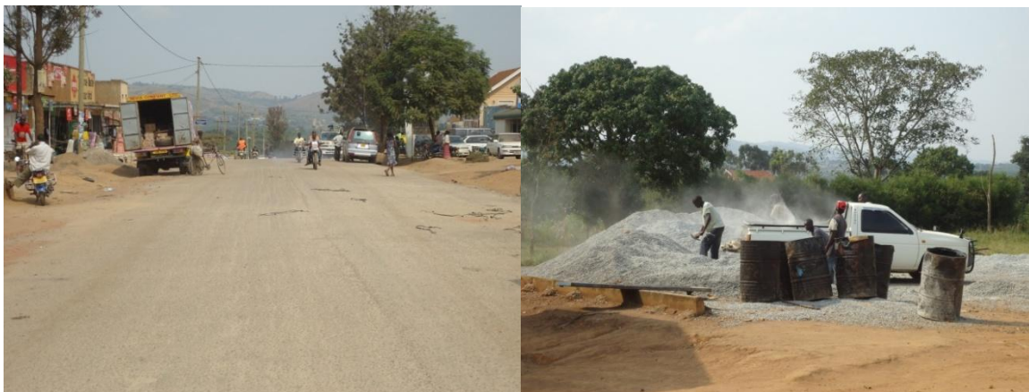
FIGURE 17.1A RESEALED SECTION OF MARKET STREET WITH THE SECOND BITUMINOUS LAYER (LEFT); ADDITIONAL CHIP STONE AND BITUMEN WAS ALSO SEEN AT THE TOWN COUNCIL YARD
