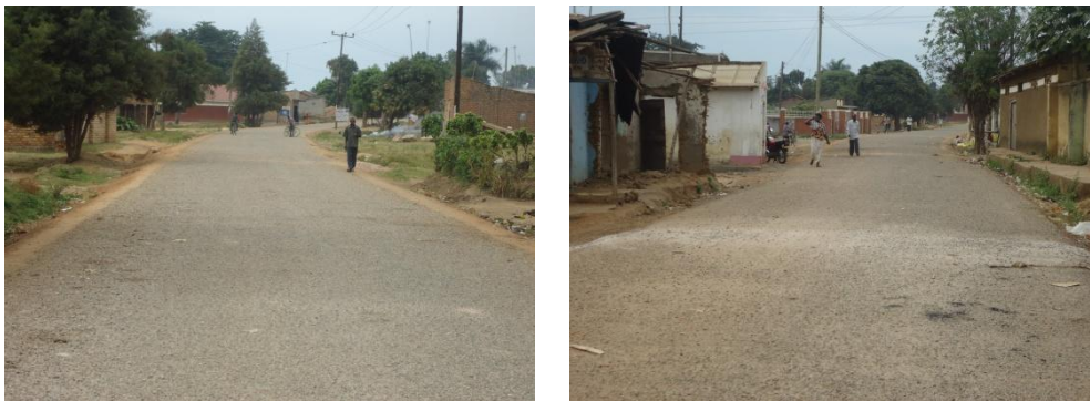
FIGURE 16 A RESEALED SECTION OF MARKET ROAD (LEFT); A RESEALED SECTION OF SEMPIJJA-BULINGO ROAD.(RIGHT) WITH ONE SEAL AND UNPROTECTED SIDE DRAINS.
