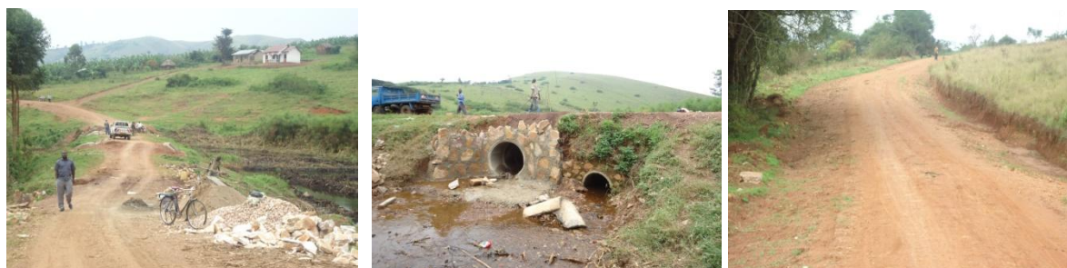
FIGURE 16 CONSTRUCTION OF CULVERTS ALONG KAGARAMA – KATINDA ROAD AND COMPLETED SECTIONS ON KASHANDA NYARWAMBU ROAD.
