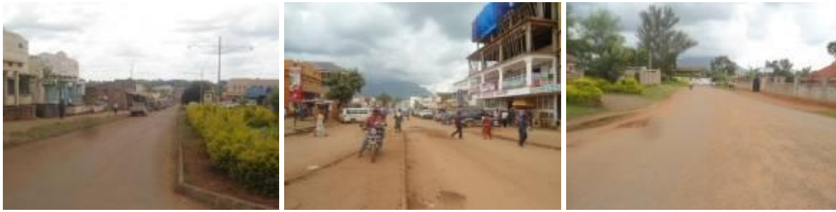
Parts of Naboia road and at the end that have the chippings stripped off (left and right) and potholes have developed before the hand over of the road at Km 0+000 (Centre)
