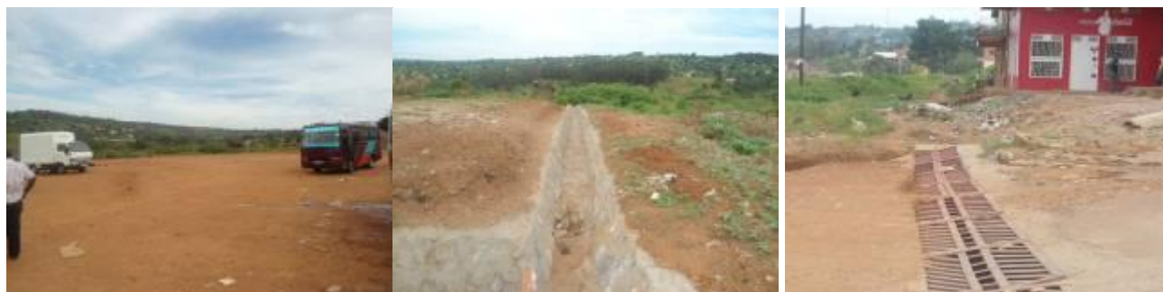
Stabilised murrum that was provided for the lorry (left); Surface drainage works around the lorry park. (centre); Drainage channel along Ssesse street.
