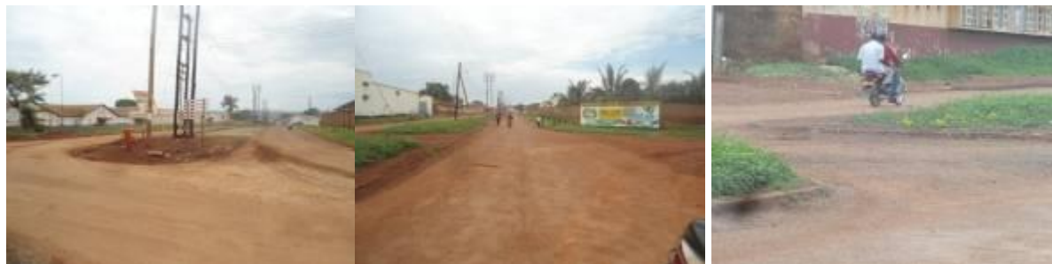
Concrete and second seal work at the Factory road junction (left); End of second seal works near Nile Ply (centre); and stripped surface in the island caused by heavy truck turning near Nile Ply (right)
