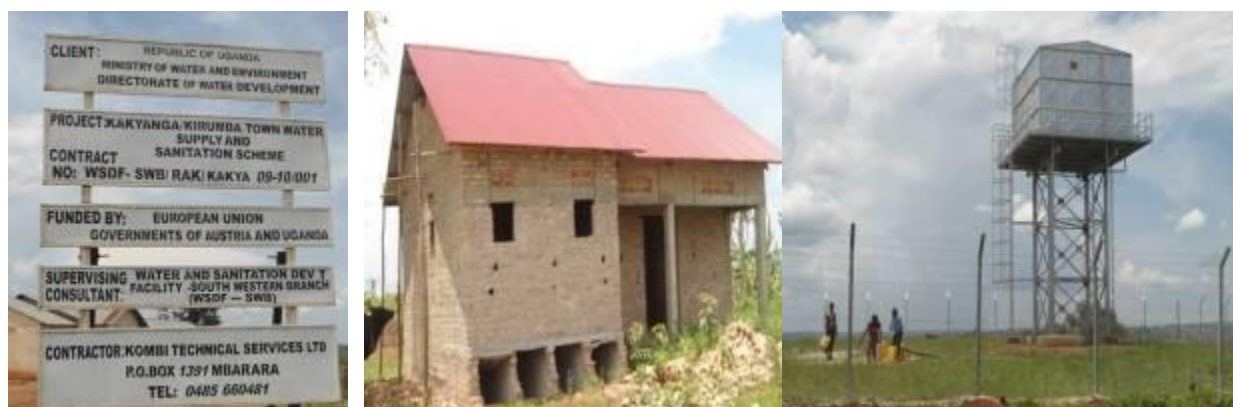
Photos 10, 11& 12 for the Kakyanga office block still under construction and Reservoir tank ;( inset people collecting water at no cost).
