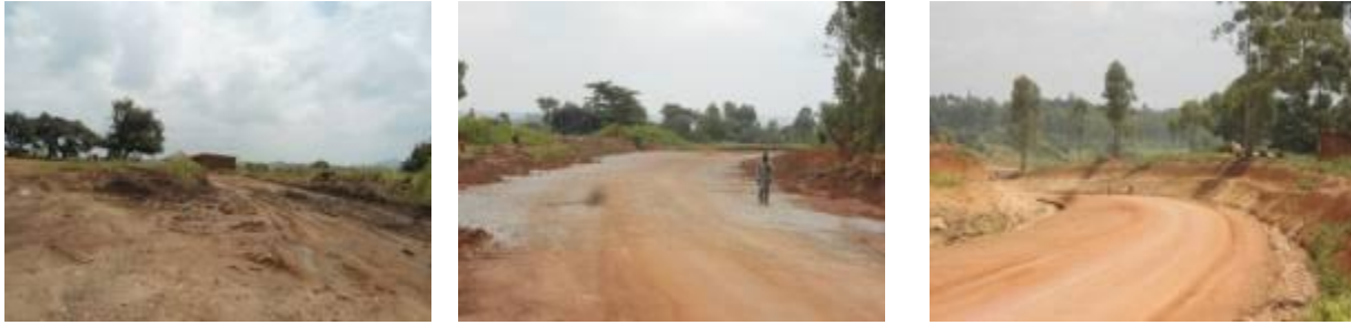
(Left); A section of the road at Km 61+930 where compensation issues have hindered clearing works. A grave and a house remain in the project area. (Centre): A section at Km 59 that is being maintained especially for heavy traffic that is using the road. (Right); Section of the road at Km 41 where the road has been cut to reduce on the gradient and subgrade works have been completed.
