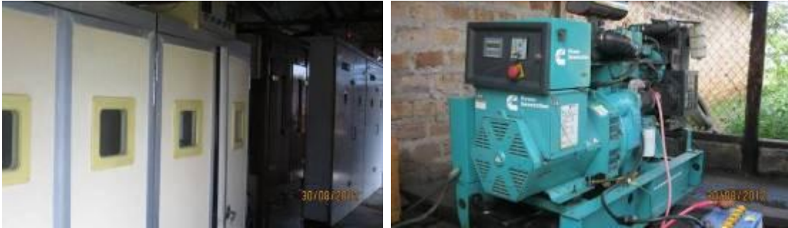
Left: ACF funded incubator on the left Right: ACF funded generator
