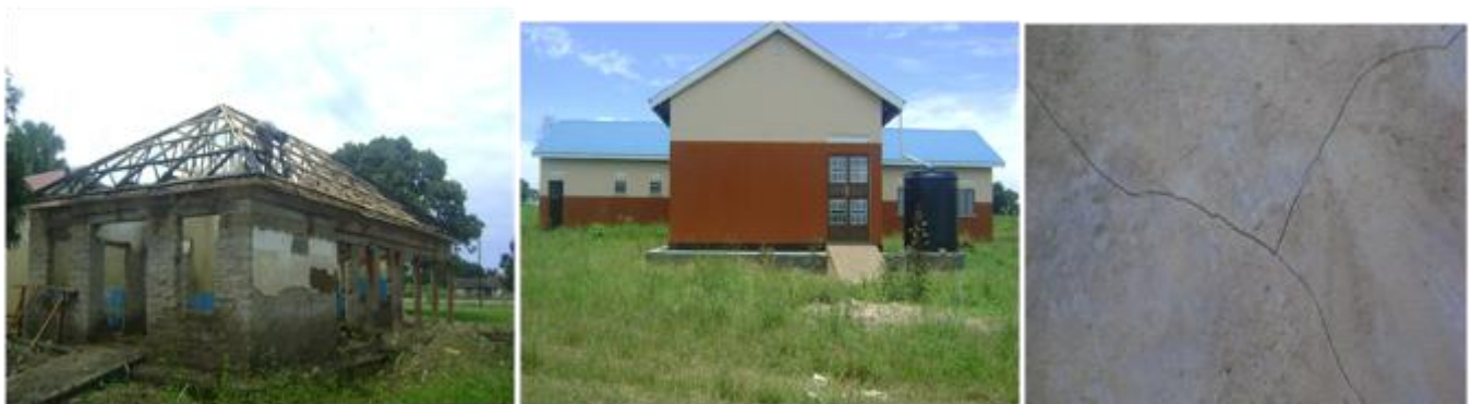
Dokolo district PHC development: renovation of OPD at Dokolo HCIV; maternity ward at Atubu HCII; large cracks in floor of the maternity ward at Atubu HCII
