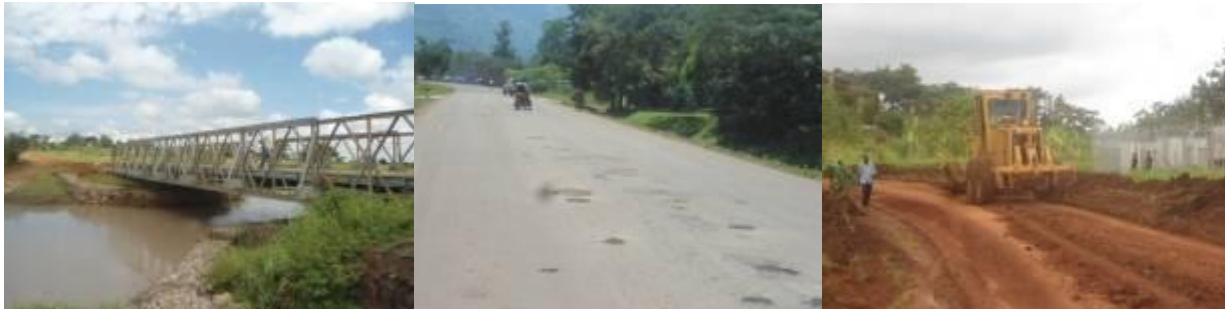
Kite –Kawanone bailey bridge (left); Section of SironkoMuyembeKapchorwa road where patching works were done but potholes are still coming up. (centre); Grading works ongoing on MbaleBufumbo road. (right)
