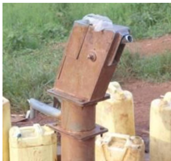
A vandalized borehole in Najembe S/C Buikwe
