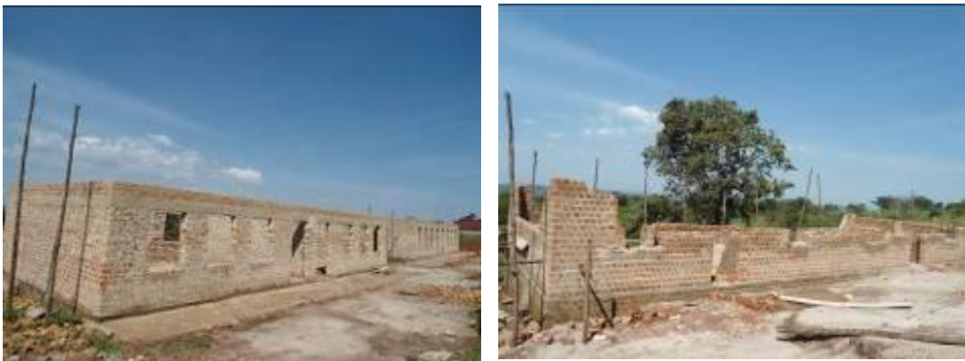
The 2 classroom blocks at ring bim level and the teachers' house at window level at Butoloogo Seed S.S
