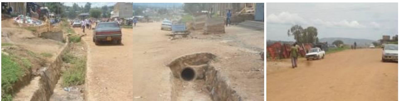
An open channel that is silting due to rubbish dumped in it. (left); A 600mm culvert line installed. (centre); The well graded, gravelled and shaped road surface. (right) on Major Victor Bwana road
