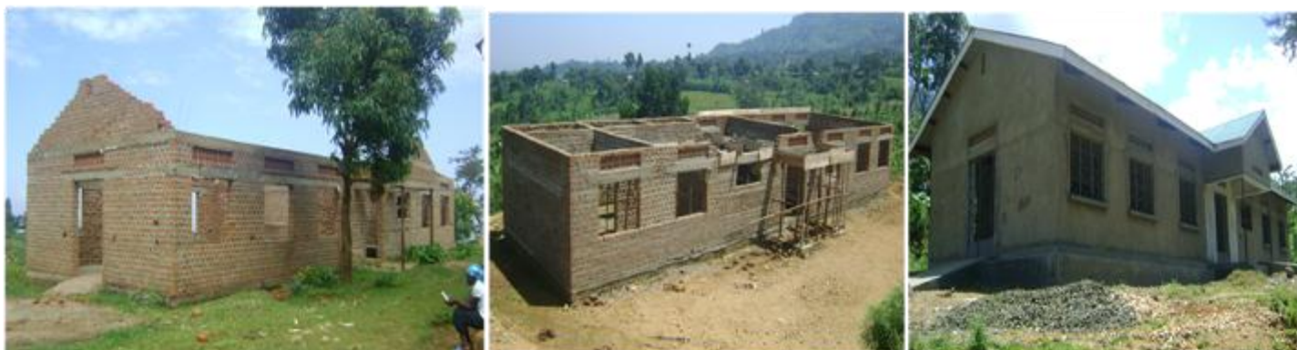
Mbale District PHC development: maternity ward at Bungokho Mutoto HCIII (left); maternity ward at Naiku HCIII (centre); maternity ward at Buwanga HCIII (right)
