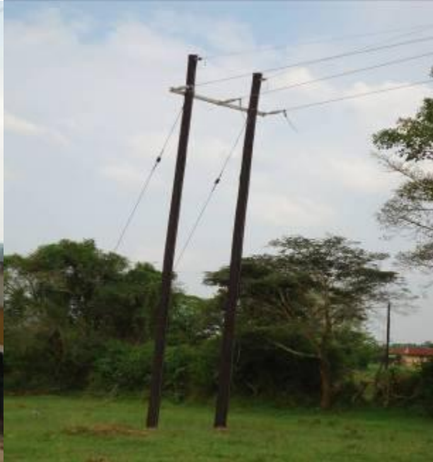
End Point of Ibanda-Kazo-Rushere line
