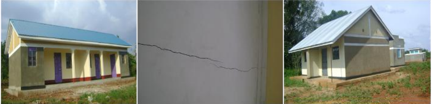
Kamuli district PHC development: staff house at Luzinga HCII (left); cracked ceiling in staff house at Luzinga HCII (centre); staff house at Namaira HCII (right)
