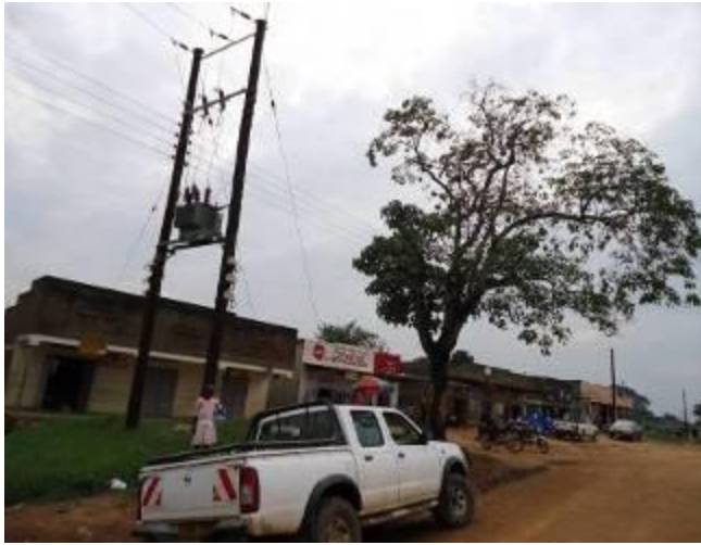
Trading center likely to connect to power on Ibanda-Kabujogera-Kamwenge line
