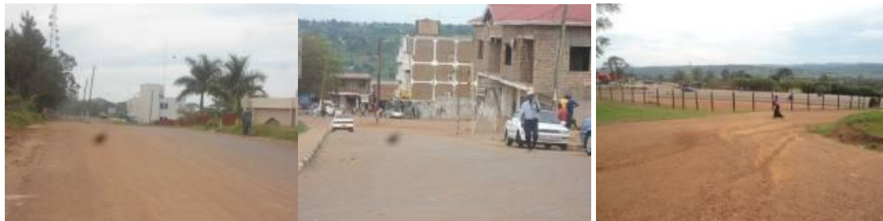
Resealing works on Victoria road (left); Noor road with first seal completed. (centre); Access to Auditor General’s Office with gulleys forming on the road surface (right).
