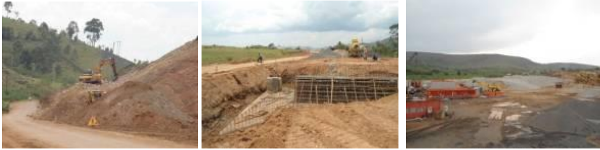
(Left): Rock excavation works along slopes; (centre); Construction of a concrete box culvert across the road at Km 67+800; (right) the stone quarry that is already in production of aggregates.
