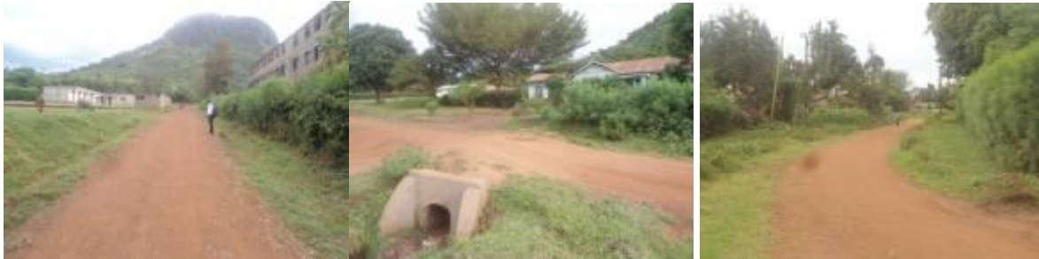
Well graded and gravelled 100m Access road (left); A newly installed culvert on Bukedi road. Note the depression at the far end of the culvert line which indicates a broken culvert. (centre); Hyena drive (right)
