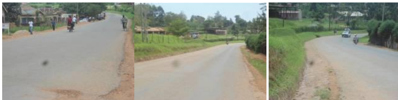
Beginning of sealing works near Ntare School gate (left); Surface dressed road surface still in good condition. (centre); and Drainage works. (right) on Ntare road
