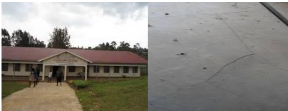
Complete structure and cracked floor in Kinyansano ICT lab.
