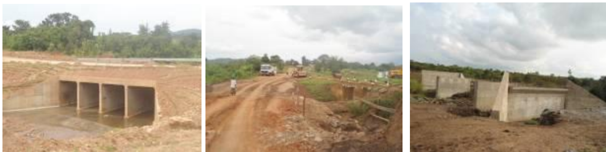
(Left): Completed Amua box culvert with guard rails installed; (centre); Completion of diversion works for Ebikwa box culvert works; (right) Incomplete Irei Bridge works with no deck.
