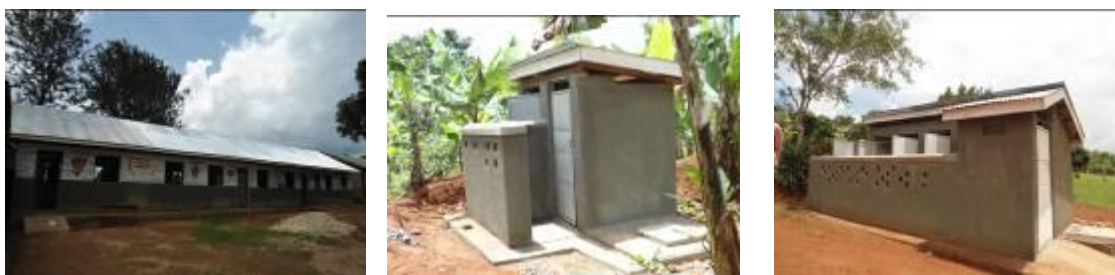
A renovated 4 classroom block, a newly constructed 2-stance and 5-stance VIP pit latrine at Kalububbu Muslim P/S
