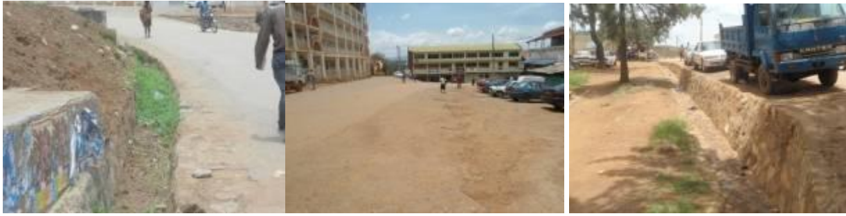
Silting in an open channel (left); sealed road shoulder (centre); and the 100m open drainage protected with stone pitching. (right) along Bananuka drive.
