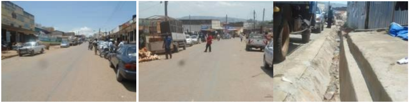
Surface resealing works Street (left) and (centre); Storm water channel (right) on Makhan Singh
