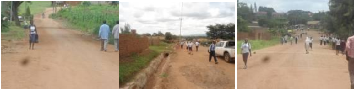
Graded section of Nkonkojeru Court road (left); Drainage works along Kakungulu drive (centre); and completed first seal of DBSD on Kakungulu drive (right)
