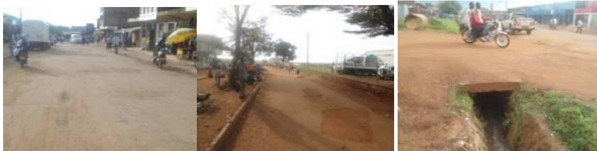
Stripping of surface on Togore Road West (left); Pot holes appearing on Obuya Lane (centre); and the newly installed box culvert on Park Lane. (right)
