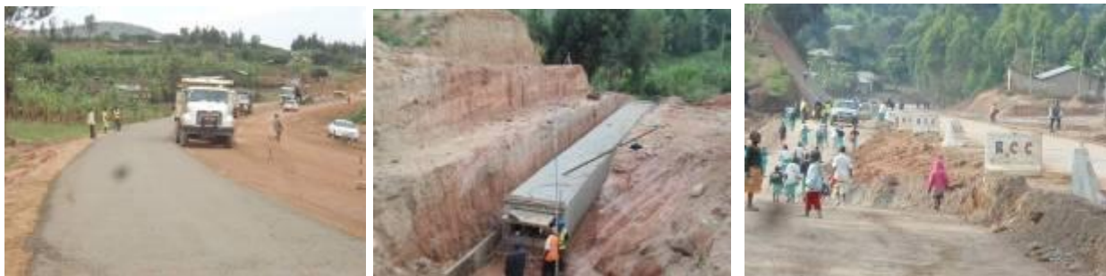
(Left): Base course works ongoing at Km 98+650; (centre); Installation of a 1.5m by 1m high culvert crossing at Km 100+488; (right) filling of embankment. Take note of the safety precaution taken by the contractor for the traffic using the project road.
