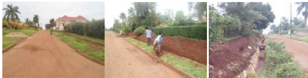
First bitumen seal (left); Excavation of side drain (centre); and stone pitching of side drain (right) along Madhvani road
