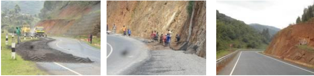
(Left); Completed section of the road where scarifying was ongoing. (Centre): Construction of a concrete line open drain. A section of the road at Km 8+300 yet to be surface dressed. (Right); Completed section of the road with the centre line not yet marked..
