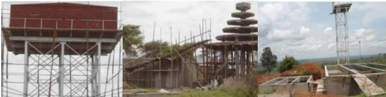
New Reservoir, aerial & sedimentation tank, sand driers and old reservoir for Lyantonde town water supply
