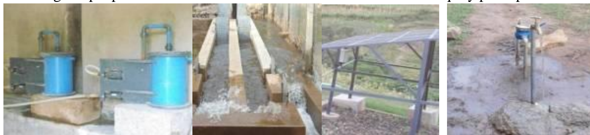
The Chemical doser Unit, the Gabion protection at intake, the solar panels and tap with water running (Tororo-Manafwa GFS)
