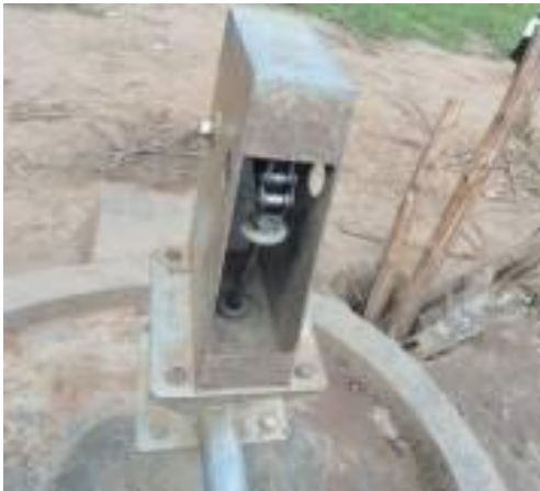
Vandalised BH pumphead at Kanani Buwama S/C.
