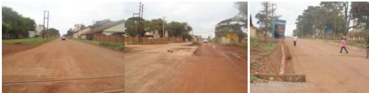
Completed section of the road at Railway crossing (left); Junction with Factory road with unfinished reinforced concrete works (centre); and stone pitched side drain works (right)
