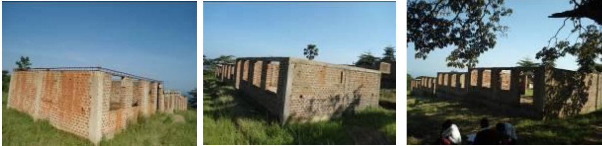
2 blocks of 3 classrooms and a 4 classroom block that stalled at Semiliki High S.S. (APL I World Bank Project).
