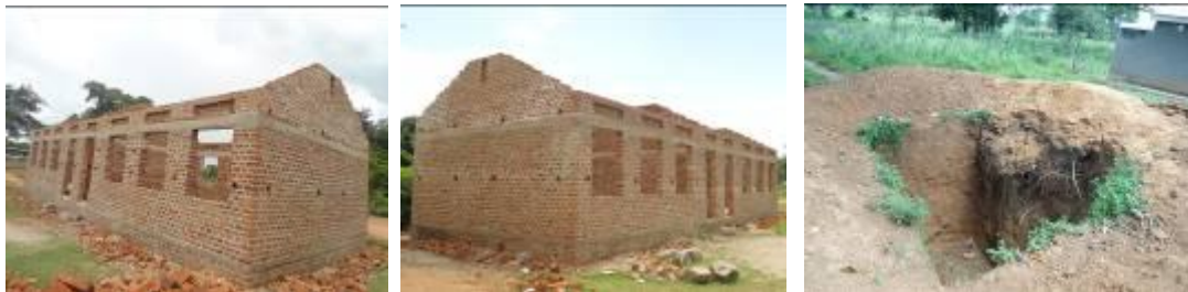
The 2 blocks each with 2 classrooms at whole plate level and the 2-stance VIP pit latrine at excavation level at Bugwe P/S
