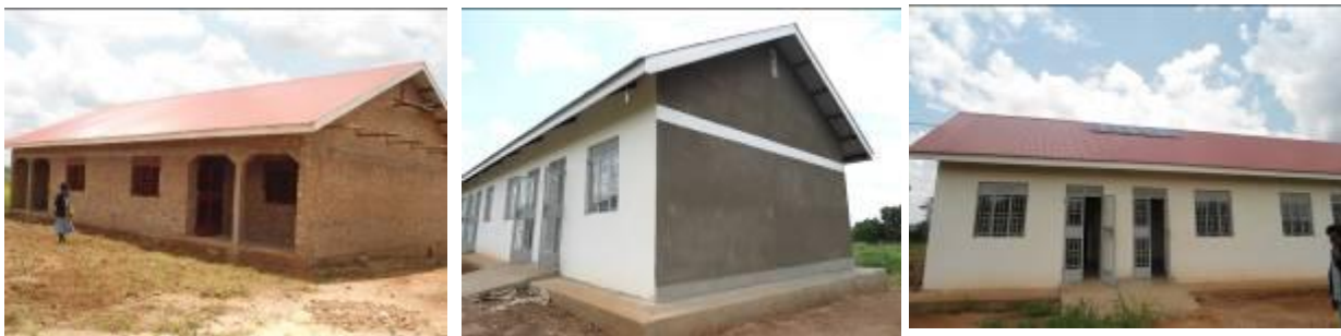
A semi detached house at finishes level, and the 2 completed staff houses at St. Edward College -Galamba
