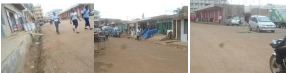
Open channel drainage works in taxi park. (left); Finished second seal works (centre); and Finished second seal works and a manhole for underground drainage. (right)
