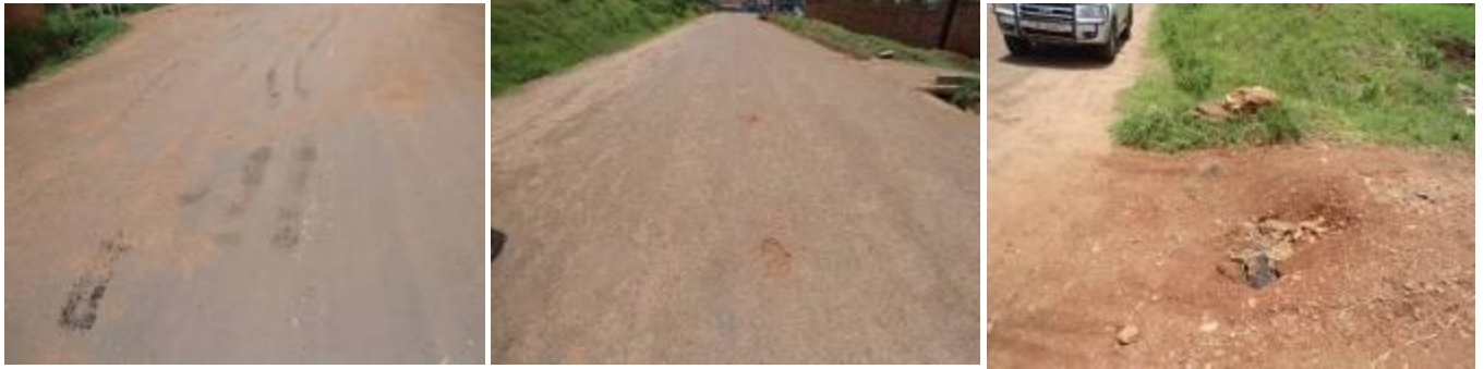
A section of Bweyogere park bleeding roads, potholes, failed culverts and incomplete drainage
