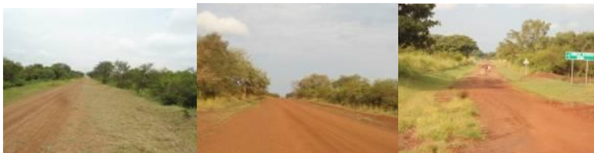
A graded section of MoyoObongi road where slashing of the road side was ongoing (left); A regavelled section of LaropiAyugi road. (centre); A graded section of DzaipiBibia road whose road surface was defecting due to poor compaction. (right)
