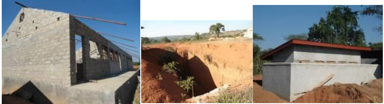
A science laboratory at roofing level, a pit latrine behind the laboratory abandoned at excavation level and another VIP latrine left finishes level at Kalisizo S.S.
