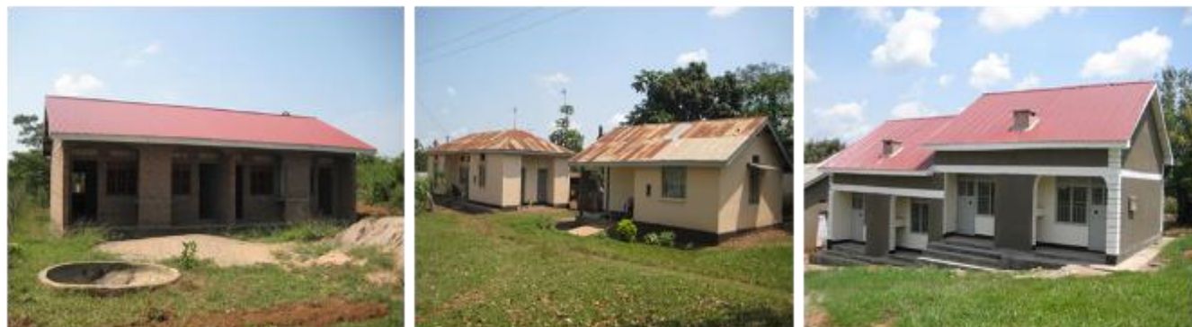
Left to Right: Staff house construction at Nakyesa HCII, Rehabilitated staff quarters at Ntenjeru HCIII and Staff house at Nazigo HCIII
