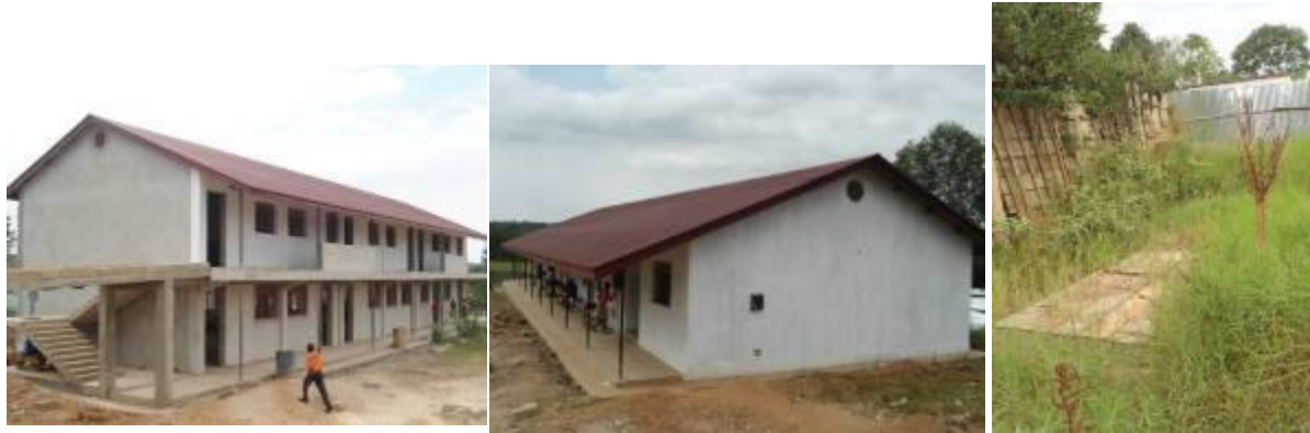
A multi purpose storied block, library with computer laboratory and a 3 stance VIP abandoned at slab level at Bulamu Seed S.S.
