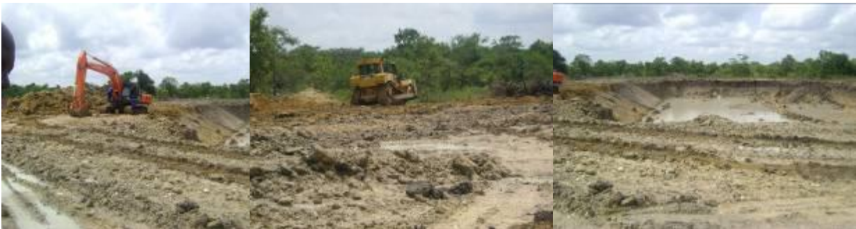
Left: Excavator working on dam Middle: Bush clearing Right: Excavated dam of Mr. Nkoyooyo in Nakasongola district
