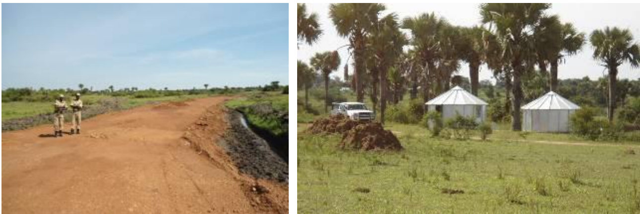
Earth works along Temele road and two uniports accommodating police in Soroti park
