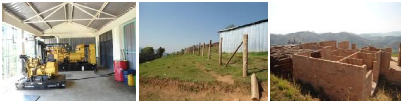
Installed factory generators, improvised barbed wire fence and stalled Buhweju Tea Factory staff houses
