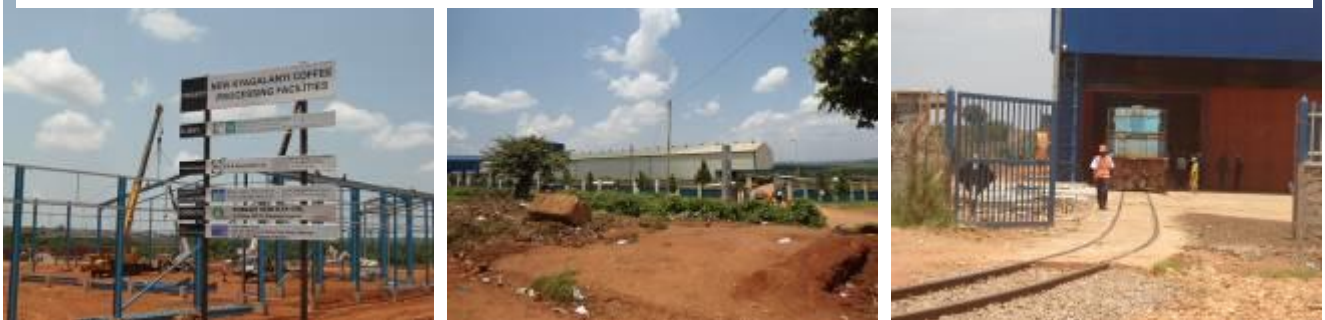
Construction of Kyagalanyi coffee factory, completed Roofings premises and a side railway truck to Roofings factory
