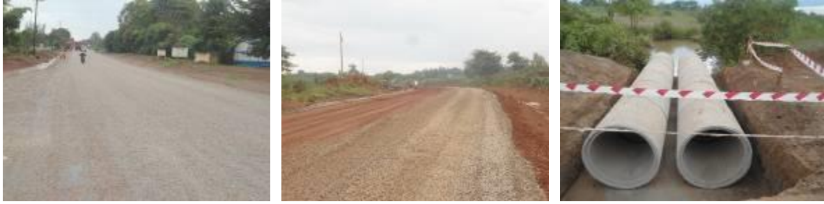
(Left); DSBT wearing course works at the start of the project in Tororo; (Centre): Base course works (50% aggregate and 50% gravel) at Km8+100; (Right); 900mm diameter culvert installation at Km24+600.
