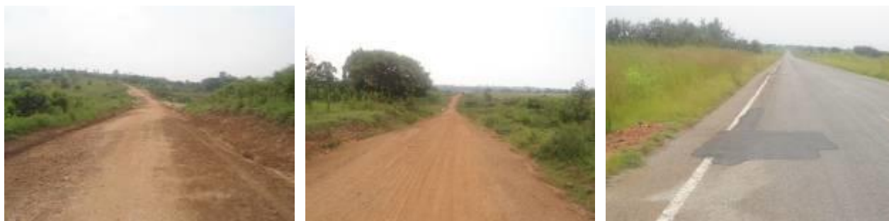
Nyadri-Katrini road (23Kms) at Km 1+900 showing a spot gravelled section with LBC works of road side and drainage cleaning (left); A regrevalled section of Arua-Muni PTTC-Erubu road (6Kms) at 3+000 (centre); Patch works along Arua-Nebbi-Packwach road at Km120+000 (right).
