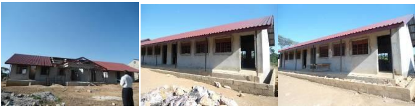
An administration block, 2 blocks of 2 classrooms each left incomplete at Kalisizo S.S
