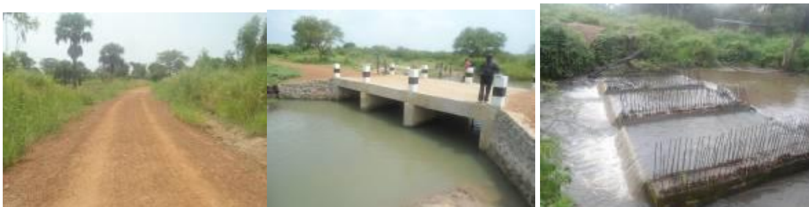
Re-gravelled section of Mile10-Inde (12Kms) road at Km 8+500(Left); Kereluva 3 cell box culvert without guard rails (Centre); Foundation works on Werike box culvert (Right).
