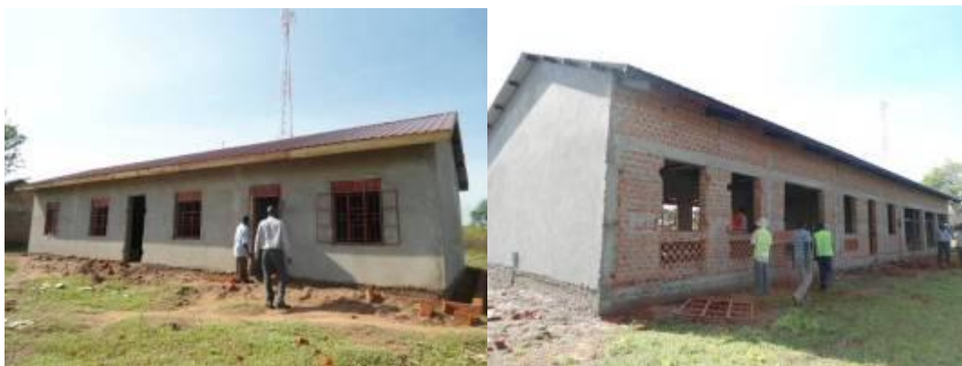
A 4 unit teachers house and the twin workshop constructed at Magoro Comprehensive S.S
