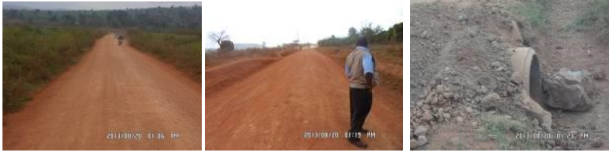
(Left): A regavelled section in a swamp at Km 1+400; (centre); a poorly graded section with raised road center line at Km11+400; (right) A 600mm culvert line installed with no head walls at Km 11+800.
