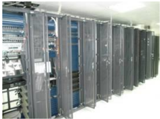
NBI secondary data centre at Statistics House
