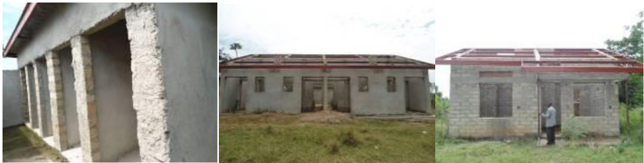
A stalled 5 stance VIP pit latrine, a 4 unit teachers' house and a 2 bed roomed head teachers' house that stalled at Bulamu Seed S.S.
