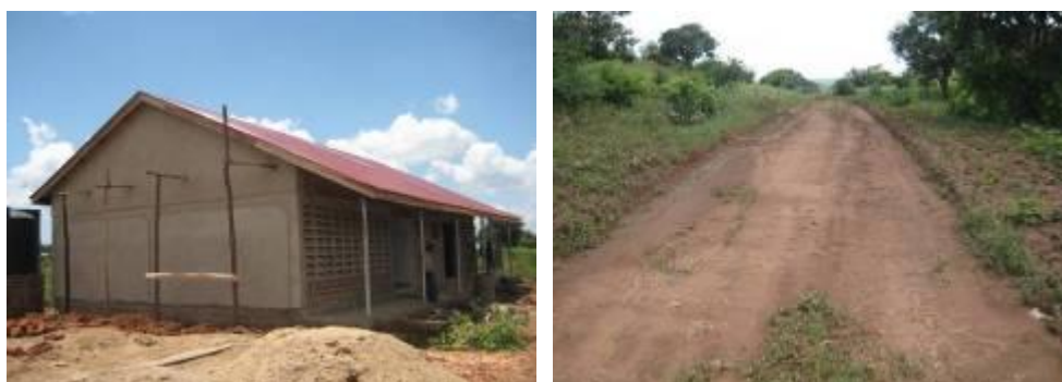
Construction of staff house at Irima HCII and opened road to the mortuary Nakasongola HCIV
