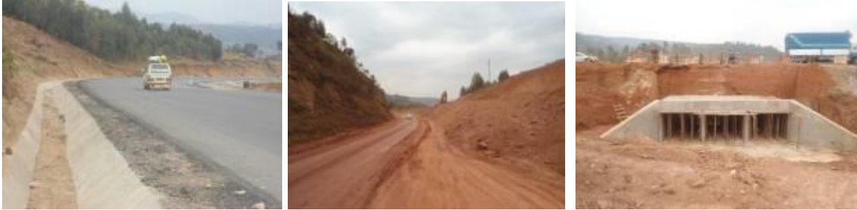
(Left): A concrete lined drain and wearing course road works at Km 108; (centre); Earthworks involving clearing and grubbing at Km 123; (right) A 2.5m by 2m, 3 cell box culvert at Km 136+600 under construction near Kabale town.
