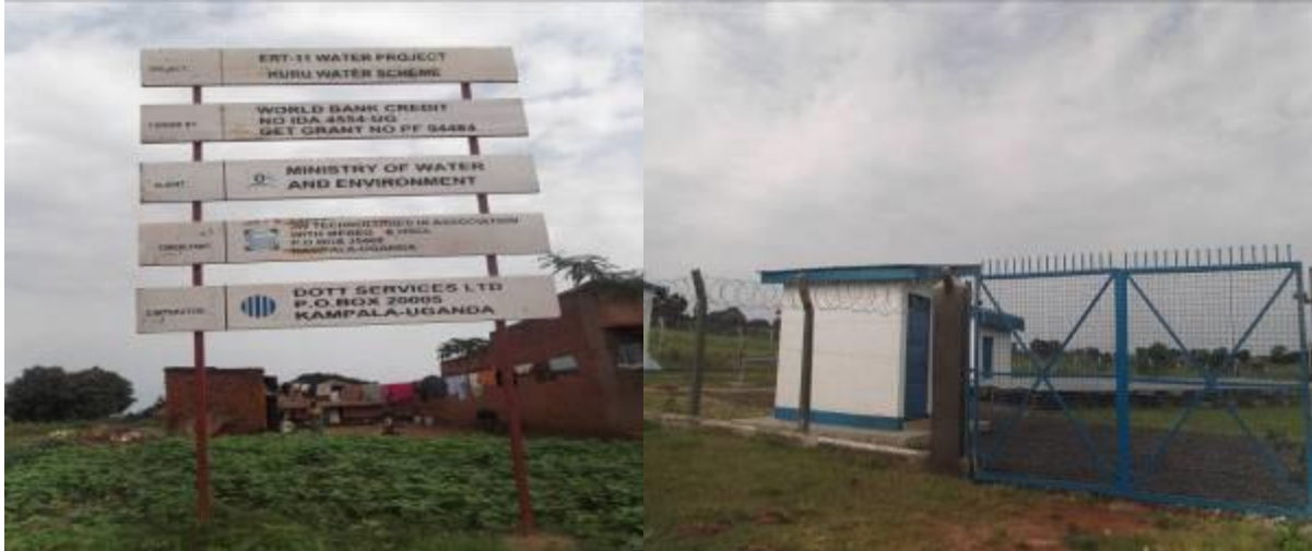
Kuru Solar Water Pumping station (Yumbe)
