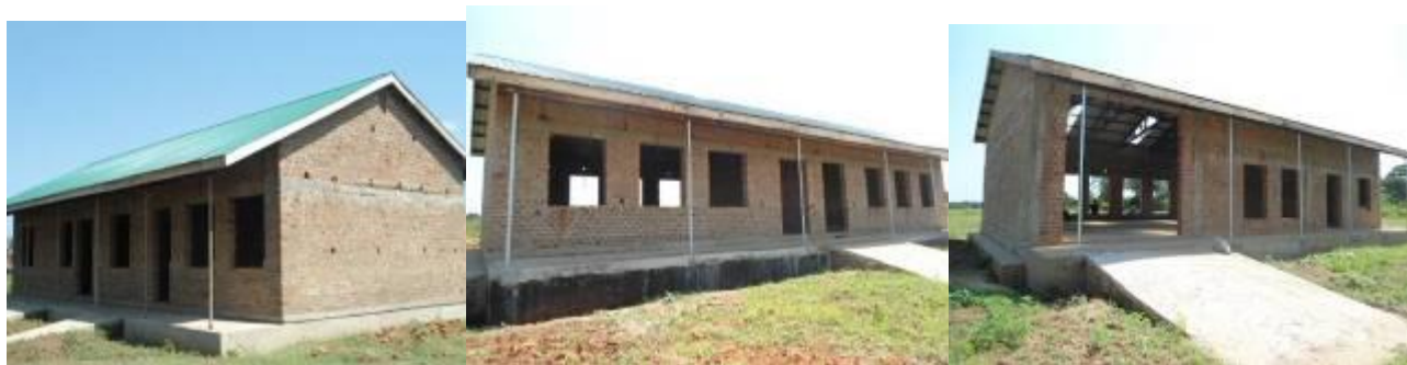
An administration block, a 2 classroom block and a CJ/BCP workshop constructed/stalled at Buseesa T/I
