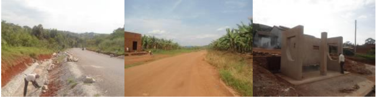
(Left); Ongoing stone pitching works at Km93+000; (Centre): A skipped section at Km 99+650 stretching for about 2Kms due to pending compensation issues; (Right); An incomplete structure at one of the bus stops.
