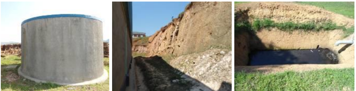
100 cubic meter water tank, embankments affected by soil erosion and affluent water lagoon
