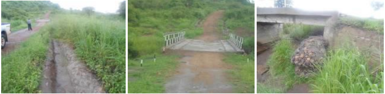
(Left): Stone pitched drainage along the access road to the bridge; (Centre): Completed bridge decking with side rails installed; (Right): Gabion protection works that were poorly constructed.
