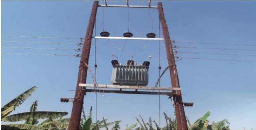
Jumpers cut off the transformer to steal the oil and copper in transformer
