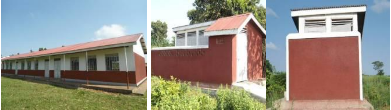
A 3 classroom block, a 5 and a 2 stance VIP pit latrines respectively constructed under the Presidential Pledge at Walibo S.S.
