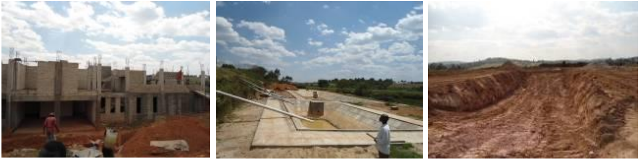
Ongoing block works at the research complex, lined lagoons and excavation of the water reservoir at Nyaruzinga
