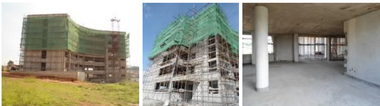
Completed shell structure, and ongoing outer and internal finishes of UNBS headquarters
