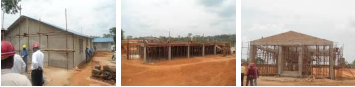
(Left); Water pump and power house construction at 90% completion; (Centre): Office block at 20% completion; (Right)); Weigh bridge house at 80% progress.
