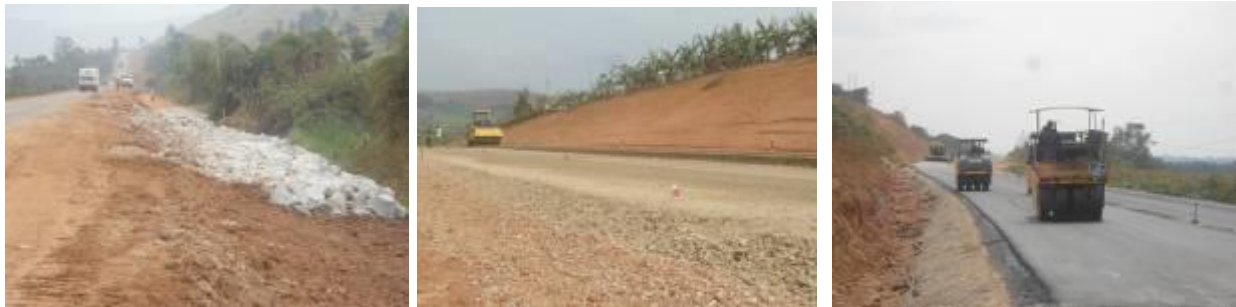
(Left): Rock fill – Swamp treatment works at Km 54+179; (centre); freshly applied base course works in 2 layers of 140mm to make 280mm at Km 66+99; (right) Finish works on DBM at Km 71+600.
