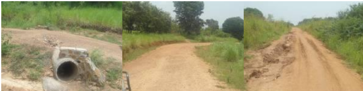
Sections of Lukuma-Mengo (7Kms) road: (Left); A broken culvert at Km 1+200, (Centre); A motorable section. (Right) Otumbari-Yoro (19Kms) road - A dilapated section of the road at Km 17+800 showing damage (gullies) caused by the rains as a result of poor drainage.
