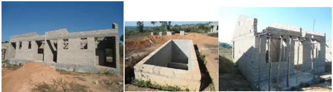
A 4 unit teachers' house, a 5 stance VIP abandoned at slab level and a 2 bed roomed house abandoned at roofing level at Kalisizo S.S.
