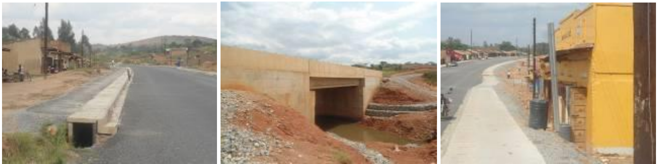
(Left); An urban drain at Km73 + 500 in a completed section without road marking; (Centre): completed Bridge 2 at Km 78+000; (Right); Compensated property in Kanoni town at Km 83+312 that is still in the road reserve.
