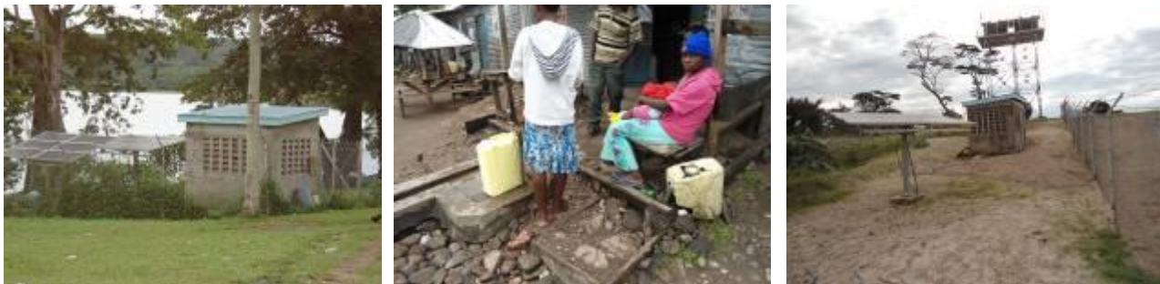
(Left) Solar powered water station and (Centre) one of the public taps in Mulabana. (Right) Water station in Kasekulo with two suspended 10,000 litre tanks
