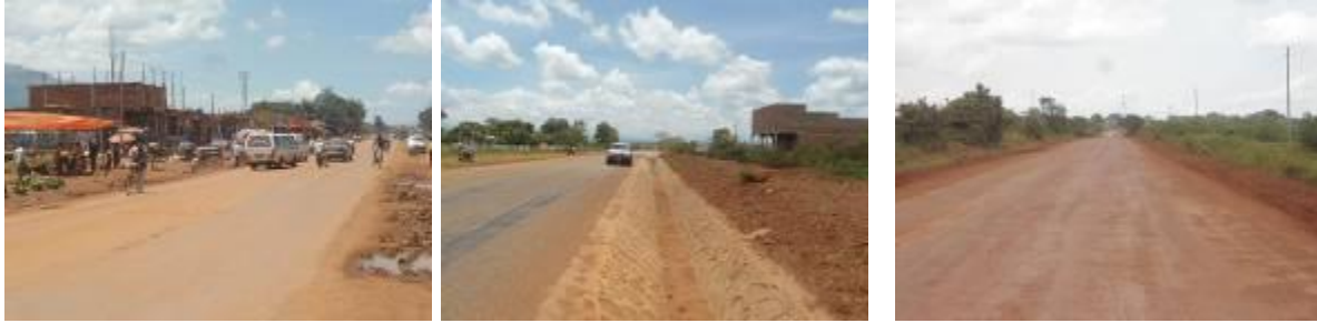
(Left); Temporary surface dressing works towards Mbale town at Km 2+600; (Centre); Drainage works near Bukedea town at Km 34+200; (Right); Scarified and maintained section to be considered as part of pavement works (sub grade).
