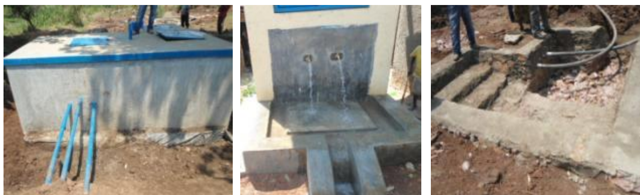
From left; a reservoir tank, a public stand post and a spring being constructed for people at the source
