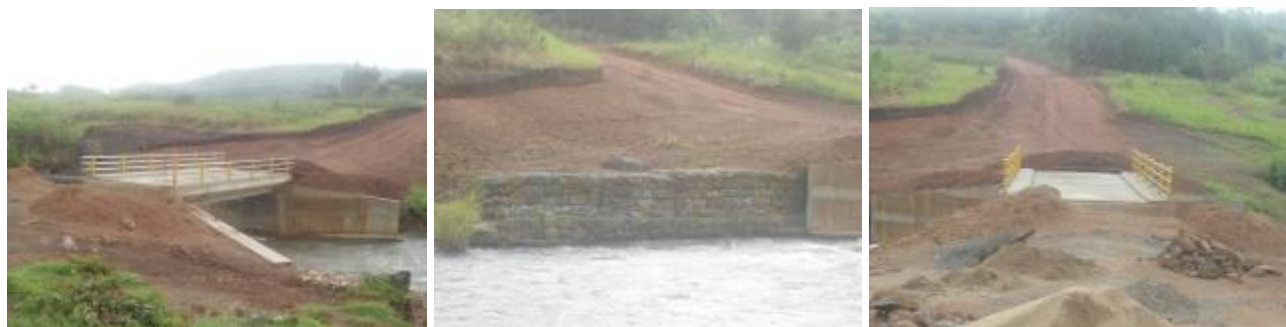
(Left): Completed abutments, decking and guard rails installed; (Centre): Gabion works at Jang Okoro side; (Right): Approaches to the bridge that are not yet completed on either side..
