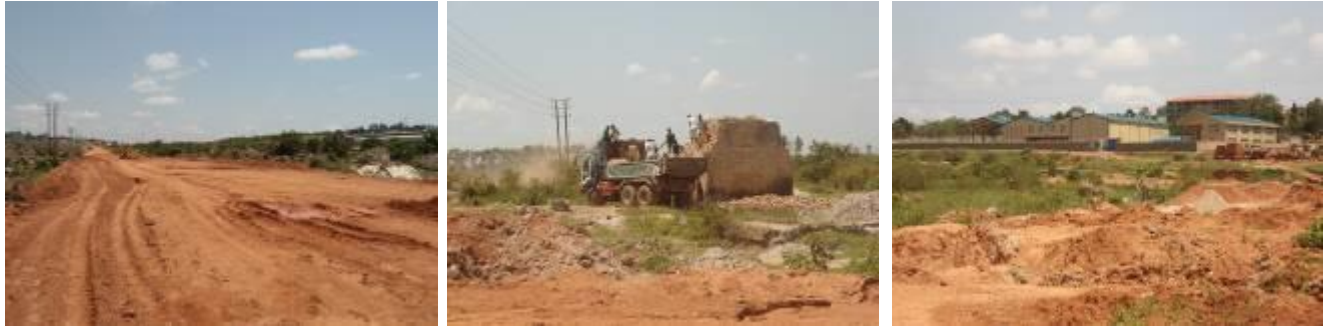
Earth works on the 2.5km road, brick makers removing their materials and completed Victoria seeds factory
