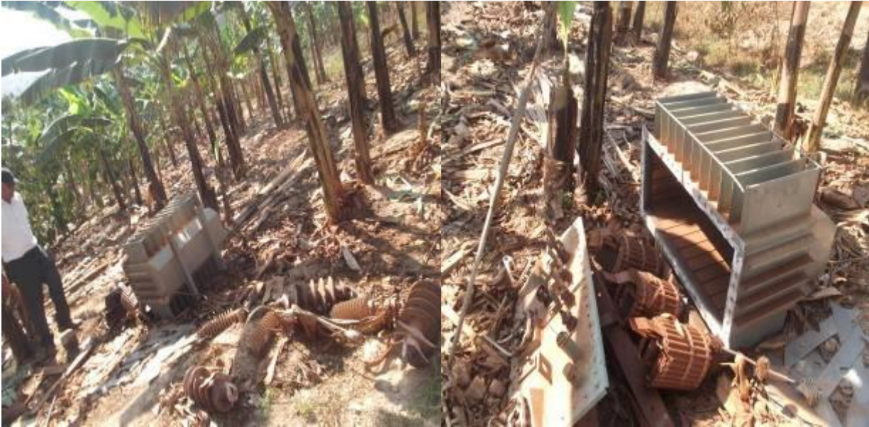
Vandalism of transformers on Lyantonde-Lumbugu line
