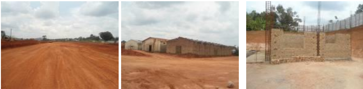
(Left); Pavement works in the yard for loading, off loading and storing containers; (Centre):Mukono district warehouses that will be demolished; (Right); ; Workshop at 15% progress.
