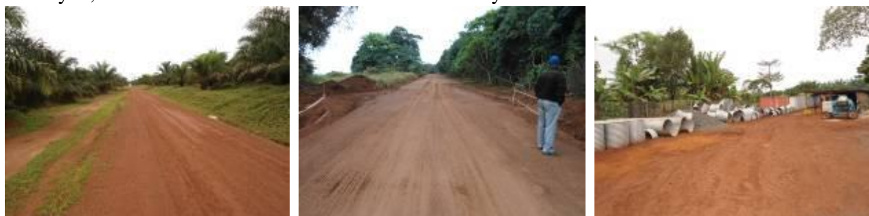
Section of the road reserve with palm trees, filled area at KM 39 and materials at camp site in Bwendero
