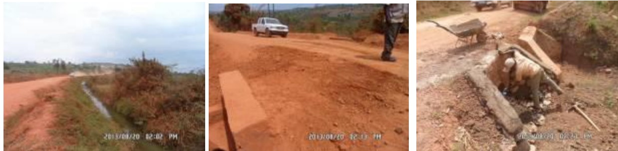
(Left): Catch water drain along the road in a raised section at Km 9+200; (centre); Replaced culvert crossing at Km 13+300; (right) Construction of head wall at Km 24+800.
