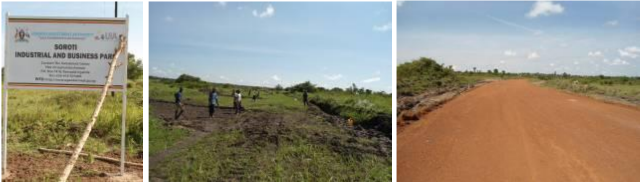
UIA signage, laborer removing top soil at Km 0.700 and graveled section of palm close
