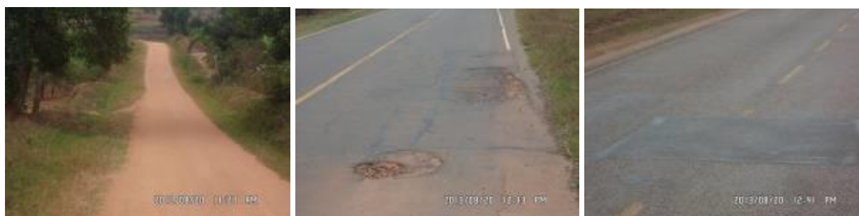
(Left): Graded section of Masaka-Kida-Dimo road at Km 20+600; (centre); Failed section on Masaka-Kyotera road at KM 48+900 on a side of the road that is heavily trafficked; (right) Patch works along Kyotera-Rakai road at Km 7+100.
