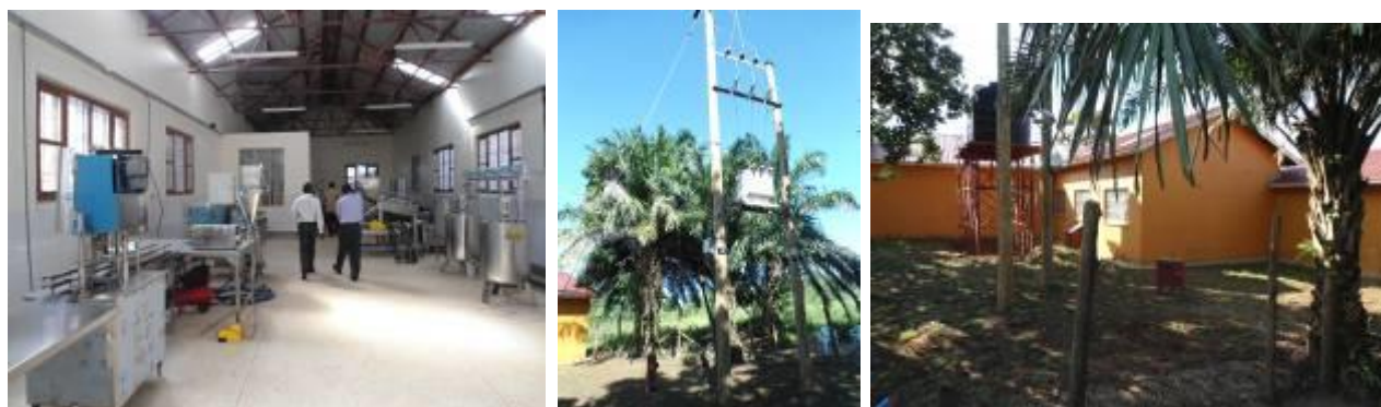
Delivered and installed equipment, single phase transformer and grassed compound besides the factory in Arua
