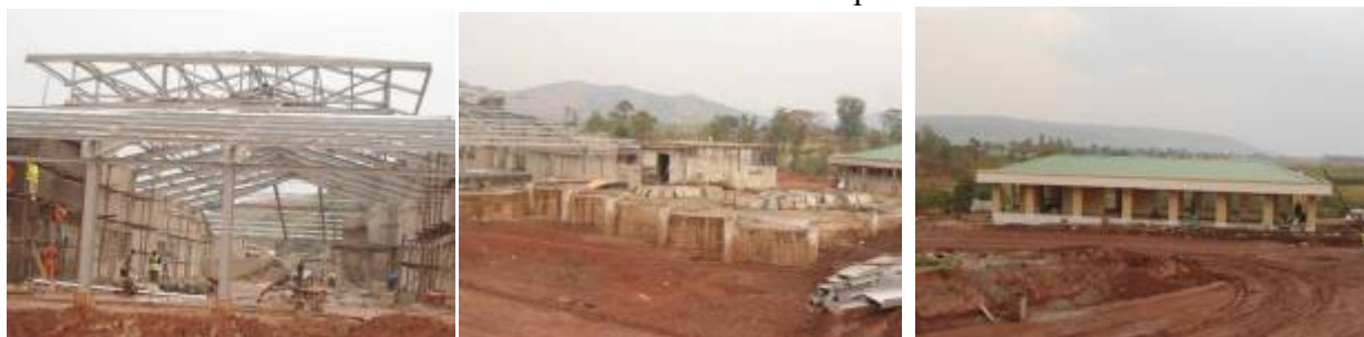
Mirama hills: Ongoing construction of the Customs and Immigration Block roof works(Left); The substructure of the verification at the floor level(Centre); The access road works and the clearing agents' office block(Right).
