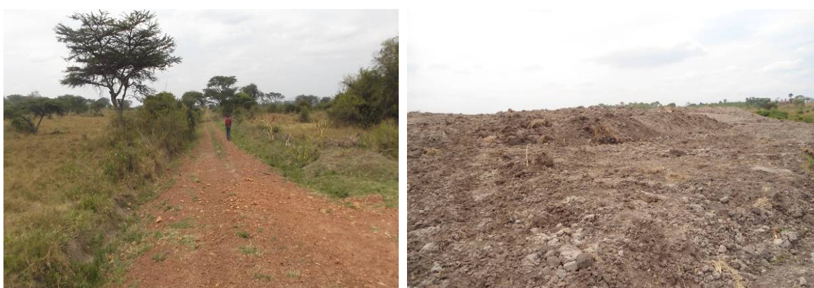
Left to Right: opened access road with murrum/stones not compacted and volume of uncompact soil materials around the valley tank and the fish pond at Mbazardi
