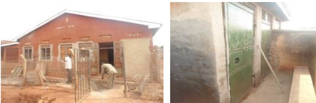
Renovation works at Mutai HCII and right is the replaced doors on the toilet
