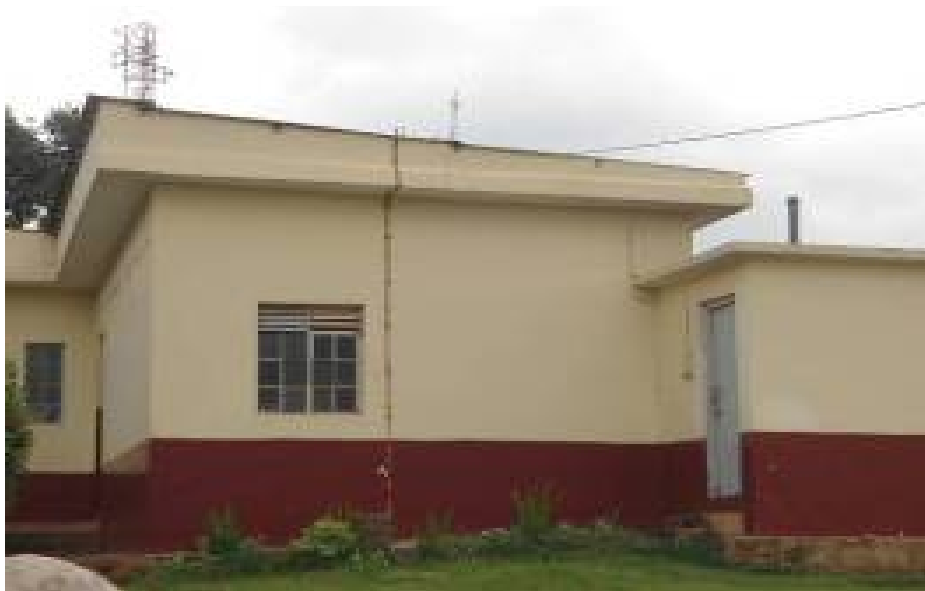
A lightning conductors installed on one of the blocks at East Kololo P/S
