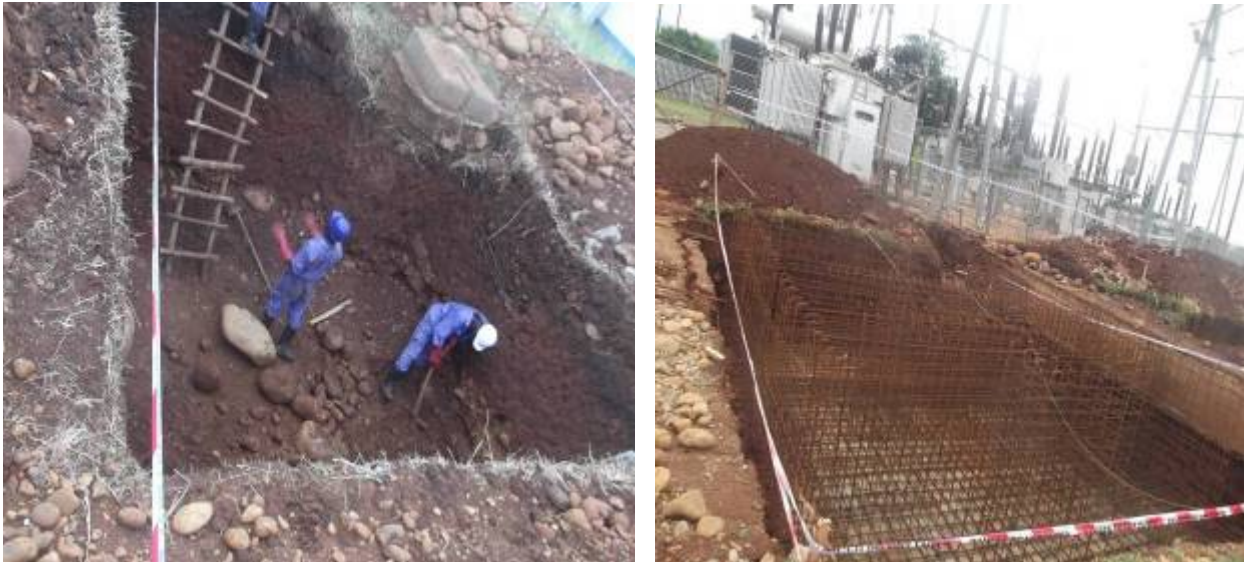
Left: Manual Excavations of hard rock Right: Preparatory works for concrete casting on Nkenda substation
