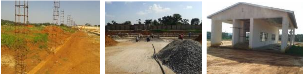
Mukono ICD; Left: An incomplete section of the boundary wall; Centre: Ongoing construction of the Container Stack Platform; Right: Weigh bridge house
