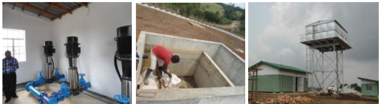
L-R: Installed water pumps, and a worker filling the sand filter at Kyamugambira; Elevated water tank and completed pump house in the background at Nyaruzinga hill, Bushenyi district
