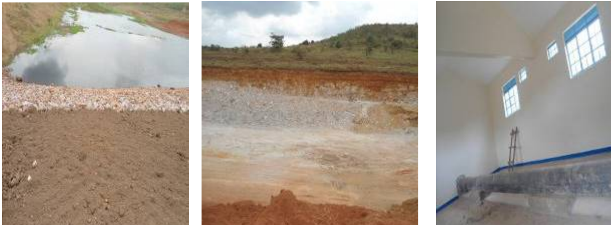
Left to right: Laying the gabion mattress, excavation works for the spillway, and an installed water pipe outlet at Kagamba sub county, Rakai district
