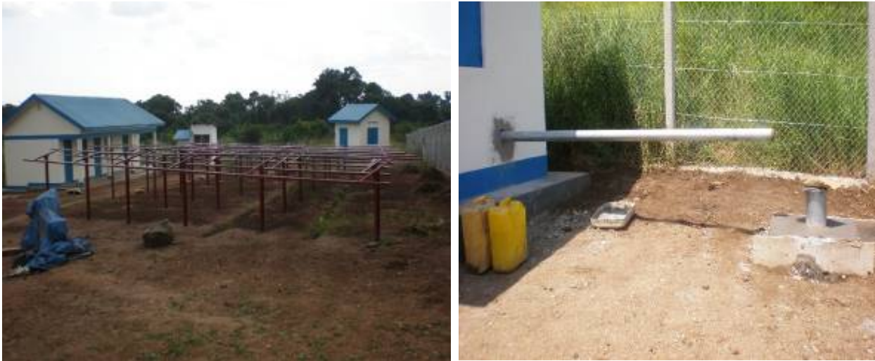
Left to right: Installed solar arrays for solar panels, a completed water office, guard house, and an eco-san toilet. Unconnected pipe from pump house to production well at Wadelai sub-county, Nebbi district
