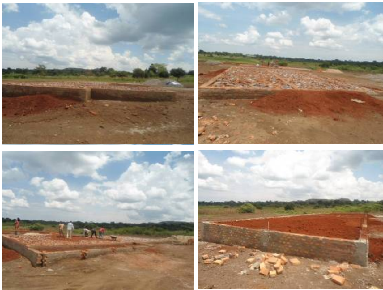
Some of the structures under construction at Engineer Kauliza Kasandha Technical Institute
