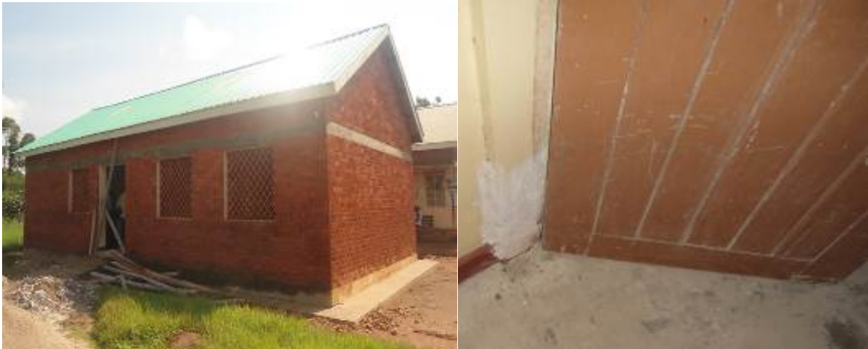
Left: Renovation works of the OPD and Right is the old door frame filled with FILA instead of replacement at Budima HCIII in Jinja District
