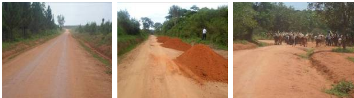
Left: Completed section of Katugo – Kinyogoga-Kaweweta at km 24+600, Centre: Gravel dumped along Katikamu-Bamugolodde-Nakasongola road at km 73+200, Right: Cattle along moving Katugo – Kinyogoga-Kaweweta road
