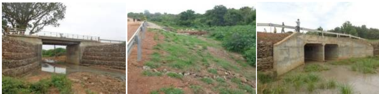
Arua-Yumbe-Wandi road, (Left): Completed Daca Bridge, 54km from Wandi road; (Centre): Grass planted along the embankment of the approach road on Ure Bridge; (Right): Completed Eventre Box Culvert, 34km from Wandi.
