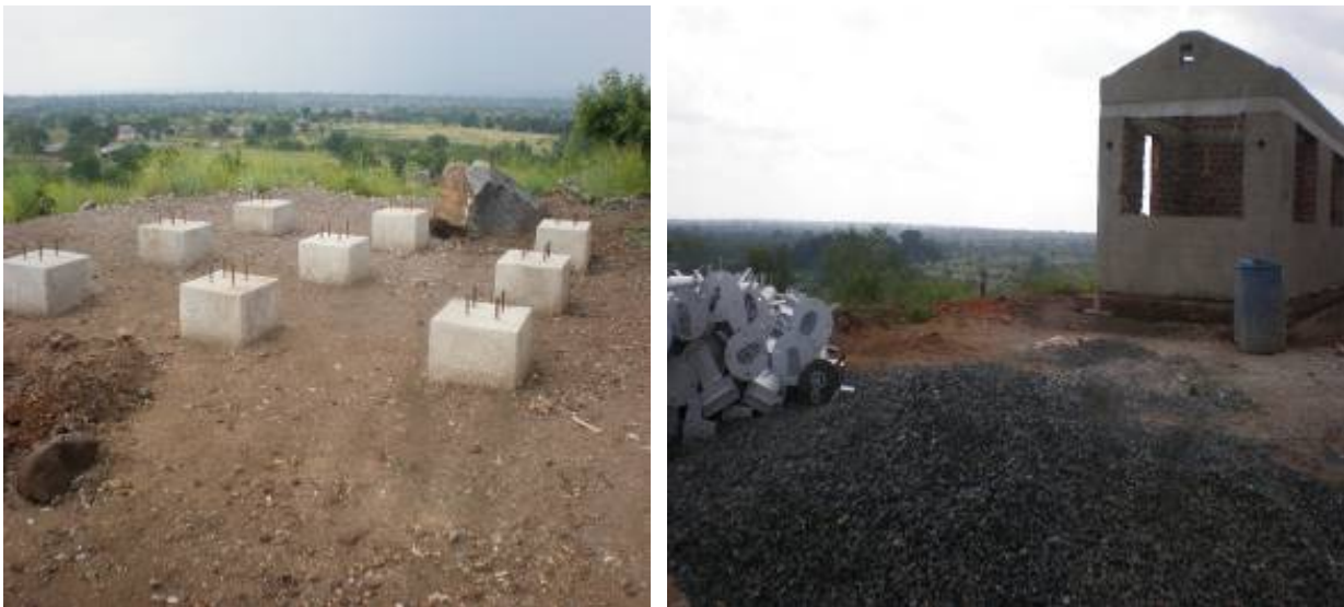
Left to right: constructed reservoir base for installation of a 130m 3 tank, materials for completing the chlorine dosing house at Wadelai sub-county, Nebbi district
