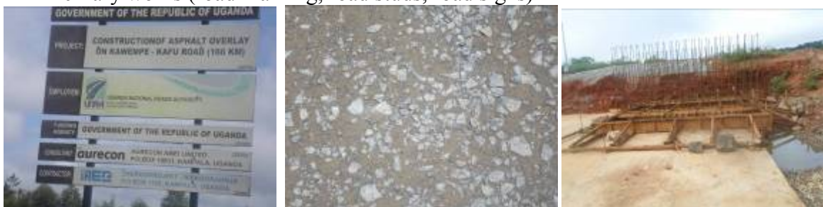
Left: A project signboard at km 166+000; Centre: A rejected section of roadbase at km 175+000; Right: A box culvert under construction at km 41+000 on Kawempe–Kafu-Kiryandongo road
