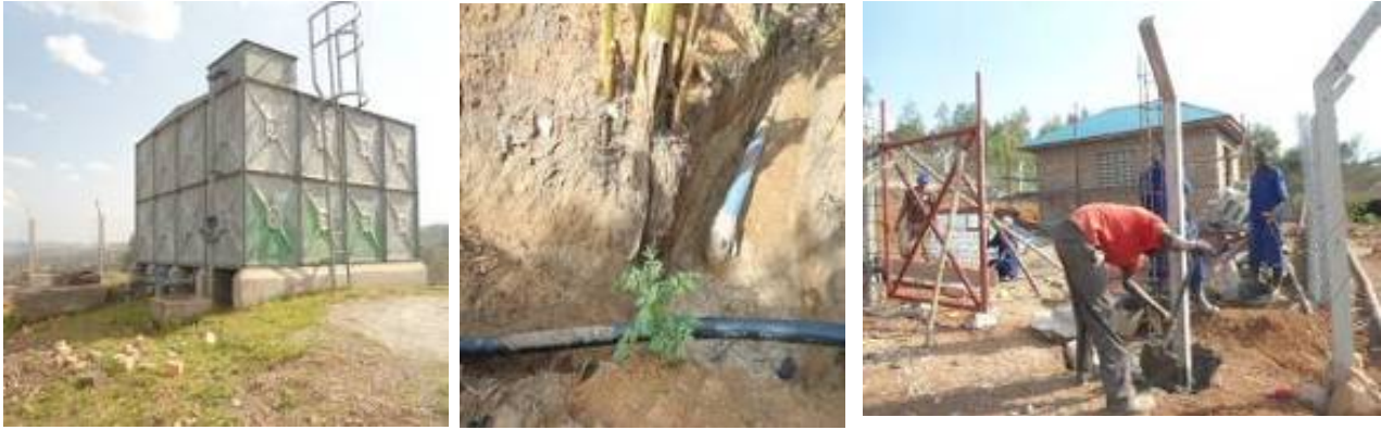
Left to Right: A rehabilitated reservoir tank at Nyabubare, laying of the distribution lines, and Construction of a Kikoni booster station.
