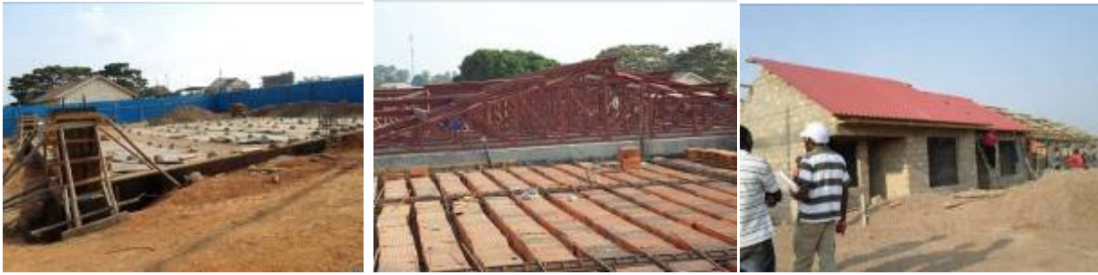
Left: light weight inspection site at foundation level; Centre: Ongoing roof works at the freight building; Right: Ongoing roof works at staff quarters at Mutukula OSBP
