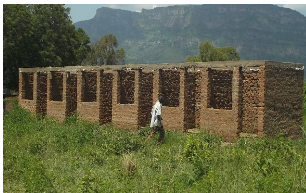
Meat stores that were constructed up to the ring beam in Iriiri Sub County
