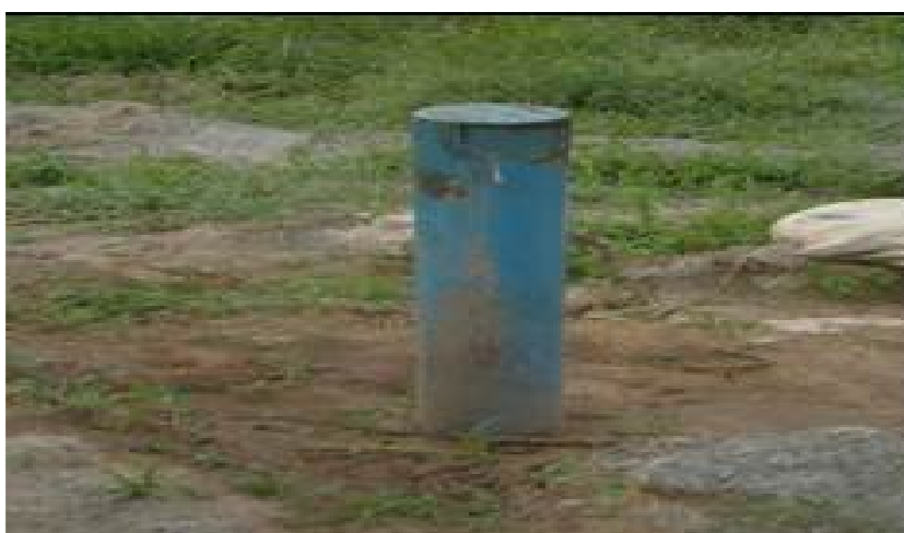
An installed production well of capacity 5m 3 /hr after the design changes in Muduuma town, Mpigi district
