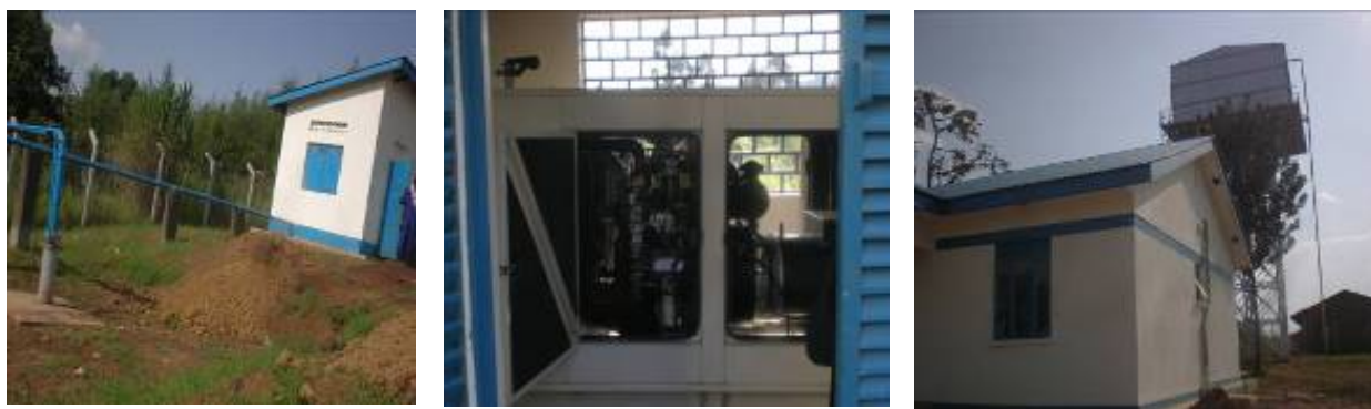
Left to right: Installed production well, pump house, Generator, Office block and water reservoir in Paidha town
