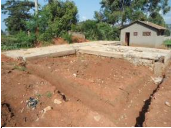
Construction of a toilet at St Paul Demonstration School Ggaba that stalled at ground slab level
