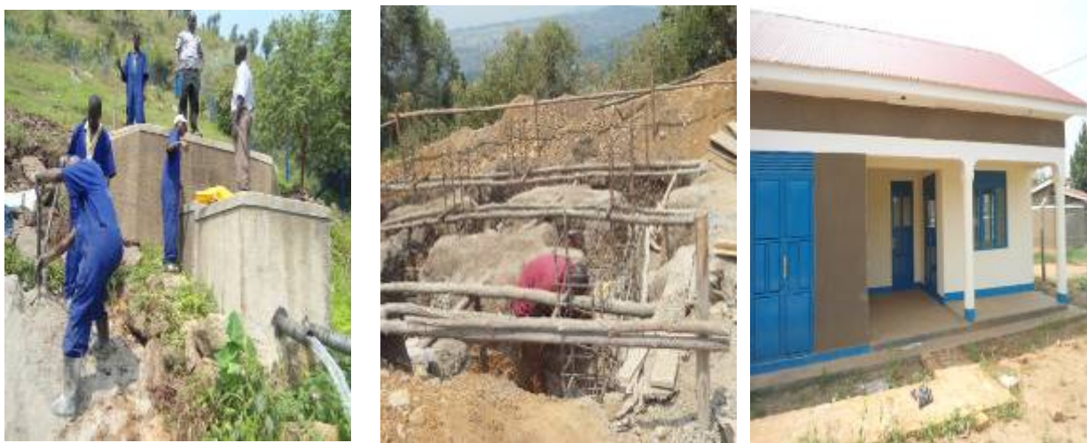
Left to right: trenching works around the 2 nd protected spring to control erosion, construction of a 170m 3 /hr reservoir tank at Kanyantorogo, and a completed office block in Kihiki sub-county
