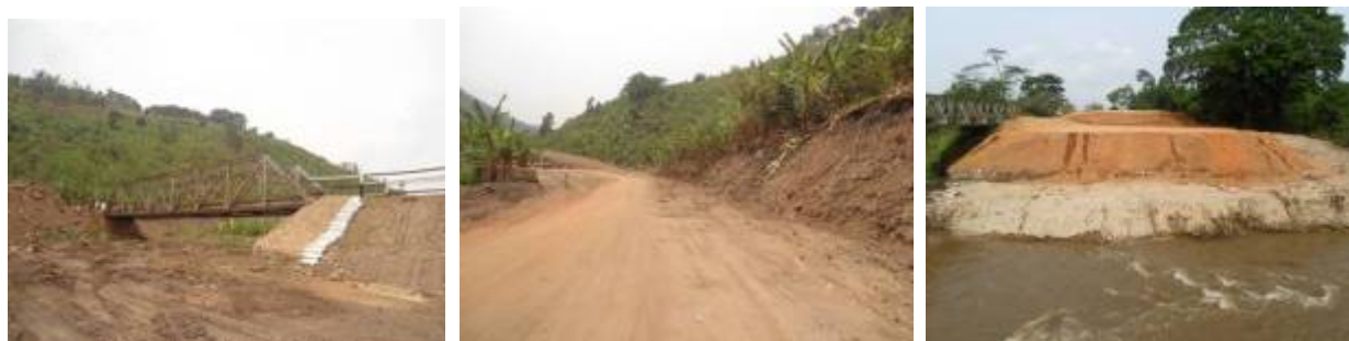
Left: The temporary access restored on Mitaano bridge; Centre: Cleared approach on the Rukungiri side of the bridge on Mitaano bridge; Right: Embankment build up on Ntungwe Bridge
