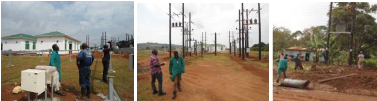
L-R: completed power house and solar panel frames in foreground, and installation of substation Works at Bukuzindu Right: Transformer wiring at Kagulube
