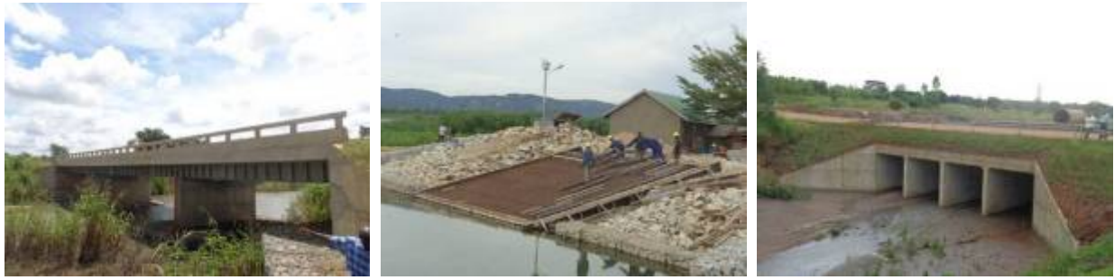
Left: A completed 3-Span Ayugi bridge at Km 13+800; Centre: Works ongoing on the spillway at Umi landing site at Km 65+442; Right: A completed 4-cell box culvert where river training took place along Atiak-Moyo-Afoji Road
