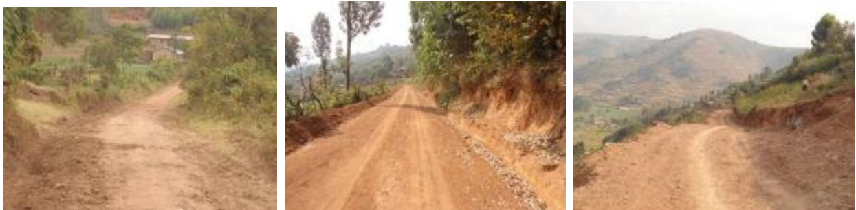
Kabale District: Left: Slashed grass along the road side of the emergency road, Nyakanengo-Nyakasiru (9 km); Center: A section of Lake Bunyonyi-Kashambya (7.5 Km) graded in June 2014; Right: An opened up section of the Kyenyi-Rutoga-Muko HCIV access road
