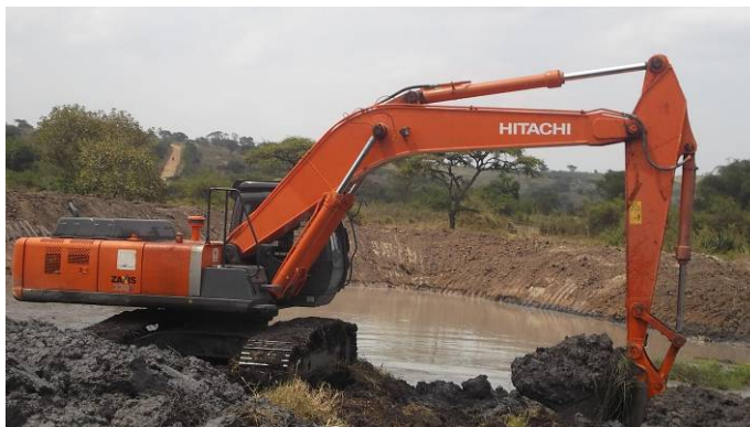
Excavation of a Valley tank ongoing at Lwakabyambi farm in Kikatsi Sub County
