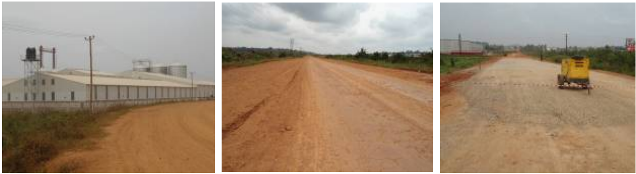
L-R: Completed Kyagalanyi coffee factory; newly opened road to North Estate by MoWT, and ongoing paving of 4 km in Namanve South Estate by UNRA
