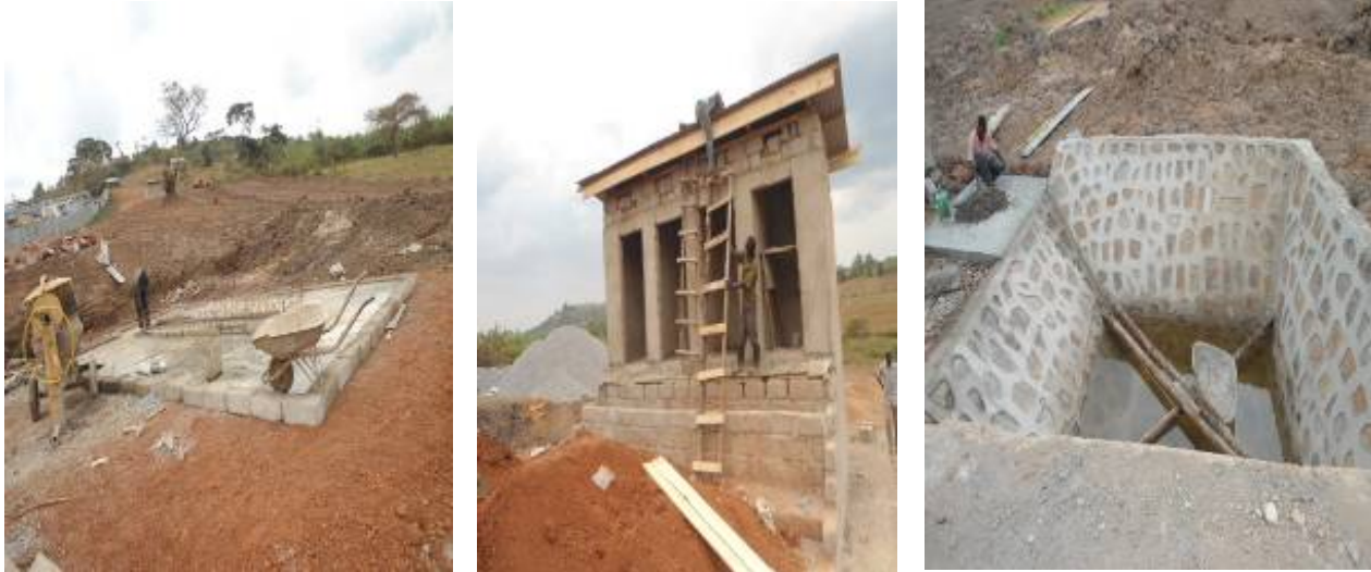
Left to right: Construction of cattle trough, an eco-san demonstration toilet, and a valve chamber at Kagamba sub county, Rakai district.
