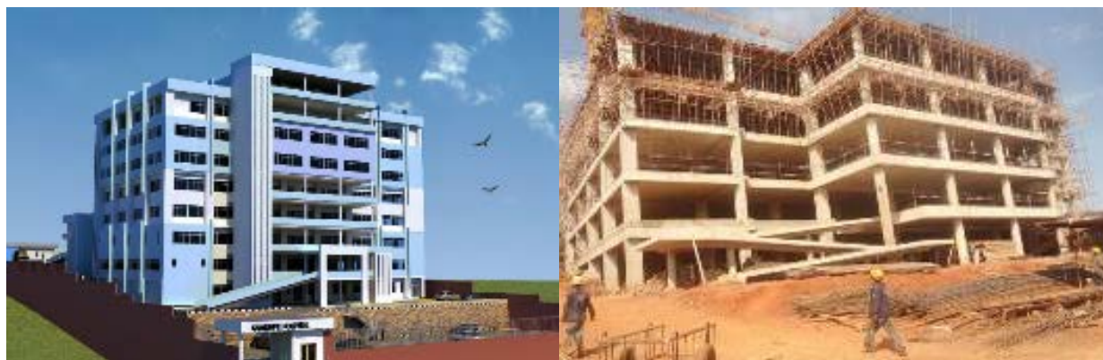
Left: Artistic impression of proposed Kawempe General Hospital. Right: Ongoing works on the main hospital block
