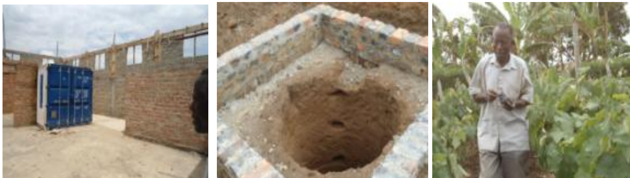
Left: Incomplete expanded structure covering the original containerized winery Centre: Excavated Pit latrine, Right: Incubatee in the grape yard
