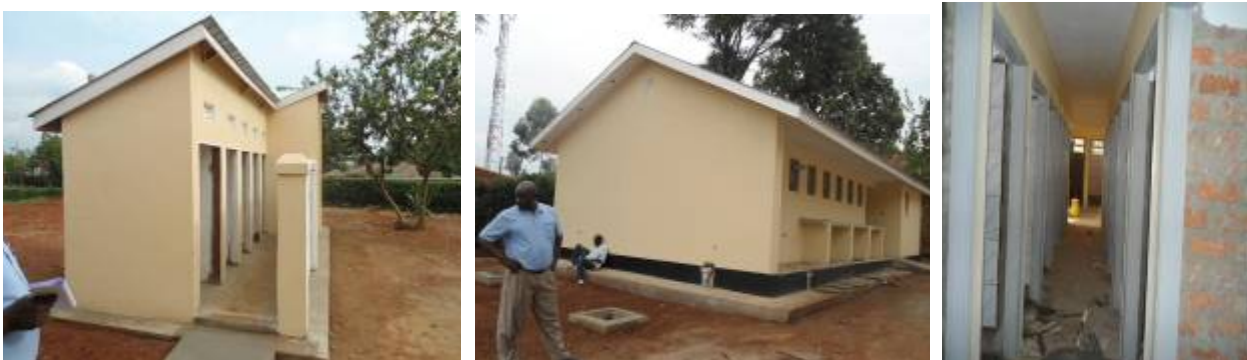
Left: the six stance lined VIP pit latrines at finishes level, Center: the girls' bathroom at finishes level and right: progress inside the bathrooms Ibanda PTC
