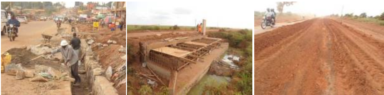
Left: Road side drain stone pitching works in Namakwekwe at Km 2+473; Centre: Extension of a box culvert at Km83+553; Right: Modification of the existing road to form sub-base at Km 95+888 for Mbale-Soroti section.
