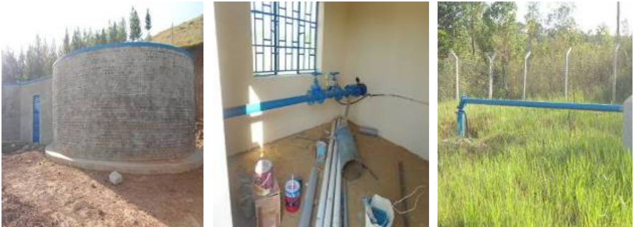
Left to right: Concrete twin reservoir tank (150m 3 ), pump control valves and, an installed production well
