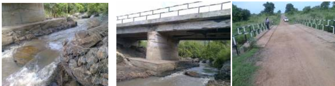
Left: Incomplete gabion works; Centre: Front view of the bridge; Right: Bridge deck and pier on Alla 2 Bridge
