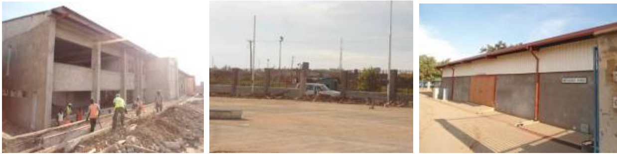
Left: Storm water drainage works around the main administration building; Centre: the rehabilitated impound shed; Right: Part of the fencing and parking yard at Malaba OSBP
