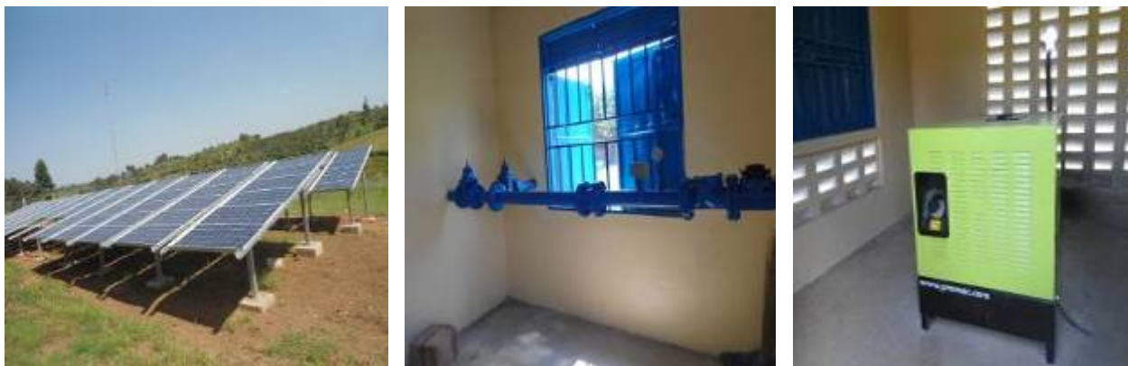
Left to right: Installed solar panels to support the system, submersible pumps, and a generator
