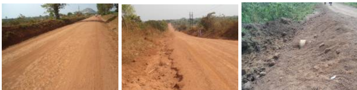
(Left): Section of Ngetta-Apala-Adwari road (4+600 km) that was re-gravelled; (Centre): An eroded and silted drain at Km 10+400; (Right): A newly installed culvert line without a headwall along Kotido-Aduku road at km 21+800
