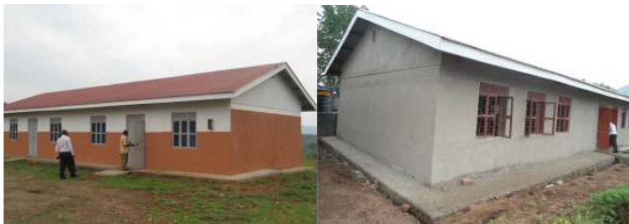
Left: A completed two unit teachers' house completed, Right: a two classroom block at finishes level at Kamwenge S.S
