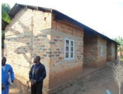
The staff house at Rukole C/P which is supposed to be completed with the funds that the C/P received
