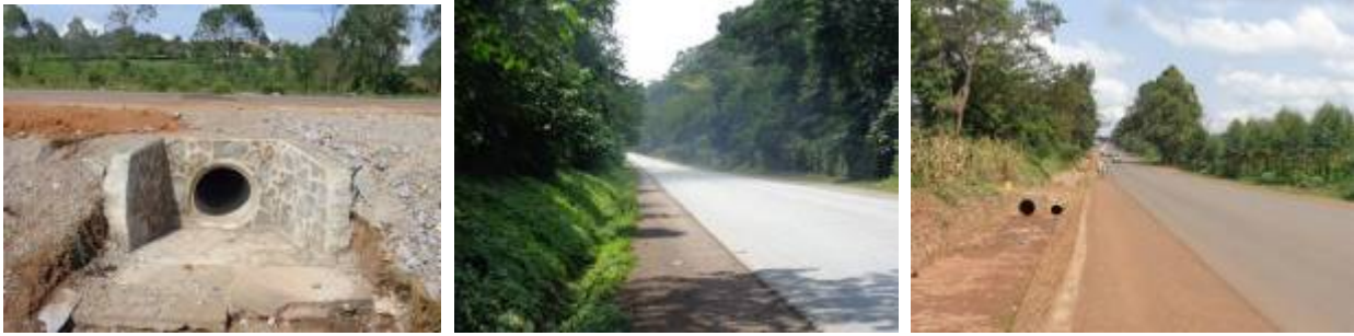
Left: 900mm drainage culvert; Centre: A completed section in Mabira forest with a narrow trapezoidal side drain at Km33+000; Right: A raised section with a stone pitched side drain between Km 52-53 for Mukono-Jinja Road
