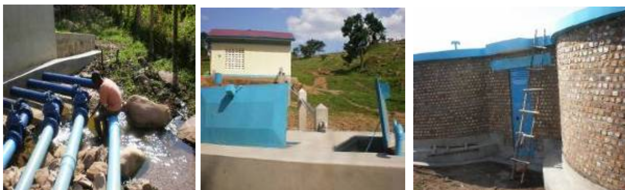
Left to right: Protected spring eyes with a boy tapping water from the pipes, collection water tank from the spring, a guard house, and a twin concrete reservoir tank of capacity 150m 3
