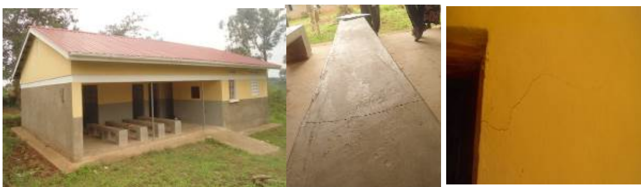
Left: Completed OPD, cracked patient bench (middle) and cracked wall in the new OPD at Kashongi HCIII (Right)
