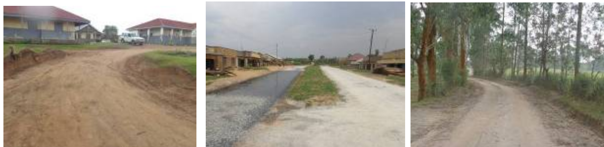
Bushenyi-Ishaka Municipality: Left; The graded and gravelled Access road to the Health Centre IV; (centre): Nyakabirizi Dual Carriage undergoing sealing works; Right: A graded section of Katungu –Nyamigo road
