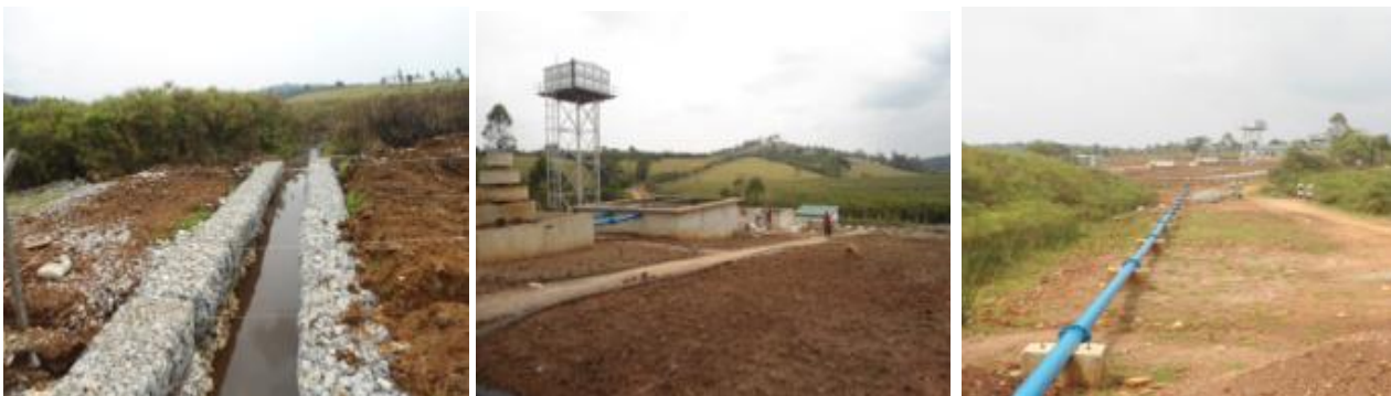
L-R: Gabion lined inlet channel, completed water treatment system and transmission pipe at Kyamugambira
