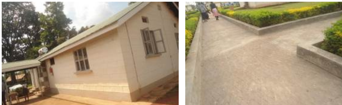
Renovated Interns mess (left) and newly constructed walk ways on the (right)
