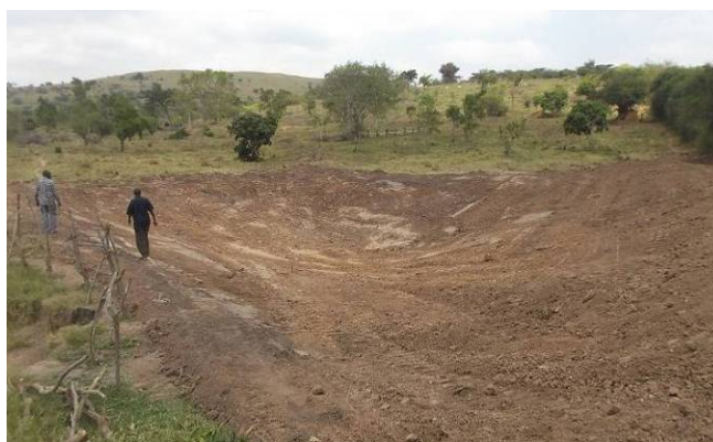
Kyataano valley tank excavated and completed at Ruhengyere field station in Kiruhura district
