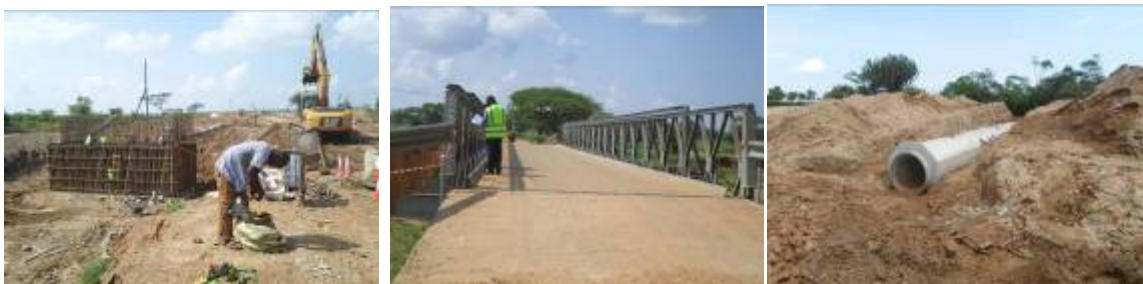
Left: Form work fixing on the new bridge at Nadunget [km 86+000]; Centre: An existing bridge at Nadunget which was to be demolished; Right: A laid pipe culvert of 900mm diameter at km 34+400 on Nakapiripirit-Moroto road
