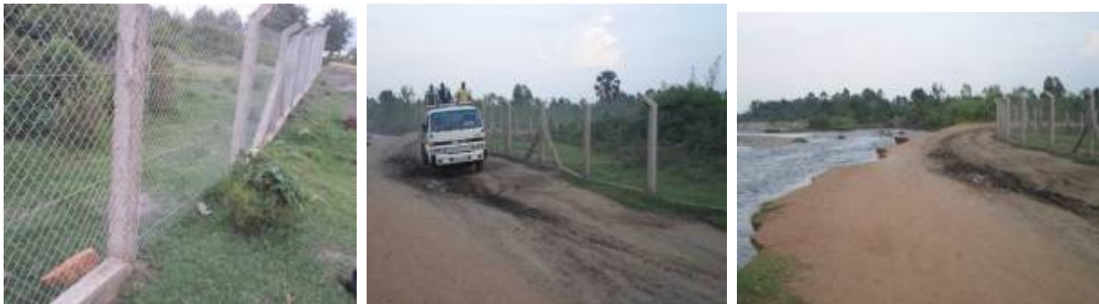
Kasese Airfield: Part of the completed perimeter chain link (left); part of the newly constructed community access road (Centre); Part of the community access road that was being destroyed by the floods (Right)
