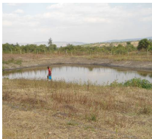
A valley tank excavated at Mr. Batisibwa's farm in Macha sub County
