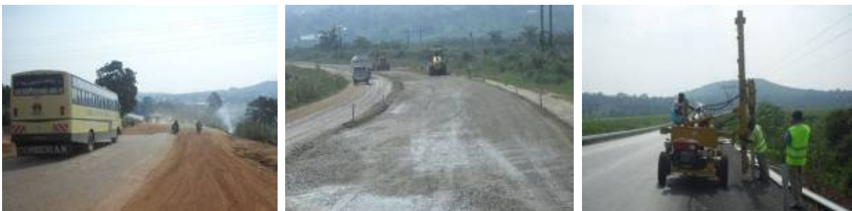
Left: A section at Maya where works had not been executed due to unsettled land acquisition issues; Centre: Base course works in the swamp at Km 20+000; Right: Installation of guard rails at Km 25+390 on Kampala-Masaka phase II
