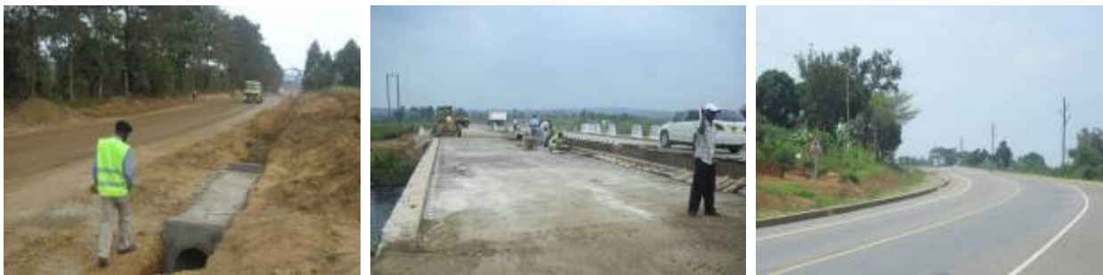
Kampala-Masaka phase II: Base course works and drainage works along the Nkozi link (Left); Parapet wall works ongoing on the New Katonga Bridge(Centre); A completed section of the road in Section 2 (Right)
