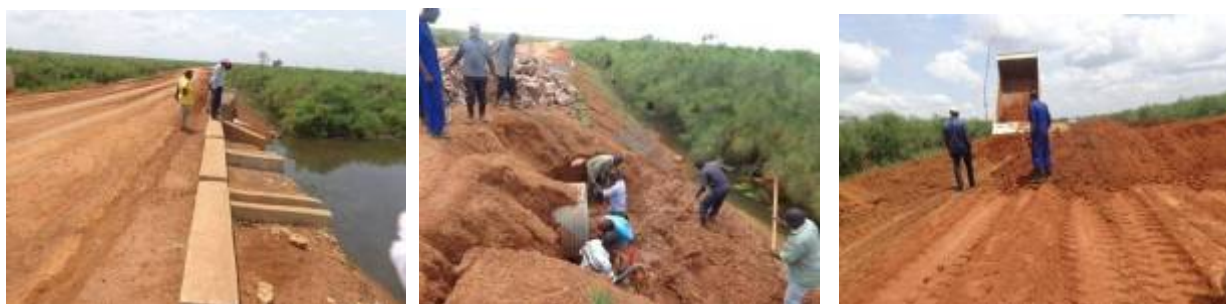
Left: A completed section of the swamp crossing; Centre: Excavation works for the culvert headwall construction; Right: Embankment filling on Saaka swamp
