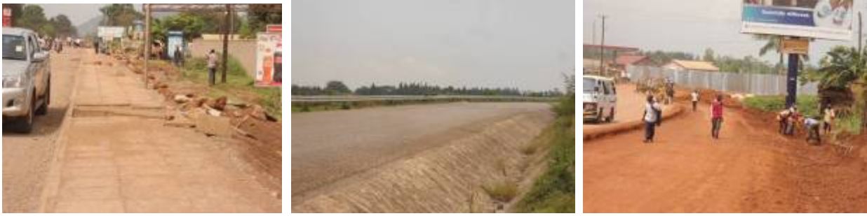
Left: Ongoing ancillary works of the pedestrian walkway at Km 3+425 in Tororo Municipality; Centre: Completed section at Km32+237 with a stoned pitched side drain and guard railing; Right: Road side embankment preparation in Mbale Town at km 47+650 for Tororo-Mbale section
