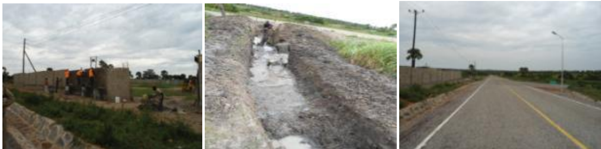
Left: Ongoing works on the fence, Centre: Foundation works for the fence, Right: Completed road in Soroti
