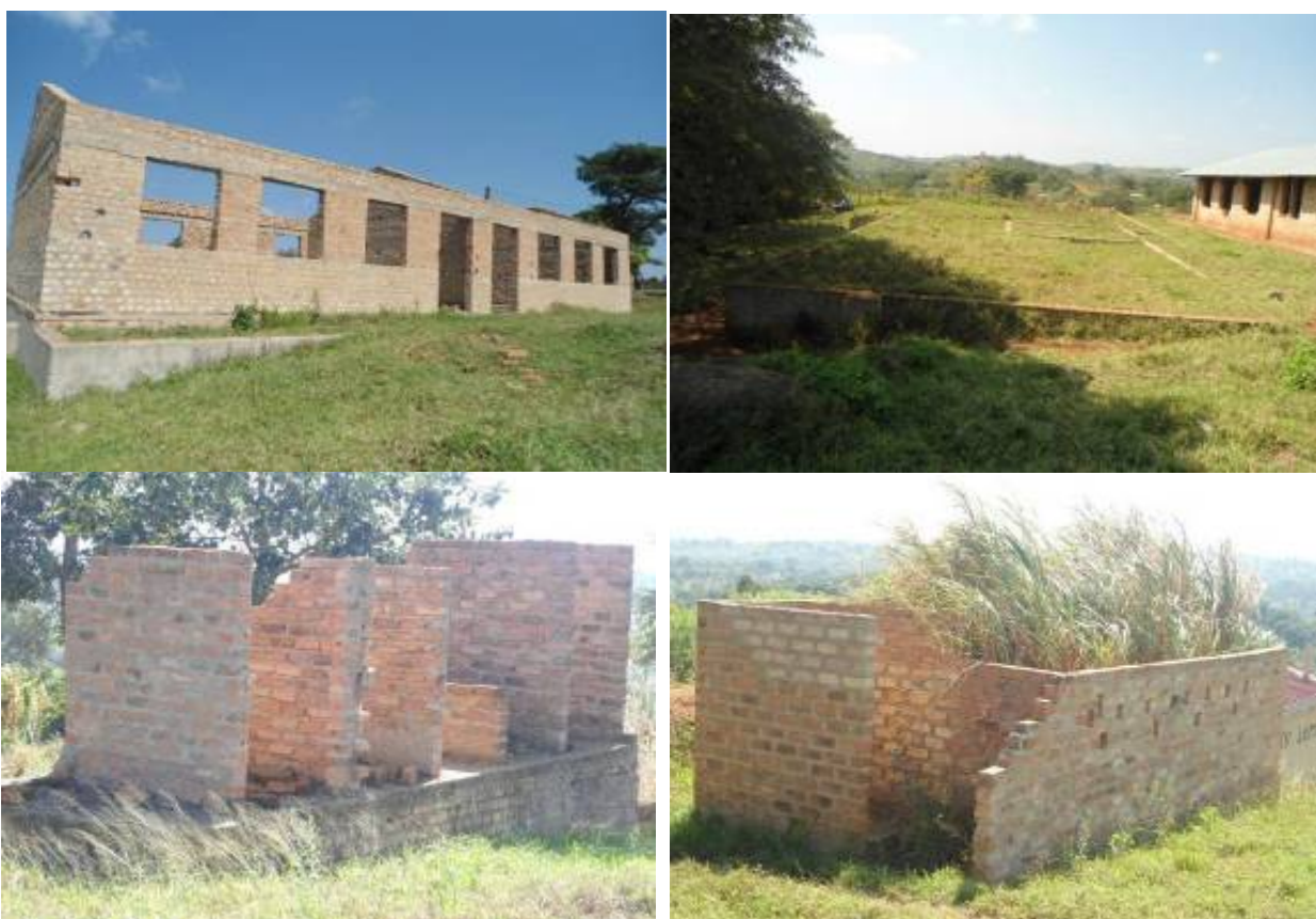
Clockwise: The incomplete two classroom block, the stalled multi-purpose laboratory and two blocks of VIP latrines at Kasule Seed S.S.
