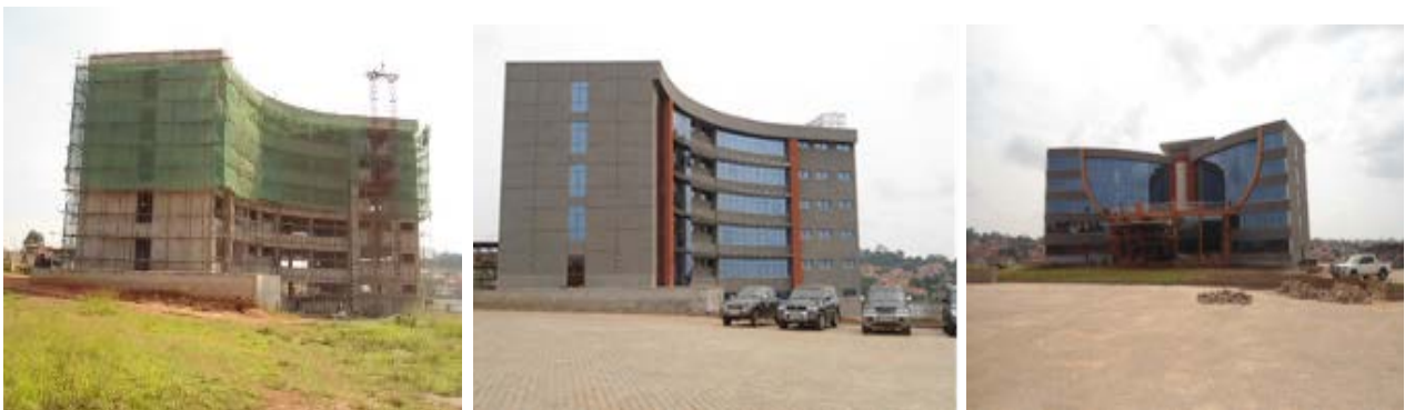
Left: Completed Phase 1A in July 2013; Centre: Curtain walled structure and Right: front view of the building
