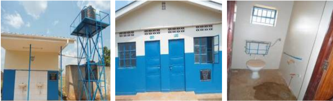
Left to right: A constructed toilet at a maternity ward at Mayuge Health Centre III, a water borne toilet at Mayuge Town Council, and at the taxi park
