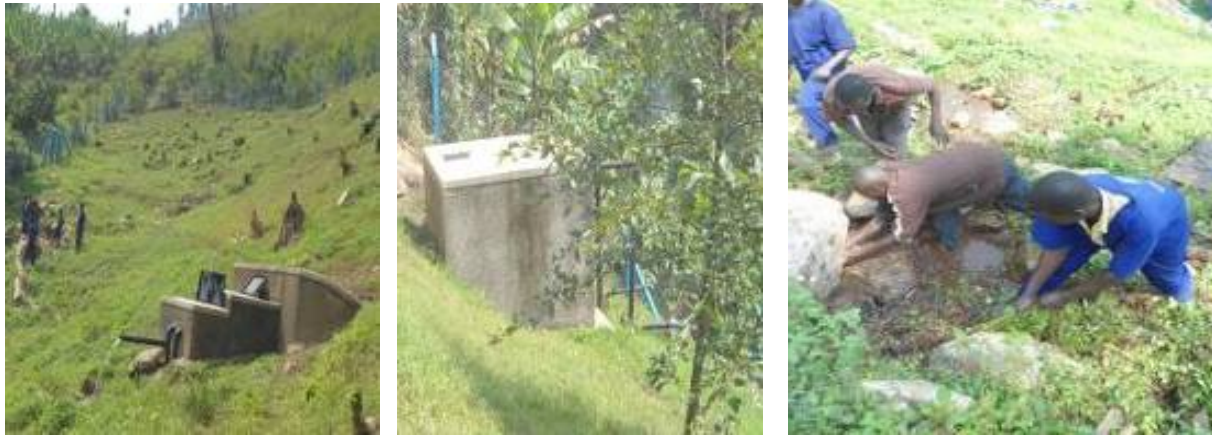
Left to right: A well-protected spring in Chumbugushu, a water collection tank for the protected springs at the source and works on a spring eye protection for community use
