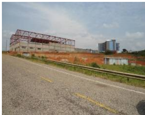
Construction of Crane paper industry and UNBS headquarters at Bweyogerere Industrial Estate
