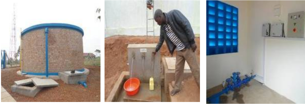
Left to right: A constructed reservoir tank, a functional public stand post, pump control valves and electrical control units in the pump house
