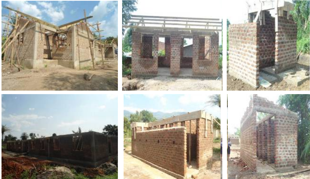
Top Left: Semi detached staff house at roofing level, outside kitchen at roofing level and a two stance VIP latrine, Bottom Left: Girls' dormitory at ring beam level, six stance VIP latrine at ring beam level and bathrooms at wall plate level at Bundibugyo PTC
