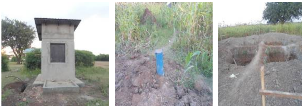
Left to right: A constructed kiosk in Ongino town, a drilled production well, and a foundation for erecting of a reservoir tank
