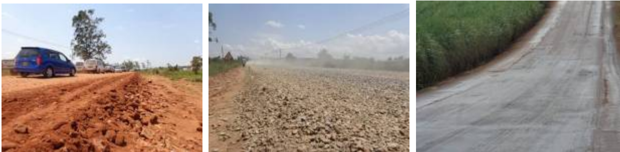
Left: Ongoing works, Mechanically modified base material that is to form a new sub-base; Centre: Crushed Run Rock for the base course works; Right: A milled CRR section at Km 45+500 for Mukono-Jinja Road
