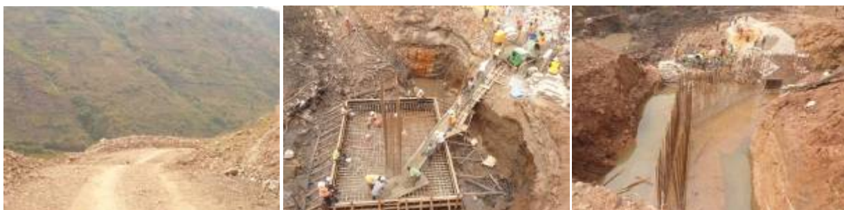
Left: An opened up section of the 2km approach road on the Kanungu side; Centre: Casting of concrete for the base of the pier; Right: Curing of the basement for one of the abutment walls on Birara bridge
