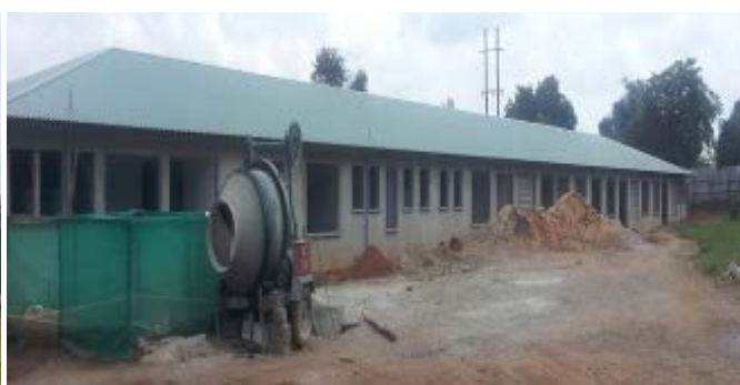
New T-Block with Wards, Theatre, offices and Mortuary under construction at Kiryandongo Hospital
