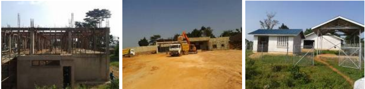
Left: An office block under construction; Centre: A Workshop/shed under construction; Right: Completed structures that will be housing the services (power and pump house; generator shed) equipment at Mukono ICD
