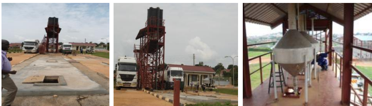
Left: Reconstructed tank with open manhole; Centre: verification of trucks and Left: Calibrated rig provers at Bweyogerere
