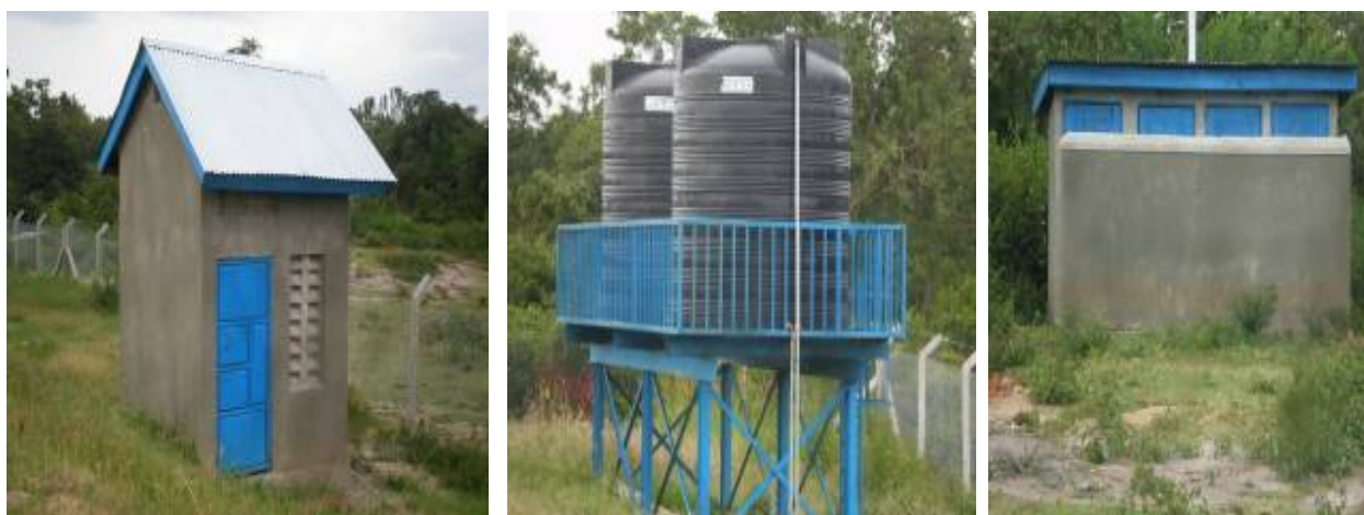
Left to right; a completed pump house, installed HDPE tanks of capacity 10m 3 , and a 4-stance VIP latrine
