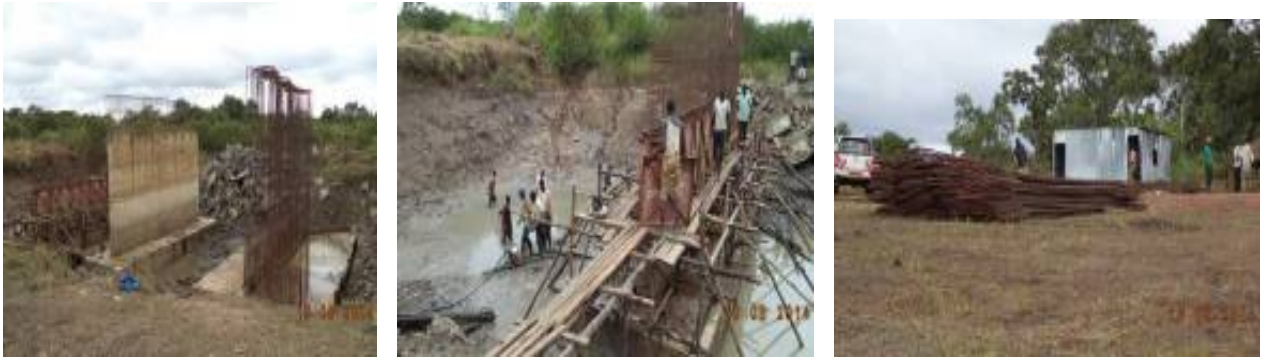
Left: A completed centre bridge pier; Centre: Steel fixing, dewatering and formwork for the abutment; Right: Steel on site for Kaguta Bridge.
