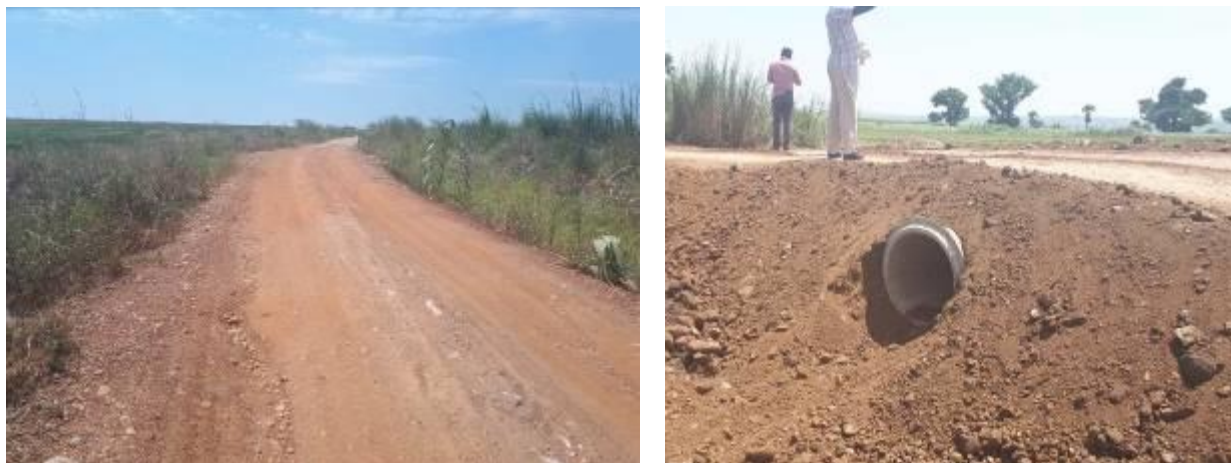
A graded section (left) and an incomplete culvert installation (right) along Anaka-Amuru road (29km)
