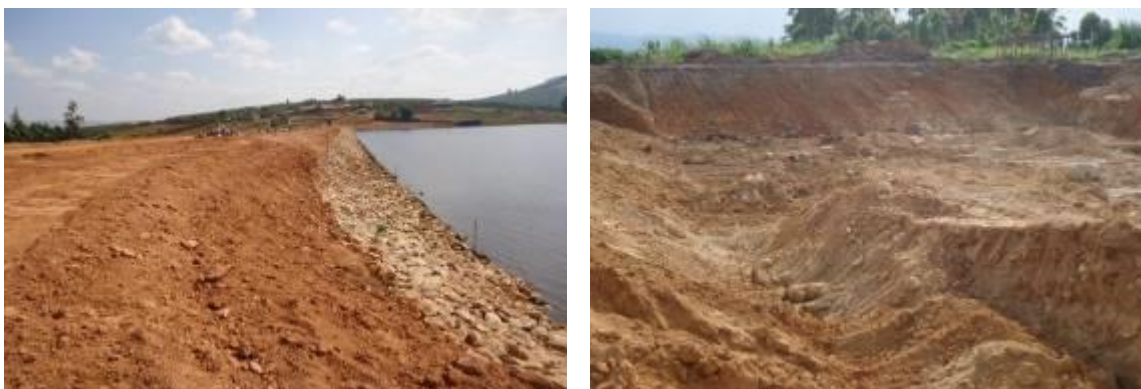
L-R: A section of Mabira dam showing riprap construction and the embankment in Mbarara district; Excavation works of reservoir tank 2 for Rwengaju irrigation scheme on Cossy Hill in Fortportal, Kabarole District
