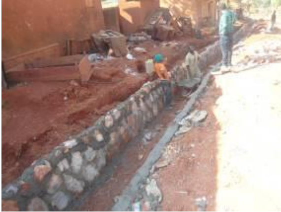
Drainage works of stone pitching on one of the access roads of Busabala - Kaazi Road at Km 1+700
