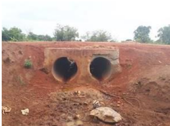
A two cell concrete encased 900mm diameter culvert installed on Lapul-Atanga Road
