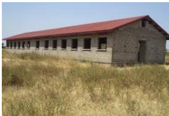
Girls' dormitory at Lolachat Primary School in Nakapiripirit district as at December 2017
