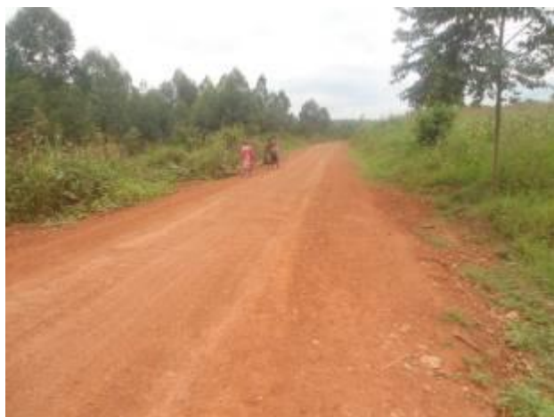
Kansiri-Kalyankoko-Kibaaga (9.1km) in Luweero: A well graded and graveled section at km 6+500
