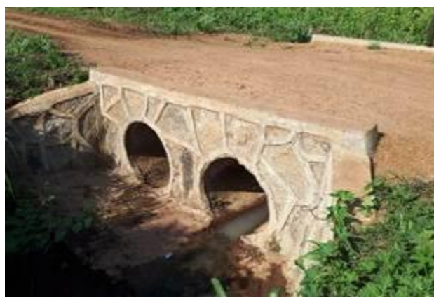
2lines of 900mm diameter culverts installed on Lurujo-Nyai road (14.4km) under RMeM in Q3
