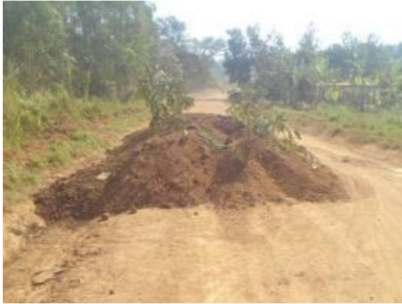
A heap of dumped gravel for correcting snag section on Lusailira-Nkonge road
