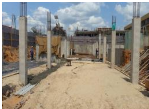
Basement ground floor columns and shear wall cast in progress at Mbarara Central Market site
