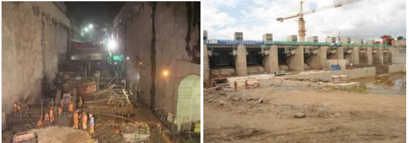
L-R: Unit 1-6 Installation works in the Power House; Installed radial gates at the spill way
