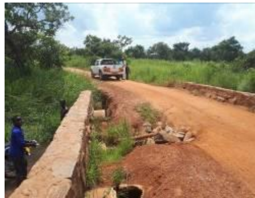
A culvert crossing on Labora-Loya-Ajonga road(29.9km) which was washed away by heavy volume of runoff
