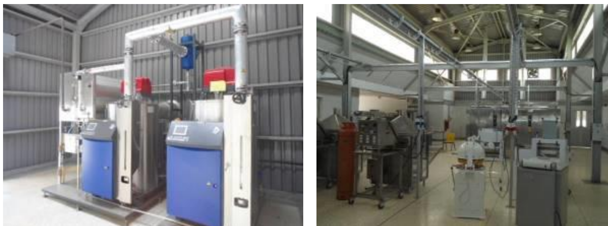
Steam boiler equipment and bakery equipment installed at PIBID Bushenyi
