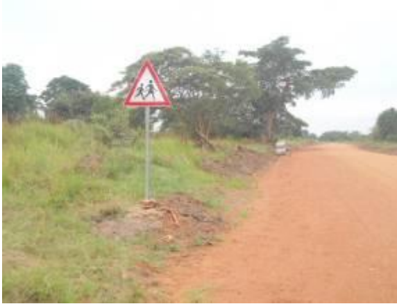
Installed road signage at km 38+200 on Ihungu-Bulyamusenyu road
