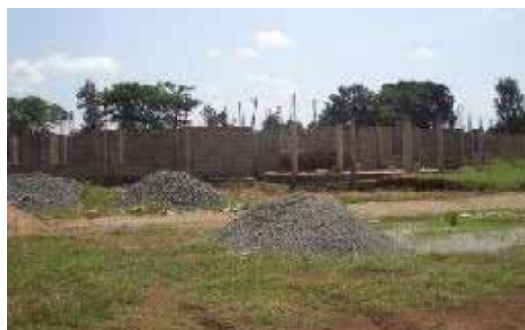
Raising of columns on new administrative block in Bulambuli District in July 2019
