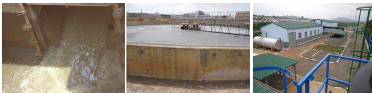
L-R: Sewerage collection point; Sedimentation tank; at Bugolobi; and completed structures of the Kinawataka pretreatment in Luzira all in Kampala District
