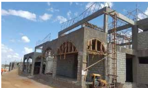
Rare elevation with roof trusses raised up and fixed at Lopeduru main market, Moroto Municipal at in July 2019
