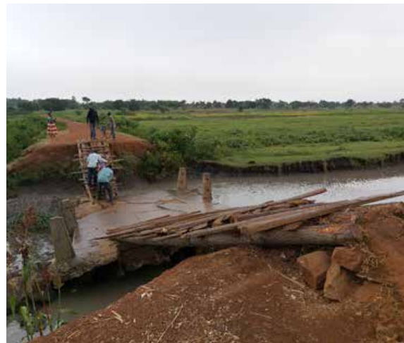
Koboleki bridge that was washed away by a flood. The bridge connects Bukedea district and Butebo District
