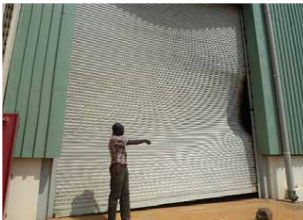
One of the damaged access doors at the cotton seed dressing plant in Pader District
