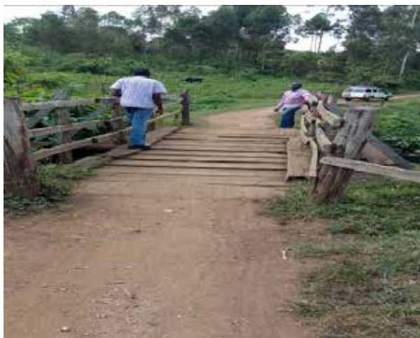
A dilapidated bridge on Kicucu-Lamabwa-Kasura Road at 2+200
