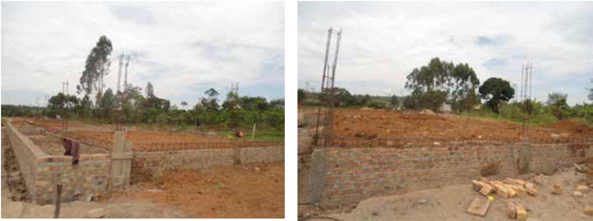
L-R: Ongoing works for construction of Mbirizi Seed Secondary School under the UGIFT Project in Lwengo District
