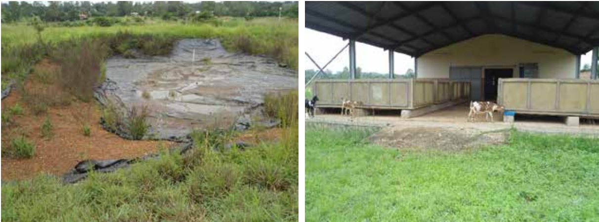
Dilapidated pond liners and bushy ponds (left) and non-functional hatchery unit (right) at Gulu Fish Fry Centre in Ariyaga East village, Gulu District
