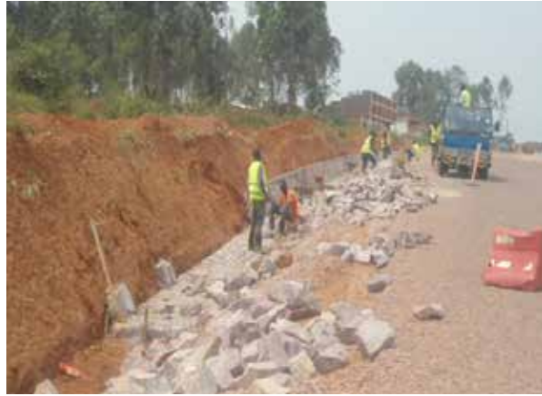
Stone pitching works along Kanoni-Sembabule & Semambule-Villa Maria (110 km) at km 7+000 in Kikoma Town
