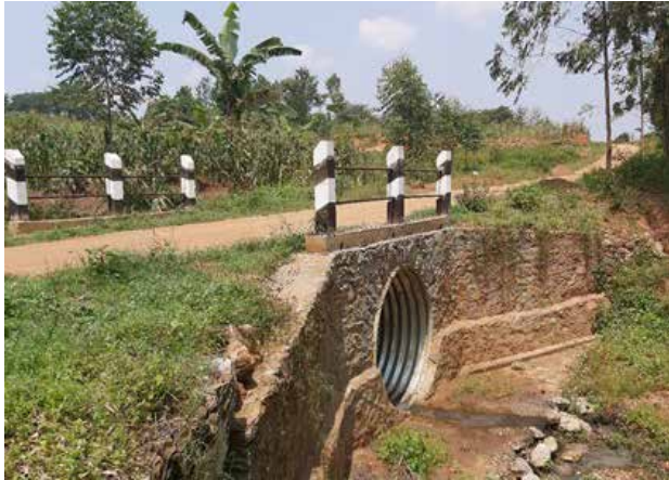
1.2m diameter Armco culvert installed on Mulatsi-Bukiende Road across a stream in Bukiende sub county
