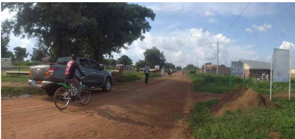
Partially completed grid extension scheme at Barlonyo Trading Center , Lira District funded by IDB
