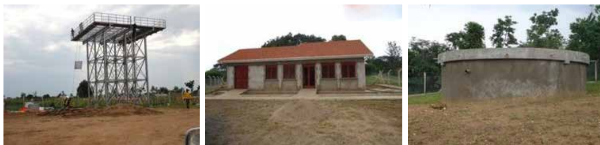
L-R: Assembling a 259 m3 steel tank in Molo Sub-County, Tororo District; A Water office; and a 191m3 concrete tank at Sibanga Sub-County in Manafwa District
