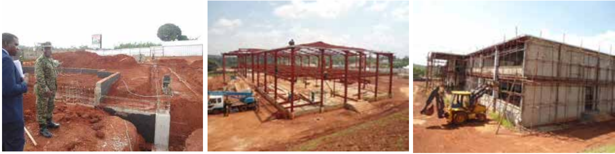
L-R: Progress on construction of the ICT Innovations Hub at Nakawa in February and July 2018, and February 2019
