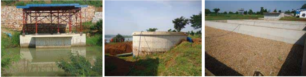
L-R: Intake works; Clear water tank; and Sludge bed structures of the Kayunga-Busana Water Supply Scheme in Kayunga District
