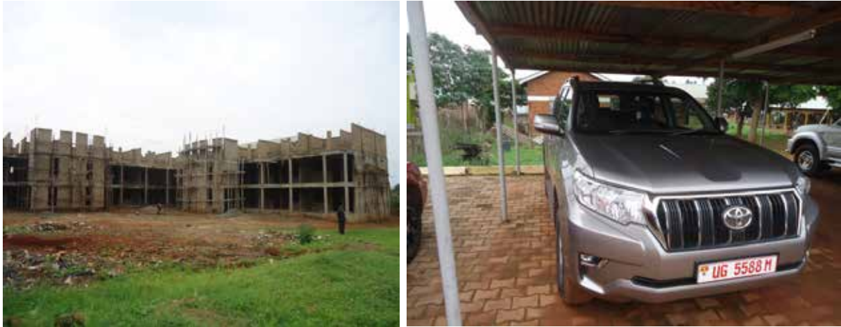
L-R: Staff house under construction and the procured station wagon for the director Gulu RRH
