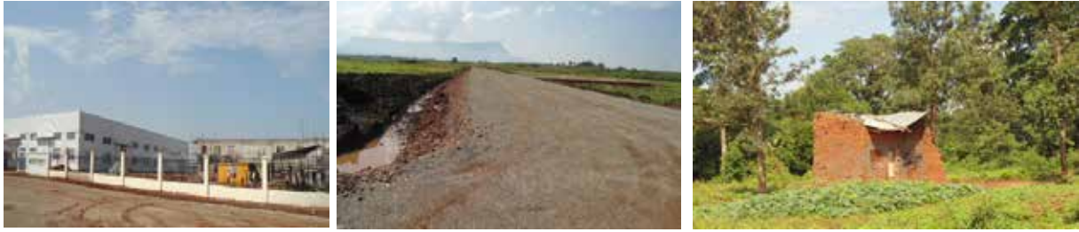
L-R: Pearl Light Tech Company, ongoing road construction works and a house for one of the remaining squatters at Mbale Industrial and Business Park
