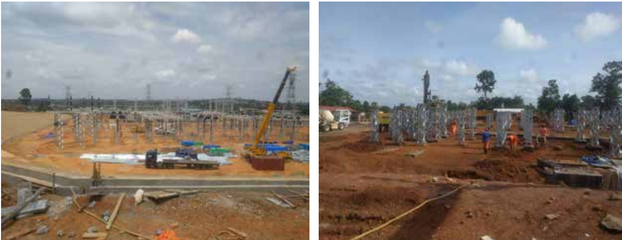
L-R: Partially complete works at Kawanda substation; Ongoing civil and mechanical works at Lira substation
