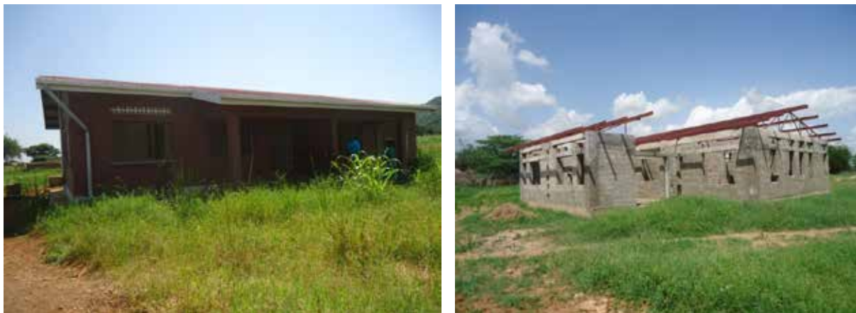
L-R: Abandoned sites staff house at Alarek HCIII in Abim and Lokopo HCIII in Napak District
