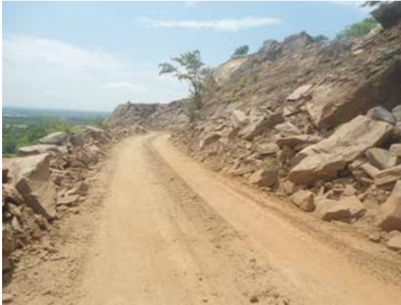
Blasted rock on Hoima-Butiaba Wanseko Road at km 34+000 Road
