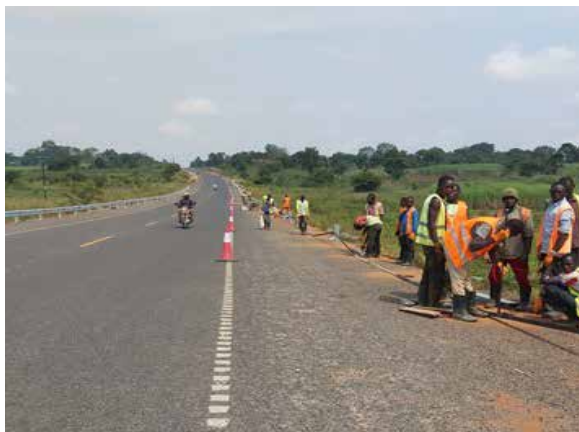
Installation of guardrails at a trial section (km 24+100) on Musita- Lumino Road
