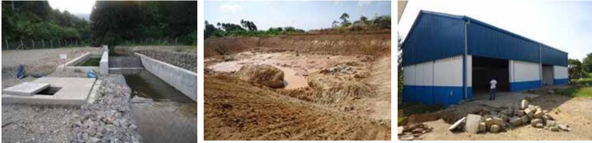
L-R: Source protection works; a 750m 3 reservoir valley tank and produce storage facility of Rwengaju irrigation scheme in Kabarole district.
