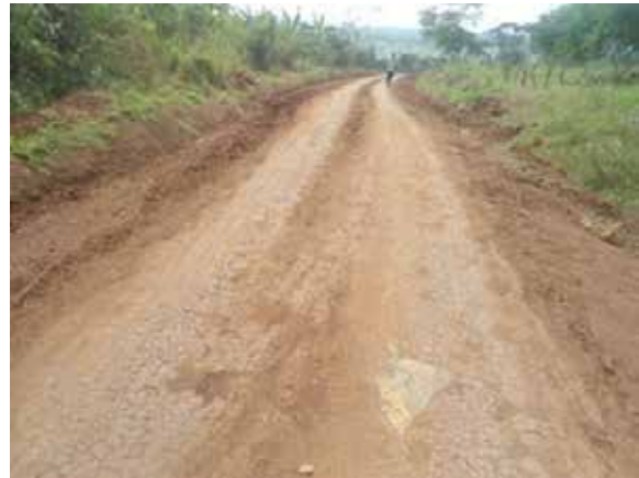
A section of Rwebikoma-Kijuma-Rwakitura Road with loose material at 10+900
