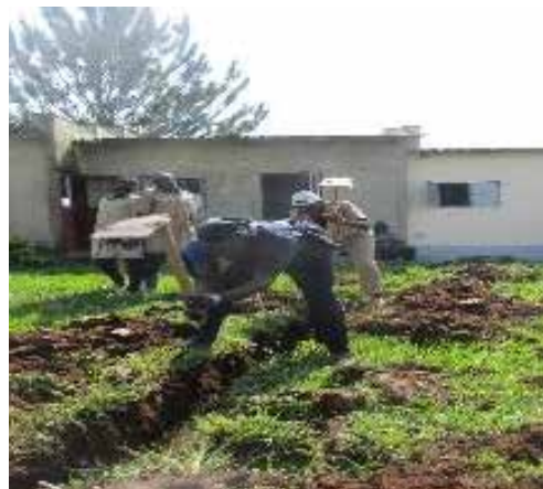
Electrical Installation students laying conduit pipes and excavating for power extension at the NUYDC in Omoro District
