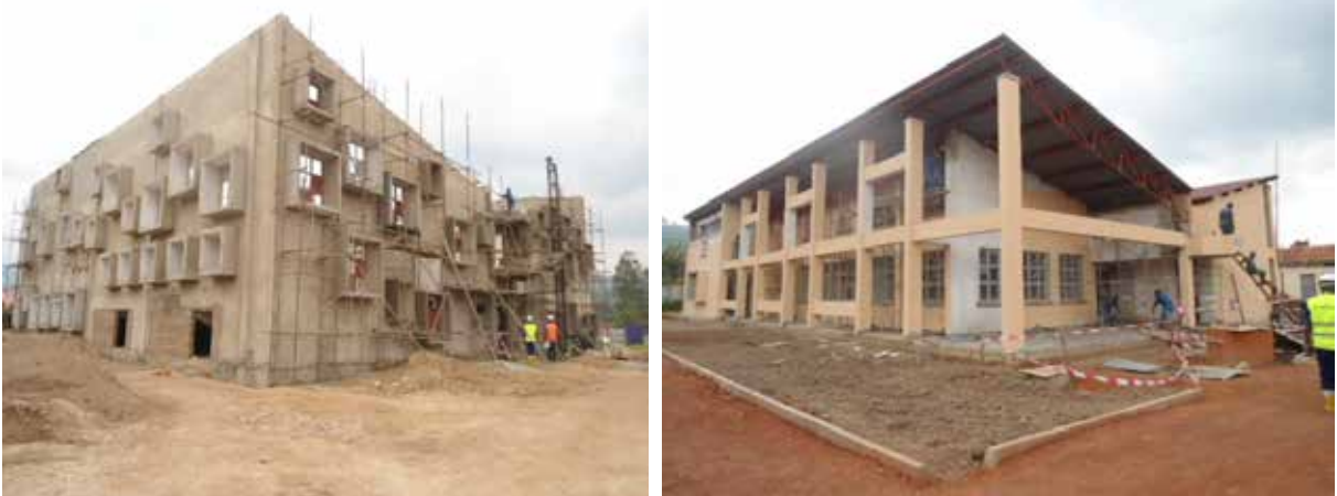
Left: On going works on the Library/Resource centre, Right: Ongoing works on the Administration block at Kabale National Teachers' College
