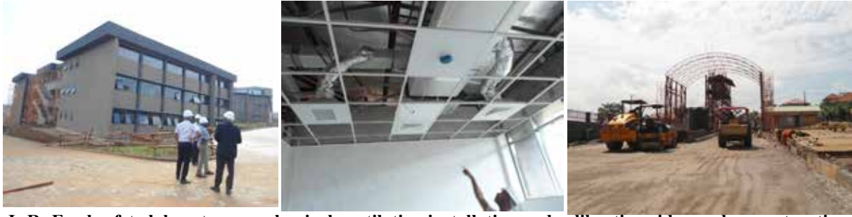
L-R: Food safety laboratory, mechanical ventilation installation and calibration ridge under construction at UNBS headquarters
