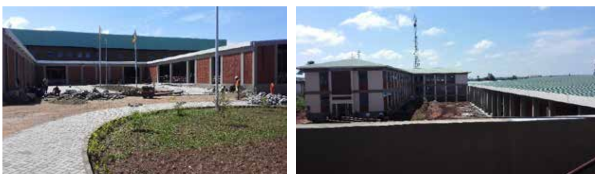
Ongoing civil works at the main building and various works at Kayunga Hospital
