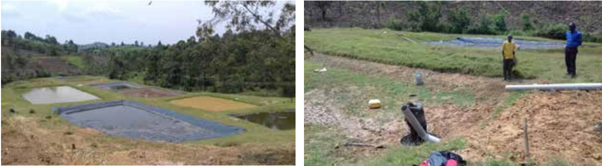
Rehabilitated and stocked ponds (left) and ongoing installation of new piping for ponds at Bushenyi Fish Fry Centre in Bushenyi Municipality in Bushenyi District
