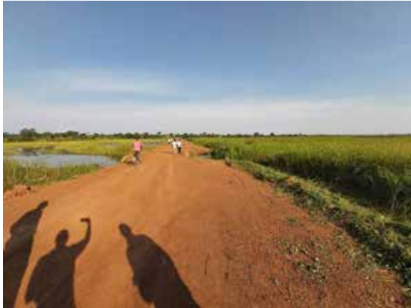
Raised and gravelled swamp section at the Kangai swamp crossing – Dokolo District
