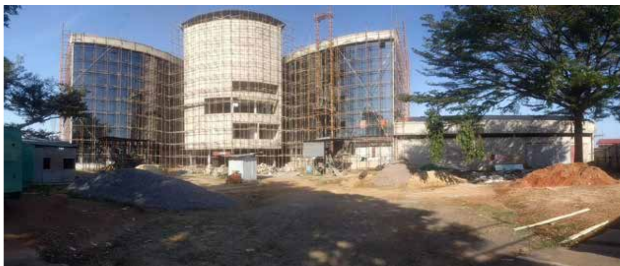
Ongoing finishing works on the offices for the Petroleum Directorate and Petroleum Authority in Entebbe
