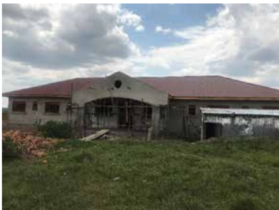
Hostel for artificial insemination staff under construction in Kayonza village in Kiruhuru district
