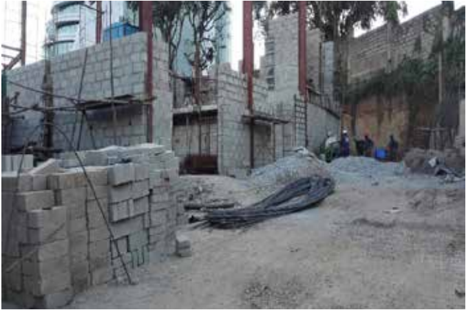
Ongoing activities on the cold rooms and stores at Nakasero Blood Bank, Kampala
