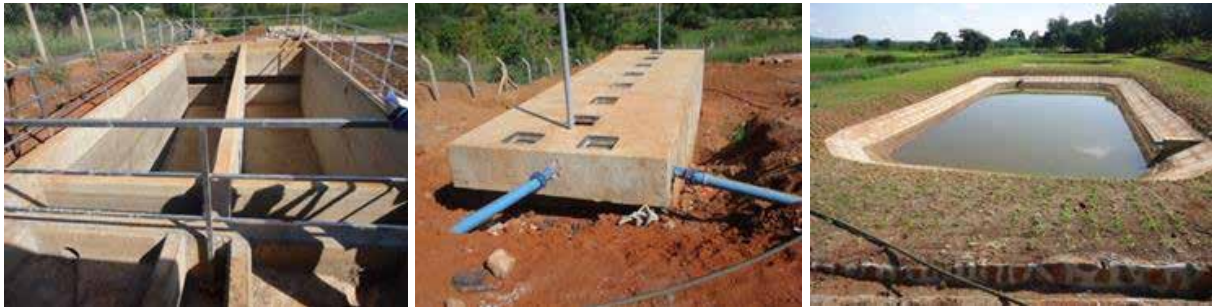
L-R: Thickening/settling tank; anaerobic buffer load reactor; and facultative ponds of Kiboga faecal sludge in Kiboga District
