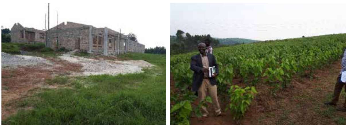
L-R: Incomplete rearing houses and part of the mulberry plantation in Sheema District
