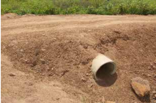
Incomplete cross culvert along Asamuk – Odon – Akore road
