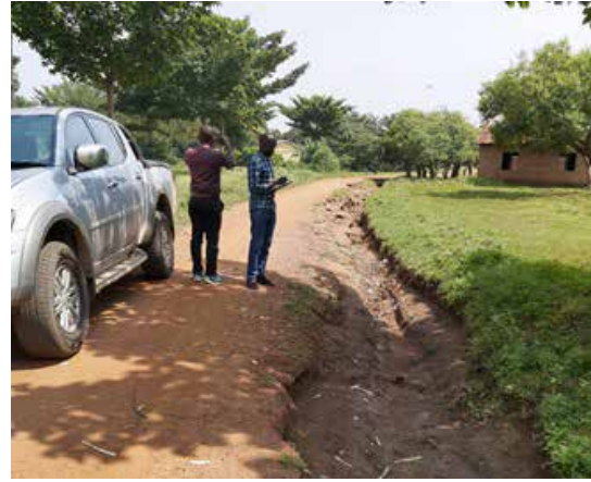
Severe scouring of side drain on Busoba – Makhai Road due to heavy rains
