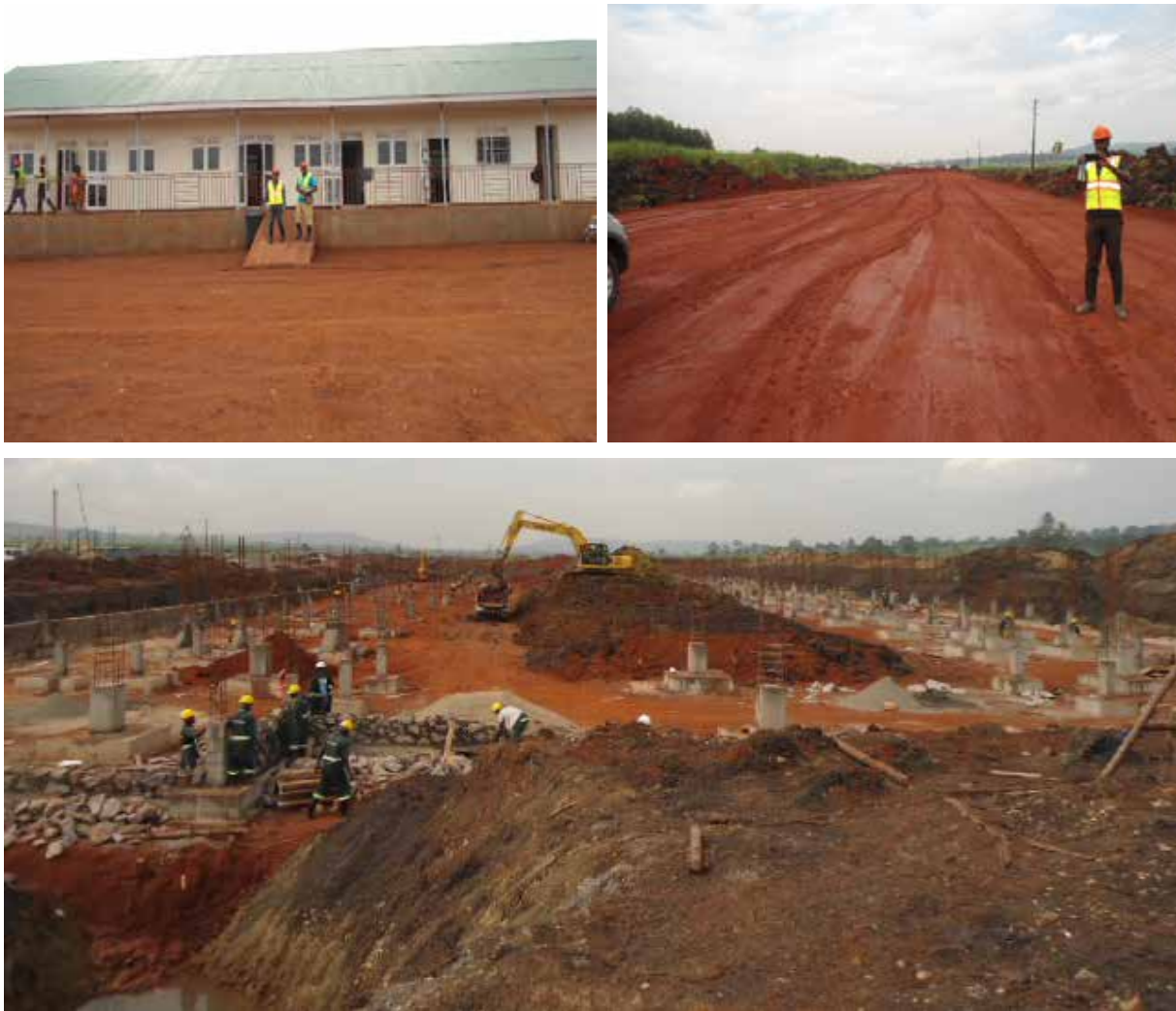
KMC site office block, b) dual carriage road under construction and c) sub-structure of KMC vehicle assembling plant
