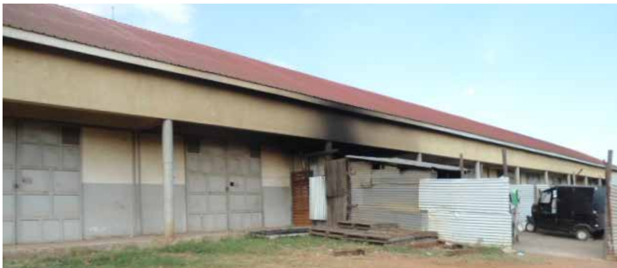
One of the blocks in Mbarara SME Park with unapproved structural alterations
