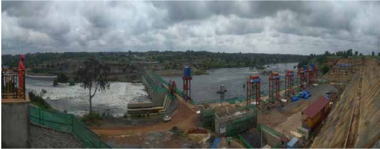
Upstream view of the Karuma hydropower project showing the completed power intake section(Right) and the spillway(Left)
