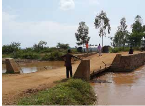
Manafwa Bridge at km 12+600 on Busolwe-Nabumali Road. The low-lying section floods during the rainy season
