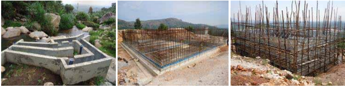
L-R: Source head works; Sedimentation tank reinforcements; clear water tank for the Nyabuhikye-Kikyenkye water supply scheme in Ibanda District
