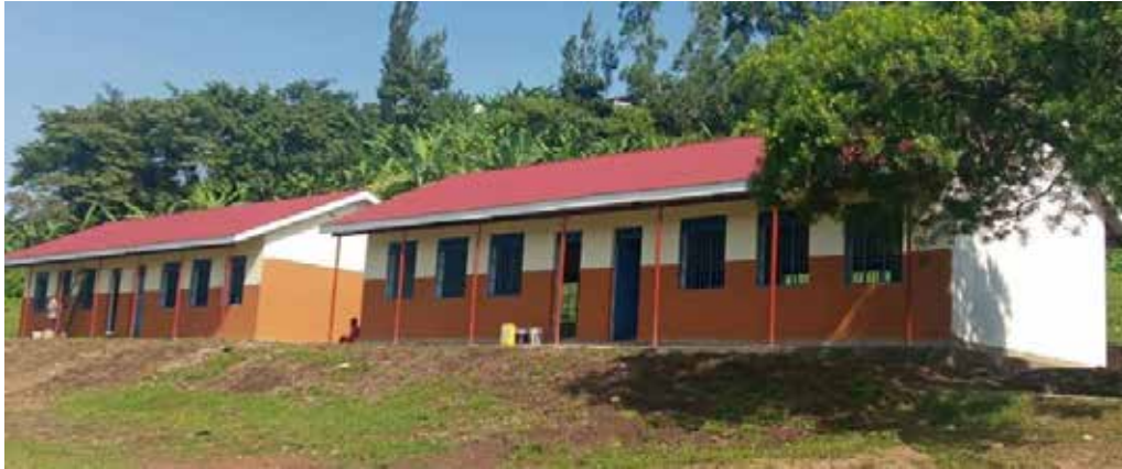
Completed two classroom blocks under Emergency Construction of Buyobo Primary School in Sironko District
