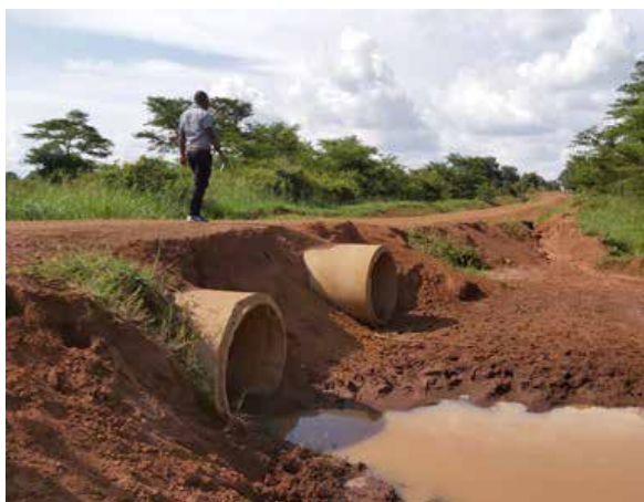
Incomplete culvert installation on Paloga – Madiopei road; graveled section of the road
