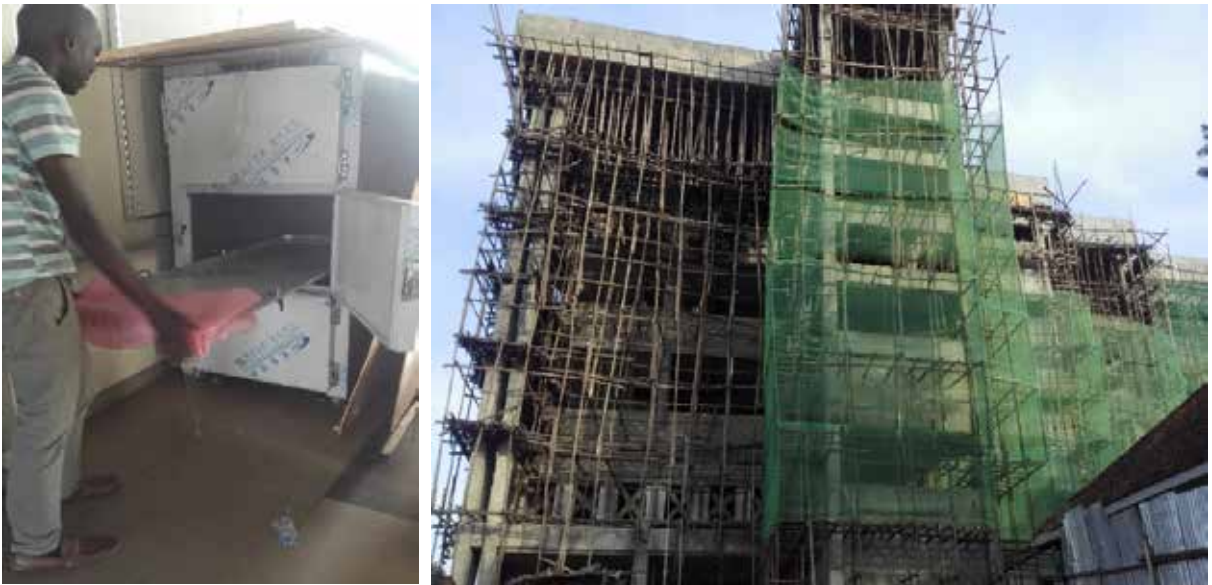
L-R: Maternity and Child Complex under construction. Newly procured mortuary fridge at Masaka RRH
