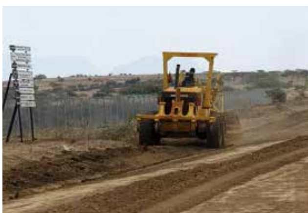
Graders on Maintenance of Nadunget-Nawanatau Acherer 12Km community access road, Nadunget sub-county, Moroto District
