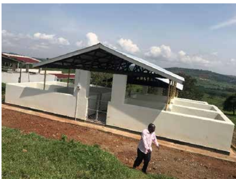
Completed pig sty at Njeru Stock Farm in Kiryowa village, Njeru Town Council in Buikwe District
