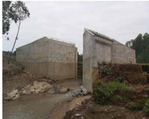
Completed abutments of Namunyiri bridge waiting to receive the deck at km 38 on Bumbobi – Lwakhakha
