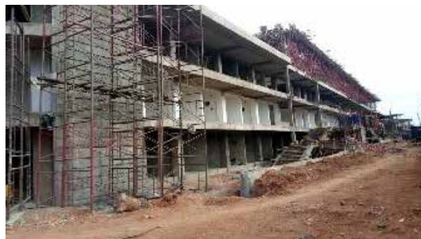
Commenced on roofing, finishing works including plastering painting, terrazzo laying at Soroti Central Market
