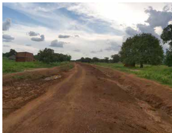
Gravel dumped on Padibe - Paloga - Madiopei Road. Gravelling works were halted due to breakdown of the grader
