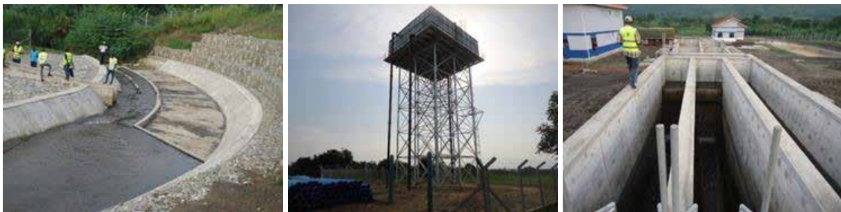
L-R: Source protection works; Kanara reservoir tank; and Water treatment structures for Rwebisengo-Kanara water supply scheme in Ntoroko District
