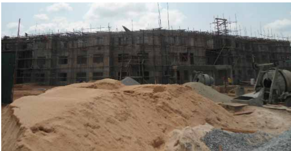
Construction of the male dormitory block in progress at Uganda Petroleum Institute Kigumba (UPIK)
