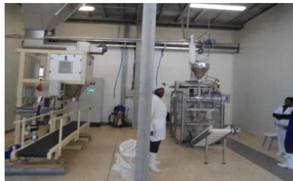
Installed machinery at the PIBID in Bushenyi
