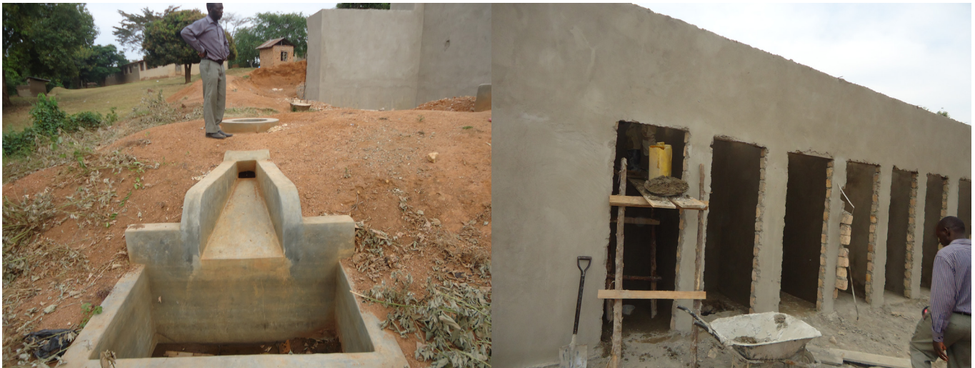
Left-Right: Bio-digester; plastering works on the bio-latrine at Kitagobwa SS, Ngando sub county, Butambala District
