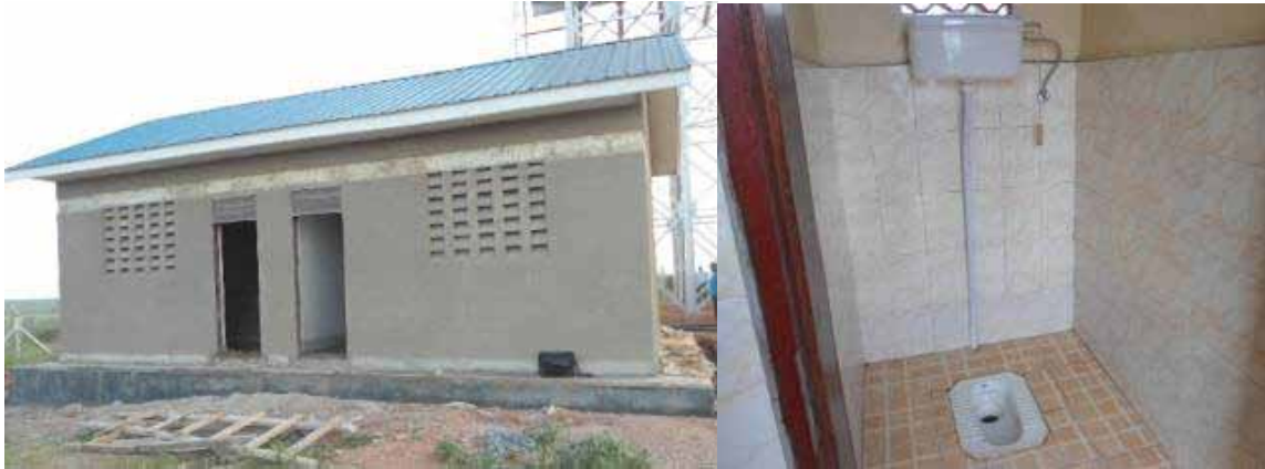
Water treatment house (left) and a water borne toilet for a public place (market place)
