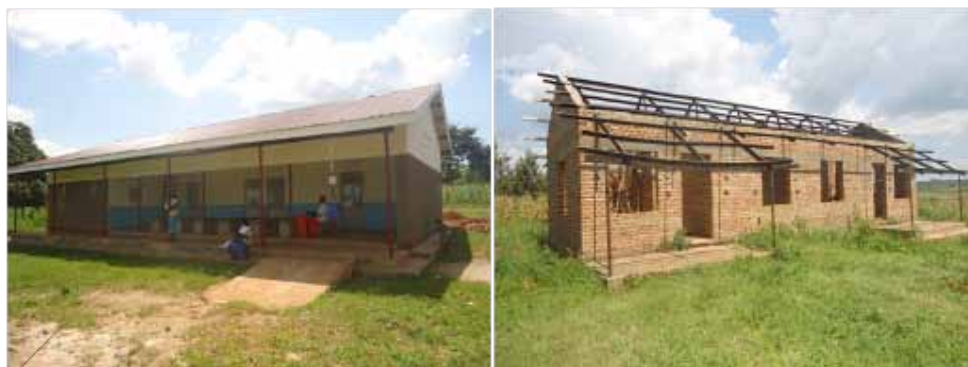
Left to right: nearly completed OPD at Muterere HCIII and Staff house construction at Maziriga HCII
