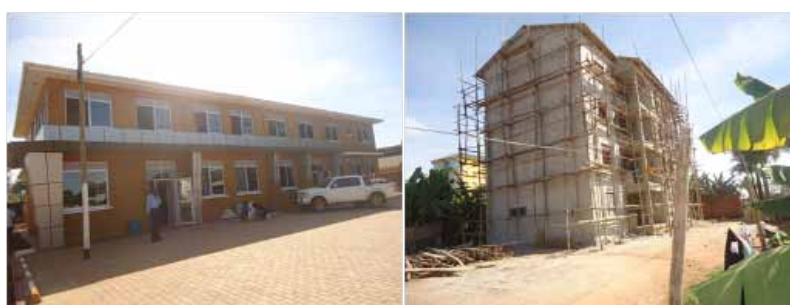
Left to right: Nearly completed administration block and staff quarters under construction Gulu RR hospital
