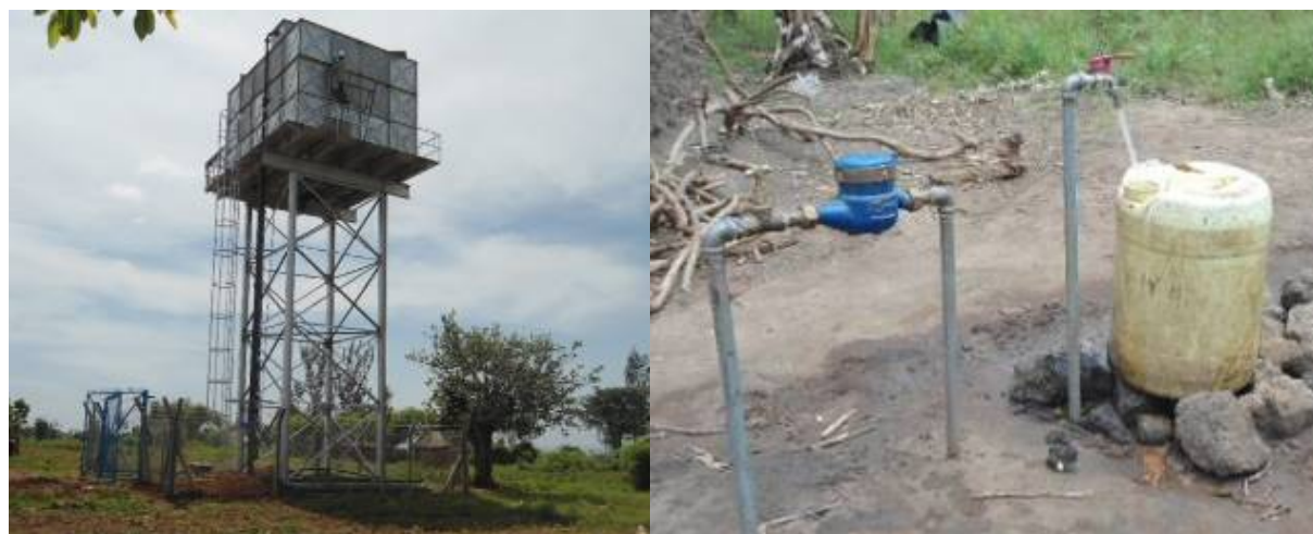
A reservoir tank with completion works ongoing and water flowing on a public tap stand as witnessed above
