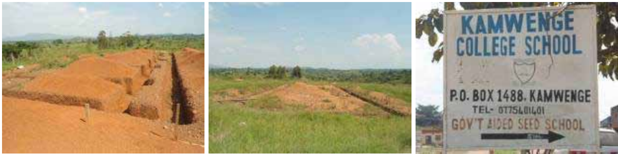
This is the abandoned construction site by Ms Lamba Limited at Kamwenge Seed School (Also known as Kamwenge College School).
