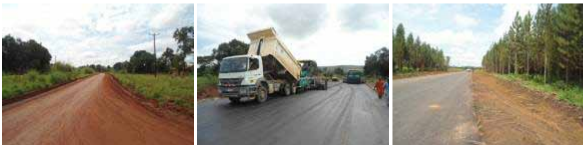
(Left): Maintenance of existing road where works have not yet started between Km 0+000 and 5+300; (Centre): Ongoing asphalt works at Km 6+480. Clearing, grubbing and removing of top soil at Km 17; (Right): Drainage works ongoing at Km 10+000, an area that had previously not been handed over due to compensation issues.
