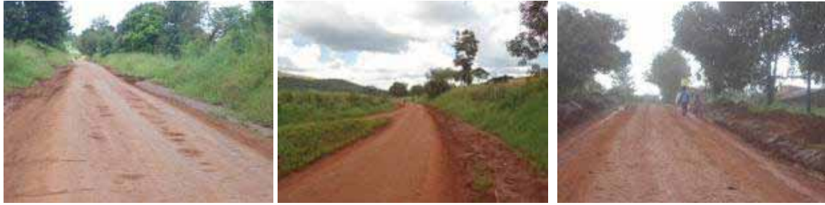
(Left): Damaged section due to poor drainage of Masindi-Kigumba road at Km 20+000; (centre); A graded section with high silt load on the right on Masindi-Hoima road; (right) A freshly graded section on Masindi-Biiso road at Km 26+500.
