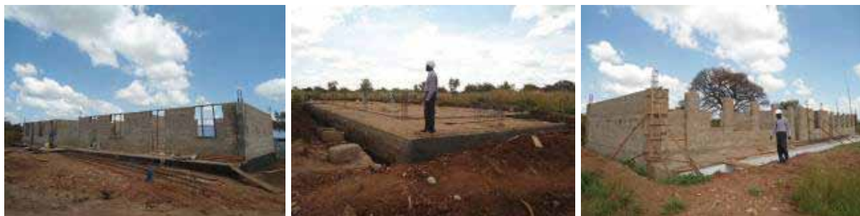
From left: The administration block was at ring beam level, 3 unit science block going on to ring beam and multi purpose storied 6 classroom block at ground slab level at Ogoko Seed S.S.
