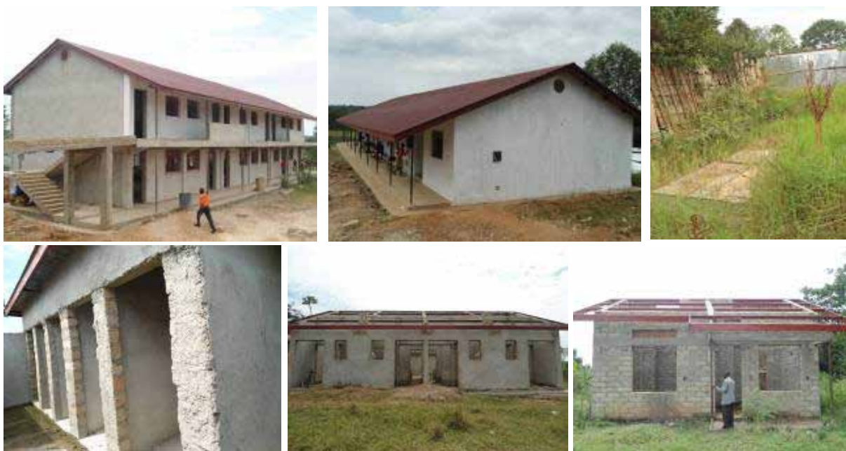
From top left, A multi purpose storied block, library with computer laboratory and a 3 stance VIP abandoned at slab level From bottom left: A stalled 5 stance VIP pit latrine, a 4 unit teachers' house and a 2 bed roomed head teachers' house that stalled at Bulamu Seed S.S.
