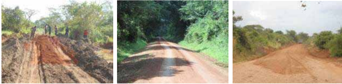
Left: Swamp filling with murram at Km 12+000 on Ikooba-Ntoma road (2Kms); Centre: A graded section with grass cut sides at Km 27+800on Kisanja-Park Junction road in the Mruchision Falls National Park; Right: End of grading works on Kisanja-Park Junction road at Km 77+700.
