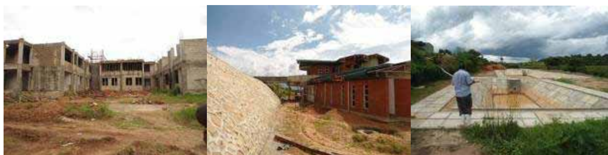
Left-ongoing final finishes at conference/office block with soil retainer wall, Centre- laying of second floor slab at Research laboratory block, and Right-completed waste water lagoons
