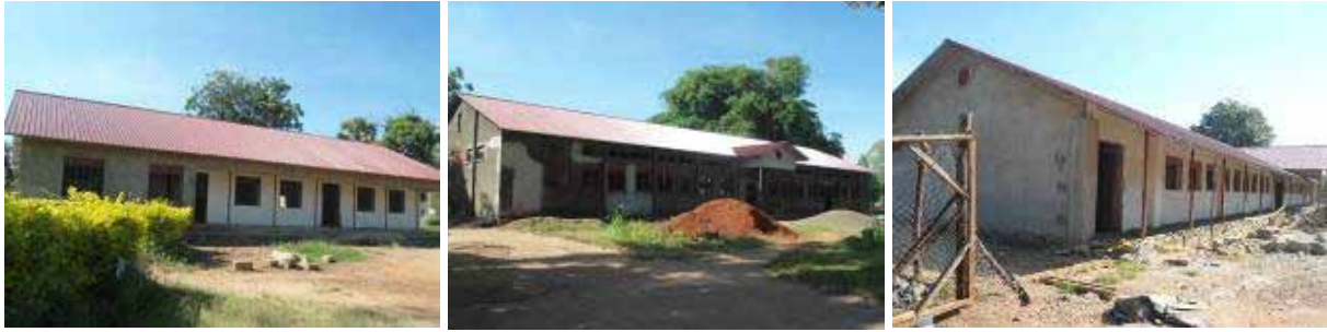
From Left: Renovation and extension of the old administration block, the dining/kitchen block and the new 300 seater library at finishes level at St Catherine Girls S.S.
