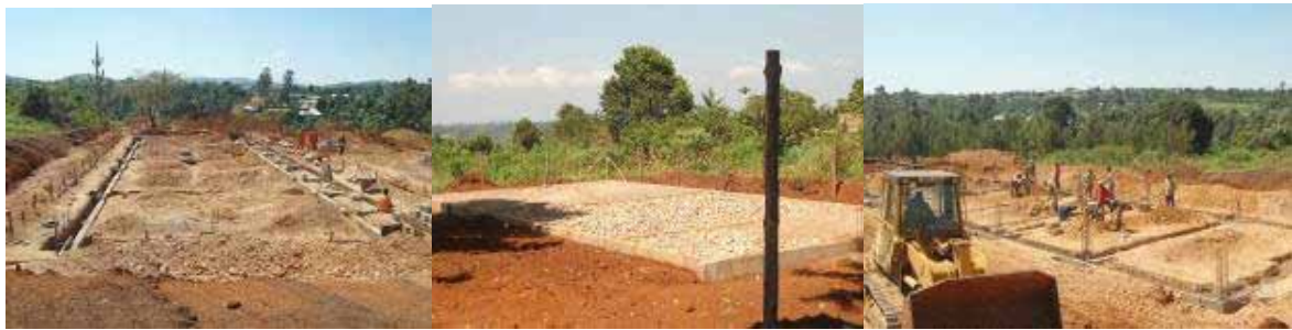
The ICT block, the multi purpose hall and the storied 8 classroom block at Kitara S.S.
