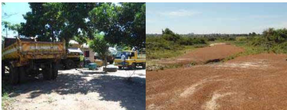
Mobilised equipment currently idle and parked at the campsite and deteriorating earthworks along Temele road, Soroti
