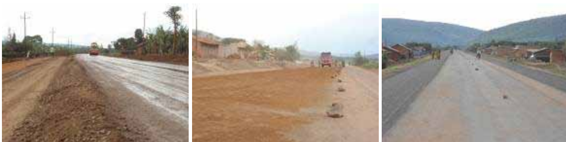
(Left): Ongoing base course works at Km 39+700; (Centre): Curing of a primed surface with sand at Km 46+980; (Right): Double surface dressing on the road shoulders and priming in the carriage way at km 49+931.
