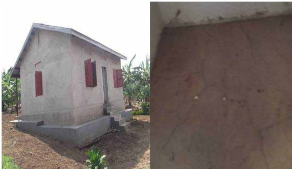
Left to right; resettlement house and cracked floor of resettlement houses constructed by Lamba investments that abandoned site on the Mbarara-Nkenda transmission line
