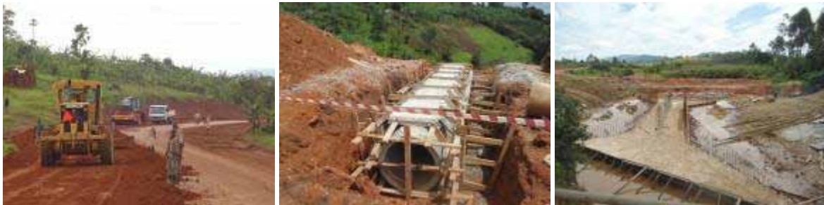
(Left); G15 material subgrade works at Km 8+928; (Centre); 900mm diameter culvert construction at Km 15+000; (Right); Bridge foundation works at Km 17+470.
