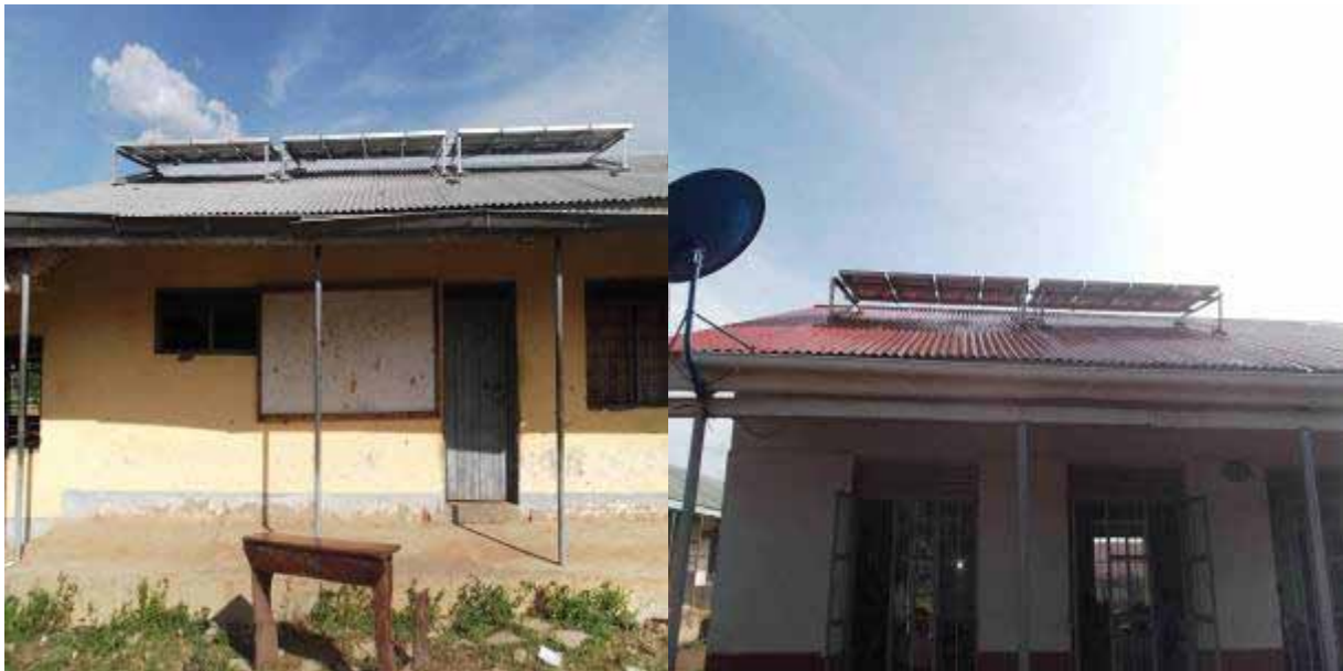
Left: Installation of solar panels at Yumbe Secondary School and Right solar installation at Aringa Secondary School.
