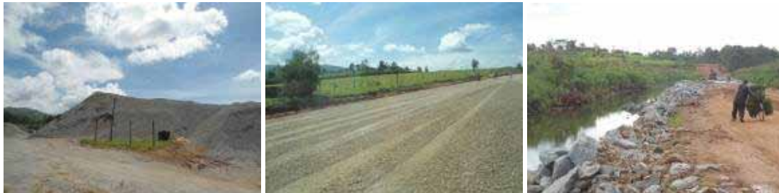
(Left); Stock piled CRR material at contractor's camp at Km 19+500; (Centre); A trial section near the contractor's camp; (Right); Swamp treatment works at Km 25+500.
