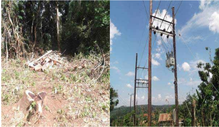
Left: Bush clearing to pave way for power line in Budongo Forest; Right: Stringing and installation of transformer on Masindi-Waki-Bilisa power line
