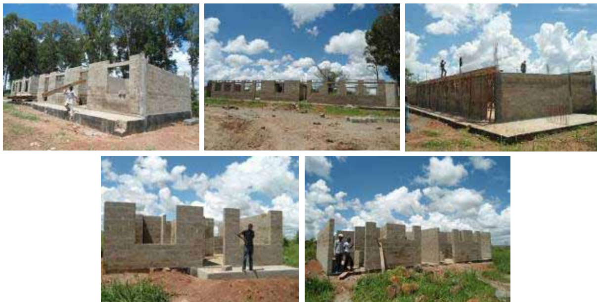
From the top left, construction of the administration block at ring beam, the 3 unit science laboratory at ring beam, the storied 6 classroom block shuttering for 1 st floor slab level, the 4 unit staff house and the 2 bedroom house at ring beam level at Purongo Seed S.S
