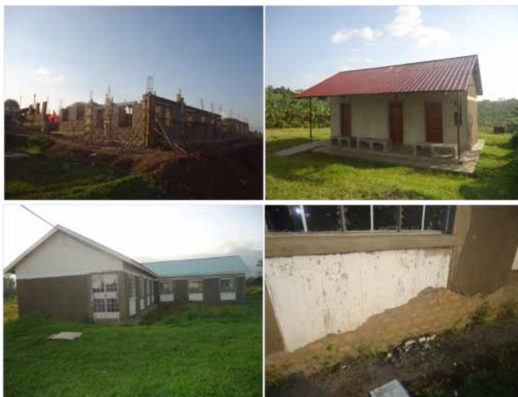
Top left to right: Maternity ward at Kibito HCIV and Completed OPD at Nyamiseke HCII Bottom: General ward at Kisomolo HCIII and Plaster that has give way on the general ward Kisomolo HCIII
