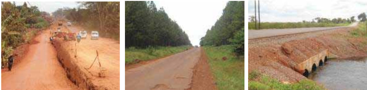
(Left); Embankment filling near Namulesa TC at Km 4+500. (Centre): A section of the road at Km 15+000 where works have not yet started. (Right); A completed section at a swamp crossing at Km 37+800.
