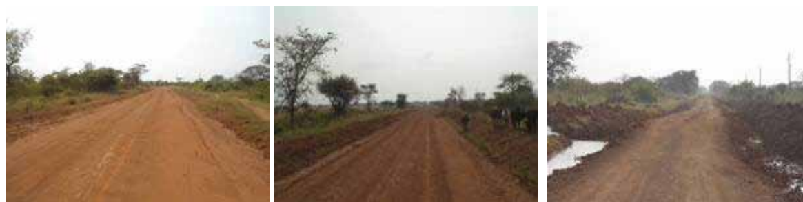
(Left): Corrugations on Arapai-Katakwi road at Km 23+600; (Centre); A well graded section on Katakwi-Iriiri road at Km 11+700; (Right) A regavelled section on Katakwi-Iriiri road at Km 30+400 done by UNRA using force on account because the contractor was not on site in early November 2013.
