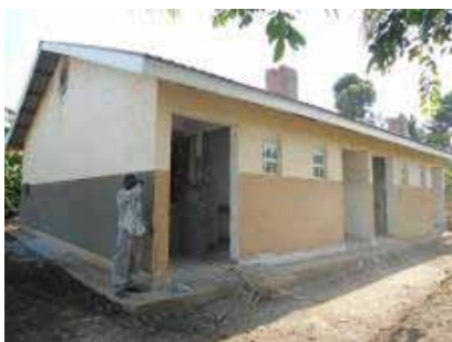
From the top left, a storied 4 classroom at finishes level, a library block at finishes, a 2 bedroom house and a 4 unit staff house all at finishes level at Bubandi Seed S.S.
