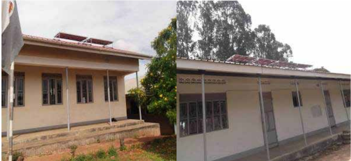
Solar Panel installation at Nyarilo Secondary School and St. Charles Lwanga Koboko
