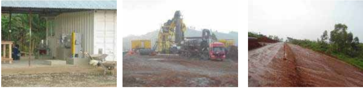
(Left); Laboratory Testing equipment at the Supervision Engineer's Camp at Km 18+500; (Centre): Setting up of the asphalt plant at the Contractor's camp at Km 19+500; (Right); Section of the road at Km 25 undergoing cut and fill as part of road bed preparation works.
