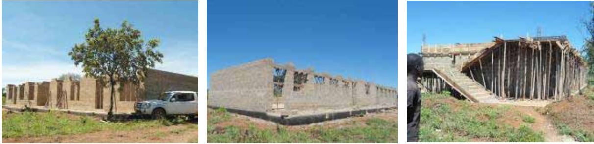
From left: The administration block at ring beam level, the 3 unit science laboratory block at ring beam level and the storied 6 classroom block at shuttering for the first floor slab level at Patongo seed S.S.
