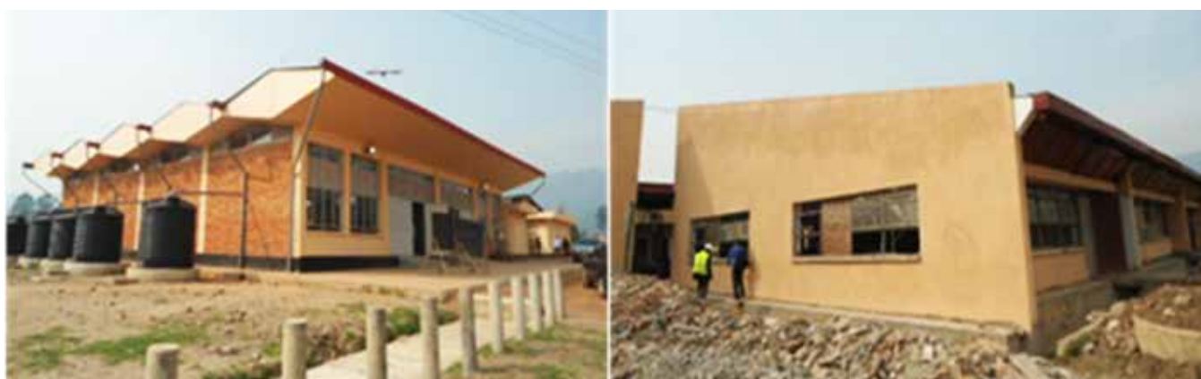
Left: completed renovation of the Multi purpose hall, Right: Renovation of the Science Laboratories at 75% progress at NTC Kabale under BTC.
