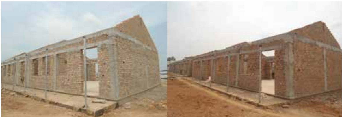
Left: Science Laboratory at wall plate, Right: 3 blocks of classrooms at a wall Plate at Nyakashashara Seed S.S. Kiruhura district
