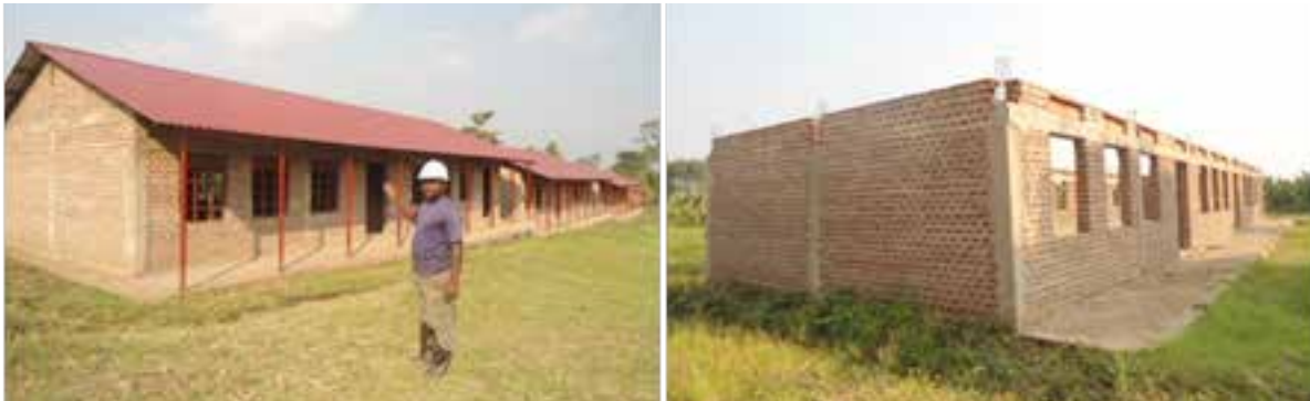
Left: 3 blocks of classrooms roofed, Right: A Multi purpose Hall at a wall Plate level at St. Paul Nyabweya (Kase bde S/C) in Kabarore district under UgIFT
