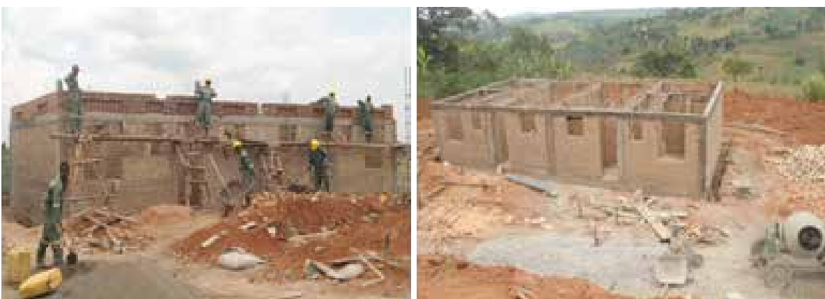
Staff quarters at wall plate level in Kigando Seed S.S in mubende district under UgIFT
