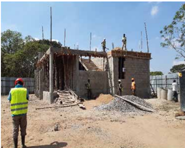
Incomplete Support to Teso Regional Office in Soroti Municipality
