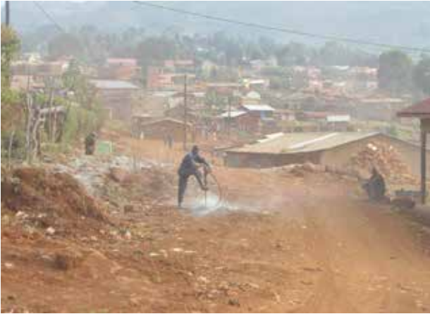
Drilling of a rock as part of the preparation for rock blasting on Chebrot road in Kapchorwa
