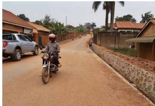
Movit Road (1.2km) in Makindye-Ssabagabo Municipality was upgraded to bitumen standard and the side drains constructed
