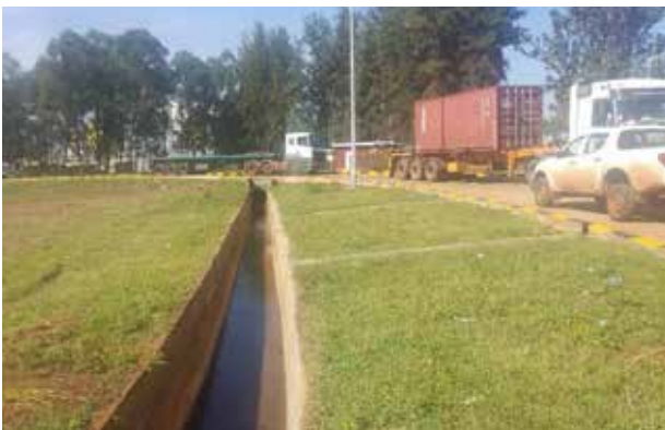
Drainage and landscaping works along the exit road of Uganda to Kenya
