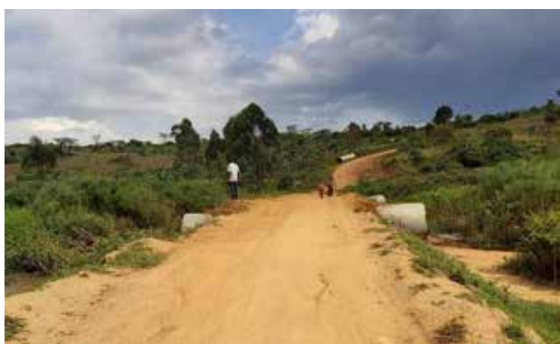
A swamp section at km 33+400 on Kitenga-Ikula-Kanyogoga Road that was raised under emergency works using FA in Q2 FY2019/20
