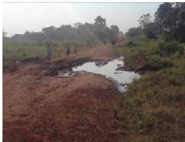
A section with a pothole along Aduku-Agwata Road at km 16+700
