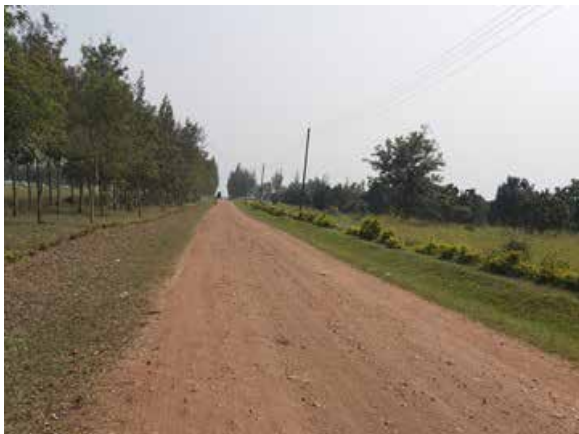
Access road to Hima Army Barracks after routine mechanized maintenance in Q1
