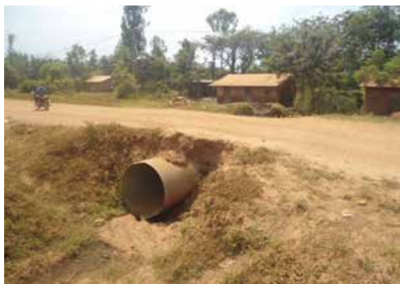
An Armco culvert of 1.2m diameter installed at 1.2km along Muyembe-Namalu Road
