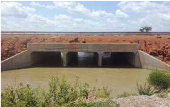
The three cell (3 by 4.5) m Opot Box Culvert along the Amuria-Amudat Road
