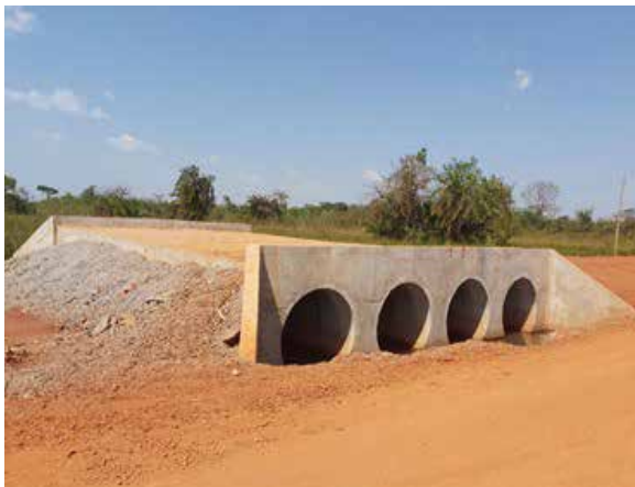
Four lines of 1.5m diameter pipe concrete culverts installed at a swamp section on Kigumba – Bulima (69km) at km 17+400
