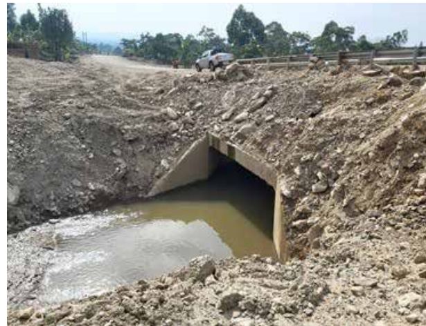
One of the sections of Fort Portal – Bundibugyo road that was cut off by landslides
