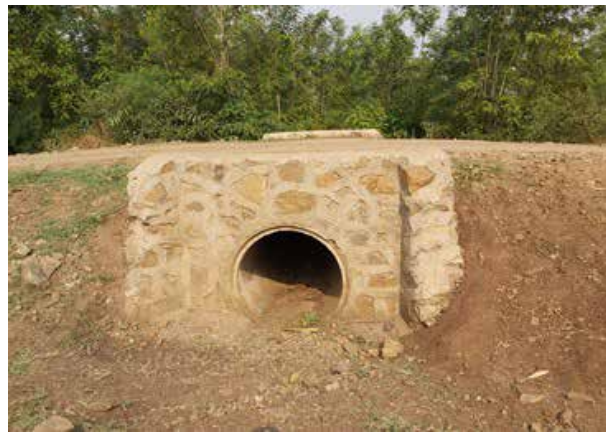
900mm diameter culvert installed on access road to Rwimi and Ibuga Prison Farm under RMeM
