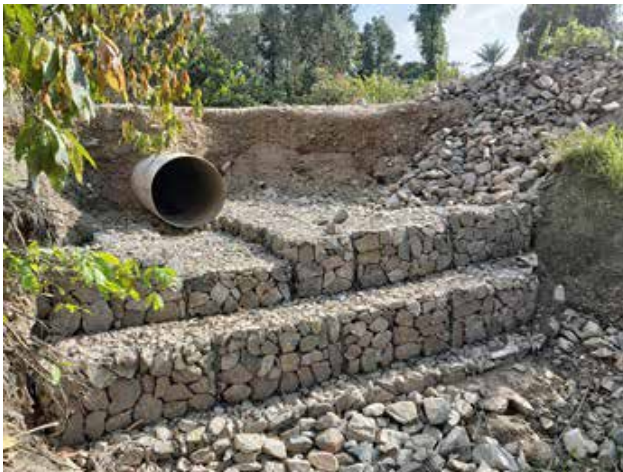
Gabion protection works on Ntandi-Kikyoo Road; part of the emergency interventions after the landslides
