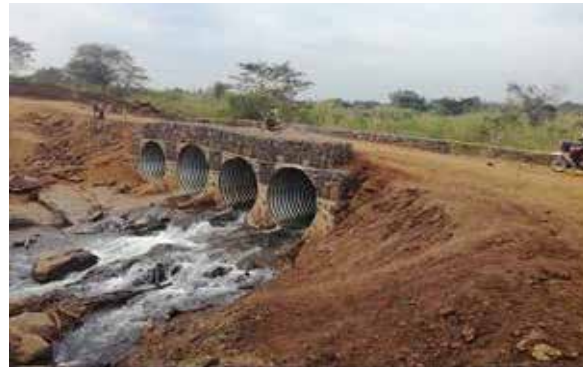
Temporary diversion works at Aji Bridge on Anyirigu-Ofaka Road in Ofaka sub-county in Madi Okollo district
