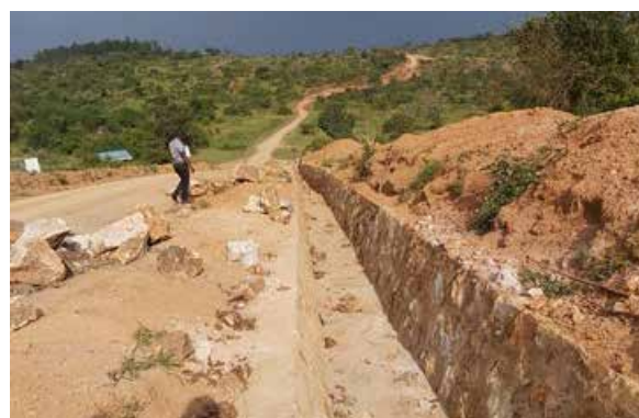
Stone pitching of side drains on Kitenga-Ikula-Kanyogoga road at km 25+400. Works were halted due to heavy rains
