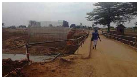
The abutment for the new bridge undergoing curing and the Old Enyau bridge on Owafa-Kubala-Omugo Road in Maracha-Terego District
