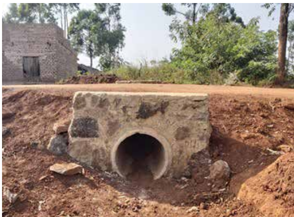
A 600mm diameter culvert installed at km 4+500 on Haibale-Hanga-Buhirigi road in Q2
