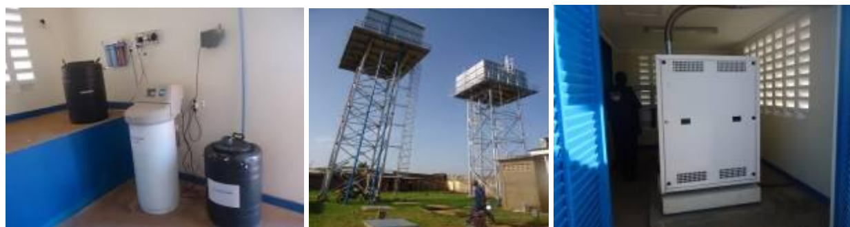
L-R: The chlorine disinfection equipment; New and old 100m 3 reservoir tanks; The 80kVA generator all in Kaliro TC, Kaliro district
