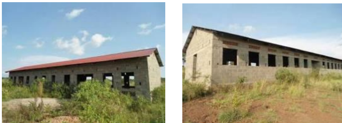
Two workshop blocks left incomplete at Engineer Kauliza Kasadha Technical Institute – Bugiri District
