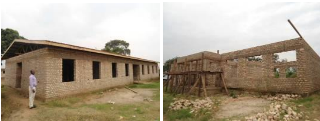
Left: Dormitory, Right: Administration block at ring beam level at Rakai PTC
