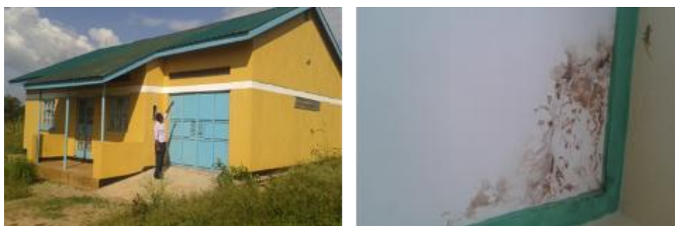
L-R: Renovated Doctor's house and a leaking ceiling at Nankoma HCIV, Bugiri district
