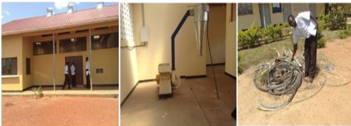
Left: Non-functional APF, Middle: Incomplete rice mill installation abandoned; Electrical items abandoned by the contractor since August, 2015 at barr-subcounty in Lira district
