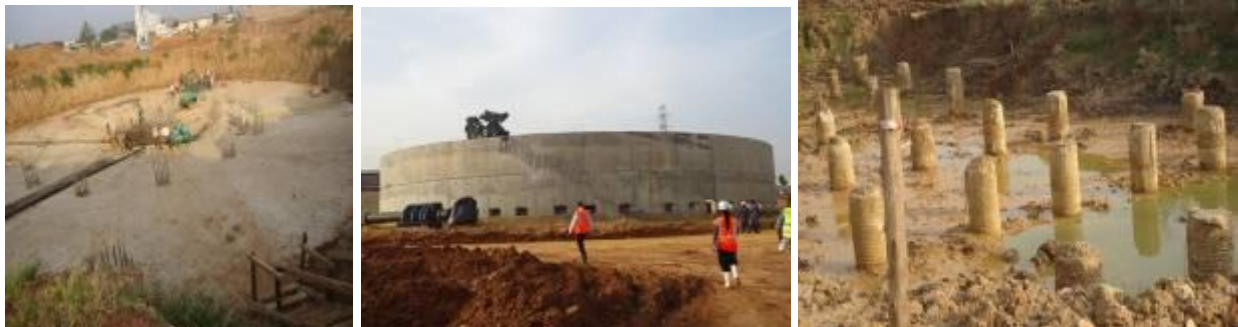
L-R: Sedimentation tank base; Trickling filter; Sedimentation tank pile foundations at Bugolobi, Kampala district
