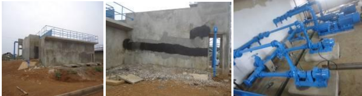
L-R: Sedimentation tank; Sealed leaking joint on the sedimentation tank; Pumps at the treatment plant, Mpigi district
