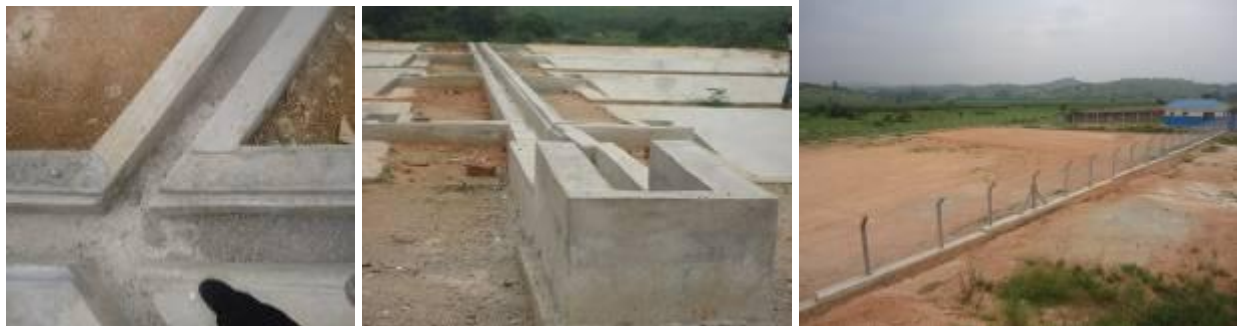
L-R: Cracked sections of the sludge drainage channel; Inlet chamber and main drainage channel; Compacted ground for the solid waste disposal site, Ntungamo district
