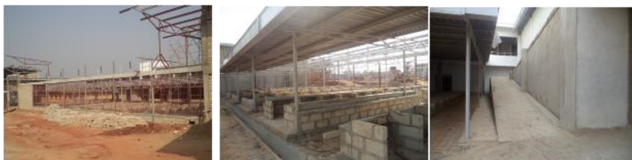
Left: Constructed columns; Middle: dry fish stalls; Right: Ramp for PWDs and other people to enter into the first floor on site in Nyendo, Masaka Municipality
