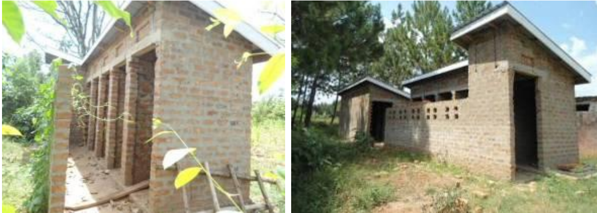
The five and the six stance VIP latrines and the shower block at Kaliro PTC
