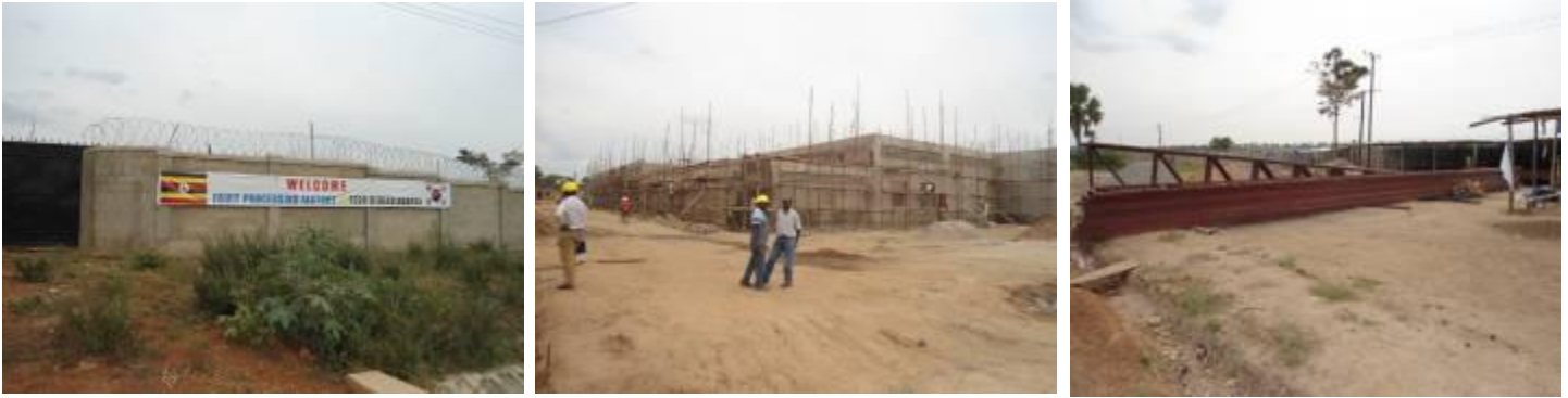
Left: External wall completed at Soroti Fruit Factory, Centre: Ongoing civil, Right: fabricated trusses on site
