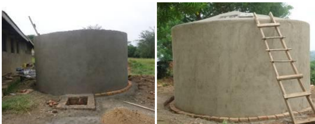
Left: Newly constructed rainwater harvesting tanks at Gentebe P/S and Right Kasana CoU Mijwala sub-county, Sembabule district
