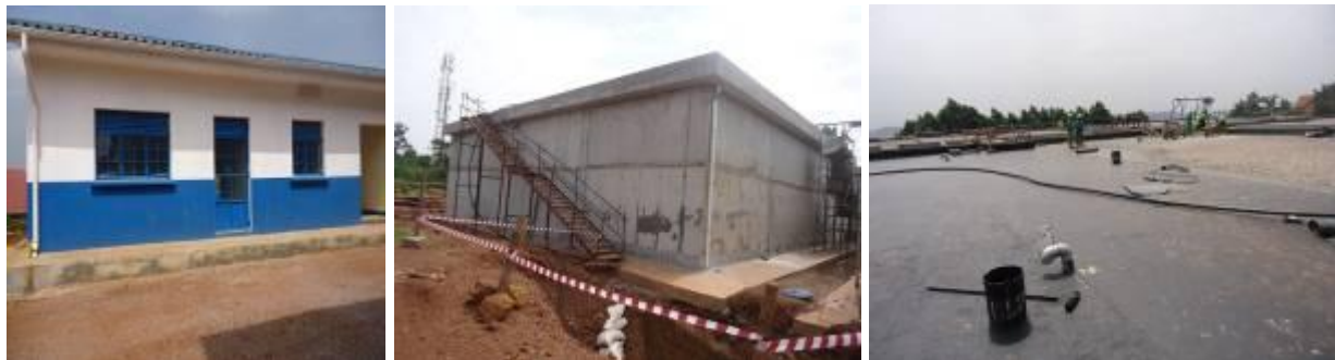
L-R: A section of the office building; One of the reservoir tanks; Placing bitumen on top of one of the tanks at Namasuba Hill
