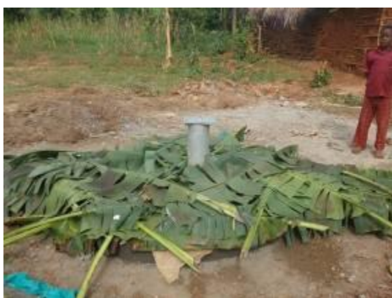
Left: A newly constructed deep borehole at Kabowa Town Council. Jinja district
