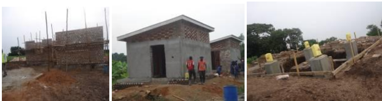
L-R: Pump House 3 and Chlorine House on Kikoni Hill; VIP toilets at St. Luke Primary school; and Stud columns on Kikoni Hill in Bukakata sub-county, Masaka district
