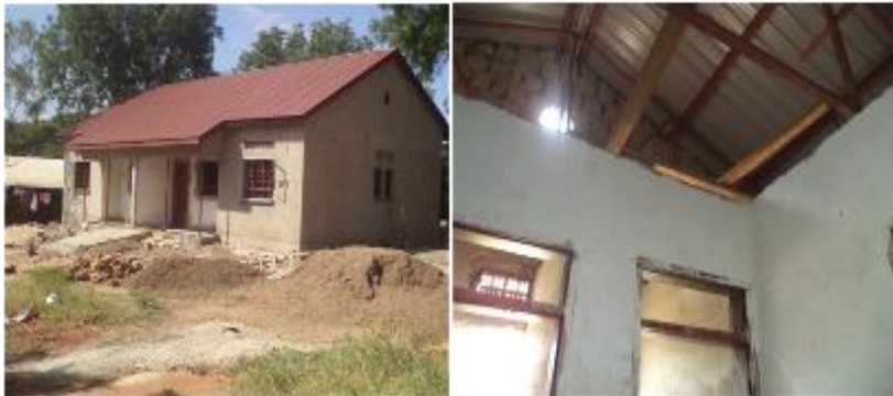
Left: One of the constructed teacher's houses; Right: One of the houses pending fixing of ceiling in Moroto district
