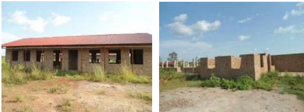
Left: A two classroom block, Right: An administration block left incomplete at Engineer Kauliza Kasadha Technical Institute – Bugiri District
