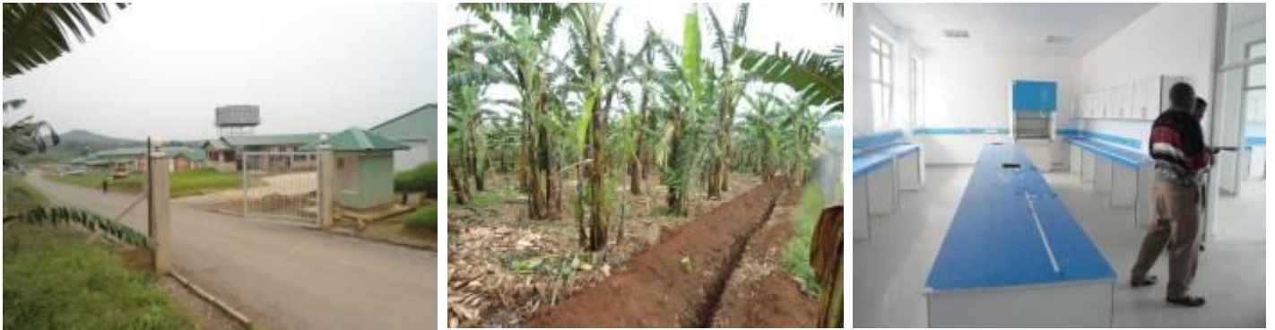
L-R: A section of road works awaiting completion, trenches for irrigation of the banana plantation and one of the Quality Assurance laboratories fitted with furniture
