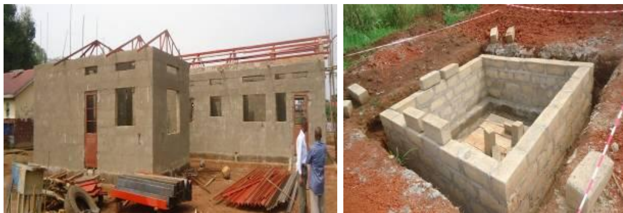
L-R: Ongoing construction of the Maternity block and Placenta pit Aduku HCIV, Apac district
