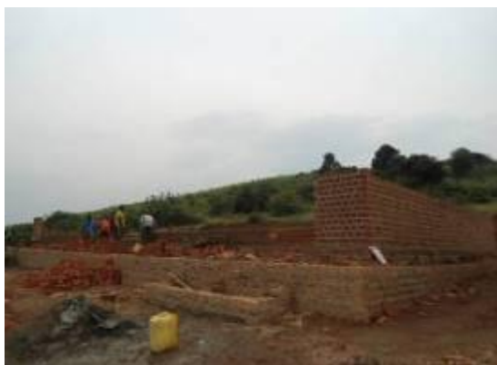
Construction of the multipurpose hall ongoing at Kifamba Comprehensive S.S. in Rakai district
