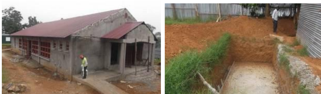
L-R: Conference facility and excavated pit still under construction at Mbazardi Mbarara district
