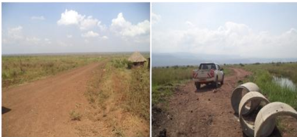
L-R: Opened 4.5 km of access road into Plots 93, 943 and 10; Culverts yet to be placed on gravel road in swampy area in Bulambuli district
