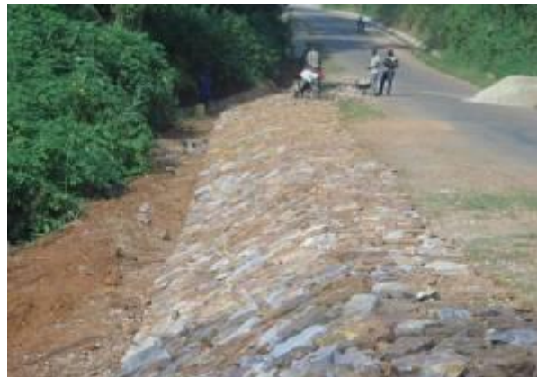
Shoulder improvement works of stone pitching along Sika Mudali – Bwanda Covent Access road – Kalungu District
