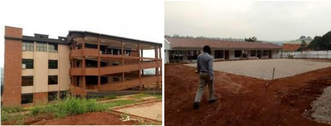
L-R: Completed Incubation Centre, and the parking yard under construction at Kyambogo University
