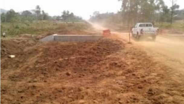
Another section at KM 6+140 with land compensation issues yet to be resolved along Bumbobi – Lwakhakha Road
