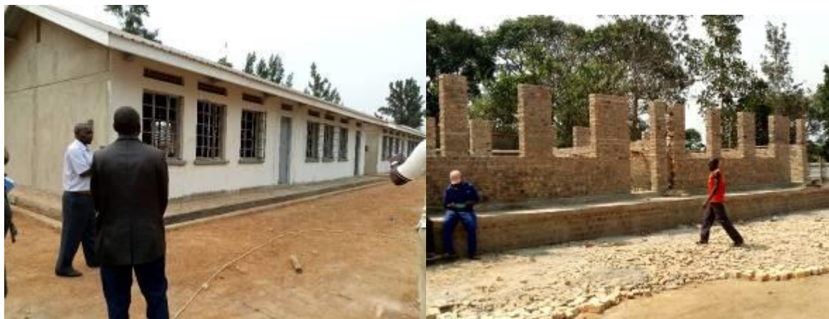
L-R: Construction of school facilities at Ishongororo P/S; Ishongororo Town Council in Ibanda District at plastering level; St. Charles Butawata P/S; Kyamulibwa SC; Kalungu District at window level
