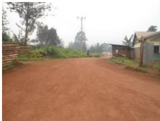
A section of Kasi Road (0.5km) in Northern Division that was graded and gravelled
