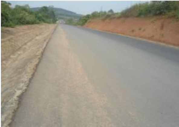
A stone pitched drain and laid asphalt layer on the carriageway at Km 2+680
