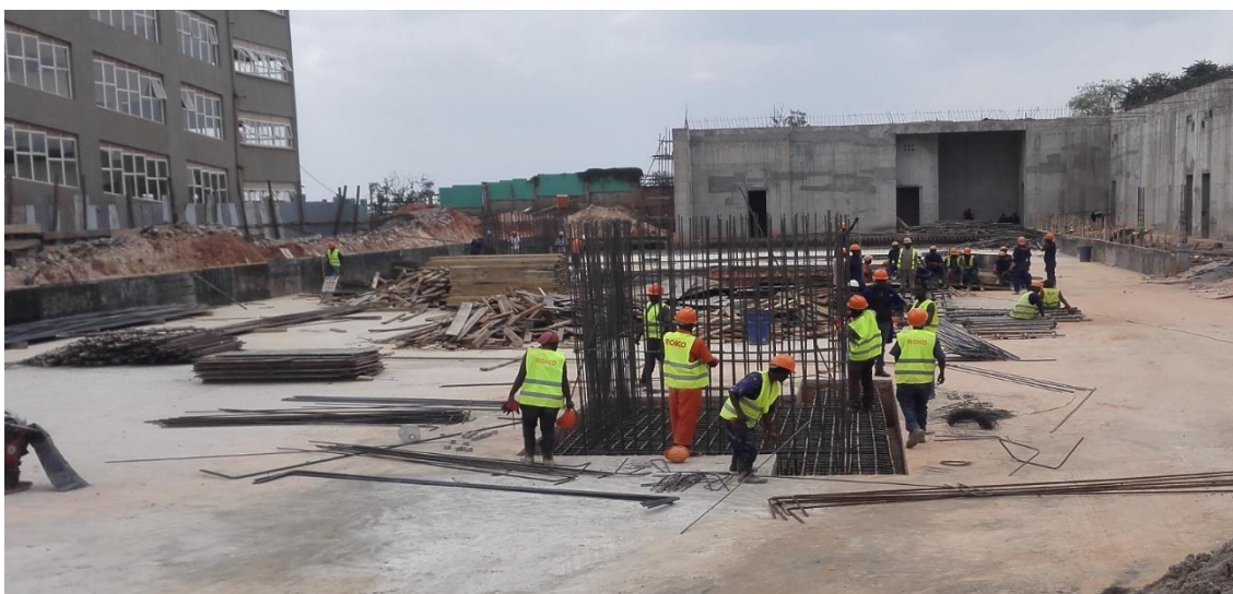
Ongoing construction works of the Auxiliary building at the Radiotherapy bunker, UCI-Mulago Hospital
