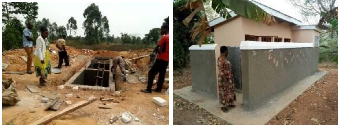
A 5 stance lined pit-latrine at underground slub in Kyankia Primary School, Kyotera District; Completed 5 stance pit latrine at Kifamba Primary School, Gomba District.
