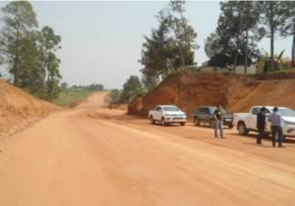
Property in the RoW obstructing works at Km 0+800 which had not been compensated on Kashenyi-Mitooma (11.53km)
