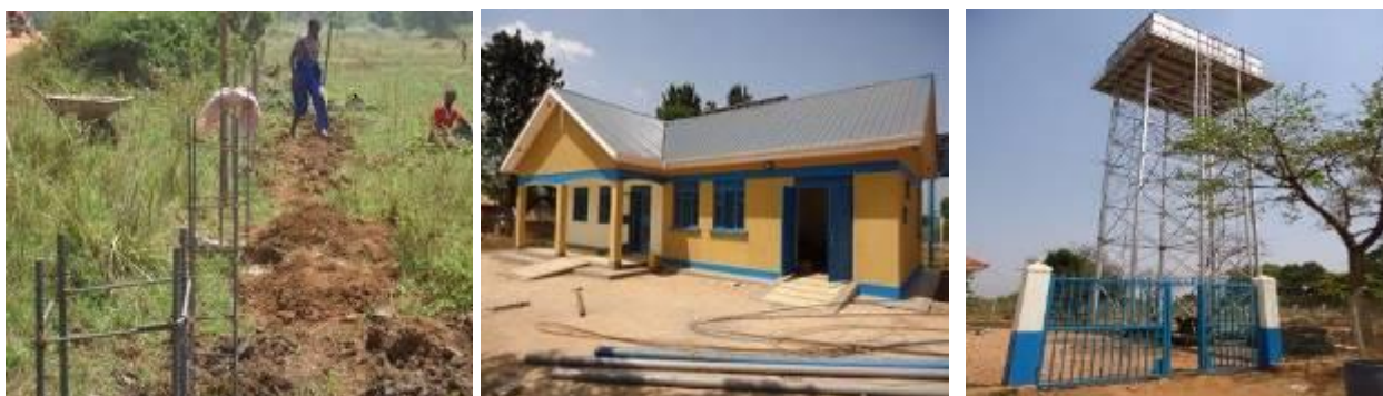
L-R: Reinforcement for anchor blocks to hold GI pipes across a swampy section; Water office; 144m 3 Reservoir tank in Buyende Town Council, Buyende District
