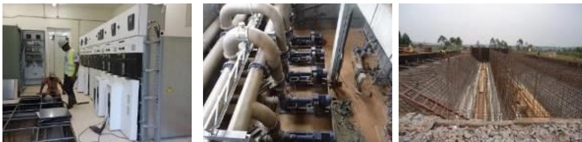
L-R: Ongoing electrical installations; Mechanical installations at the NWWTP in Bugolobi. Reinforcement steel works for the grit removal chamber at the Kinawataka pre-treatment plant
