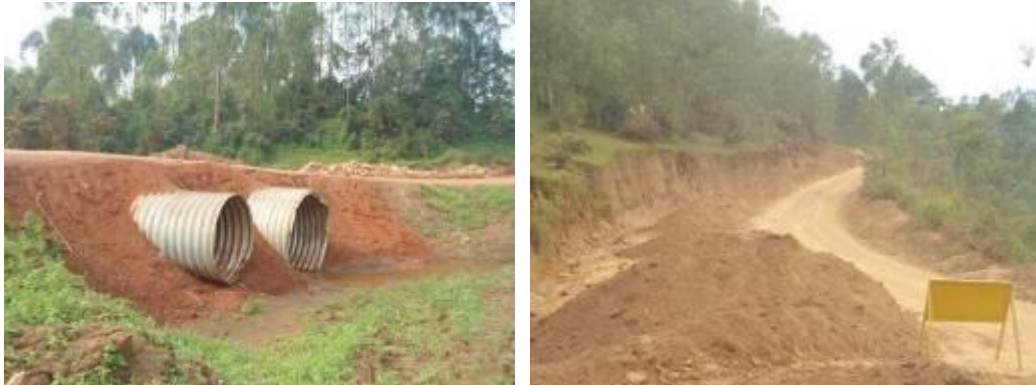
Left: Emergency works of double cell culvert installation on Butobere - Muyumbu – Rwamucucu (18.2km); Right: Dumped heaps of gravel at Km 4+00 on Rukungiri - Ruhinda (20km)
