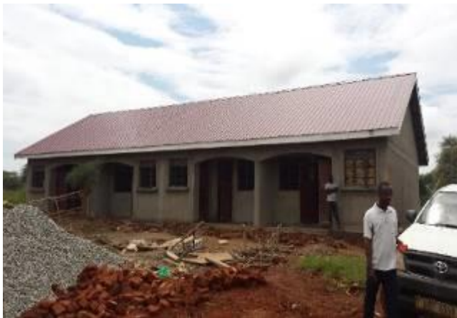
A four unit staff house at Loroo Primary School in Loroo sub-county, Amudat District
