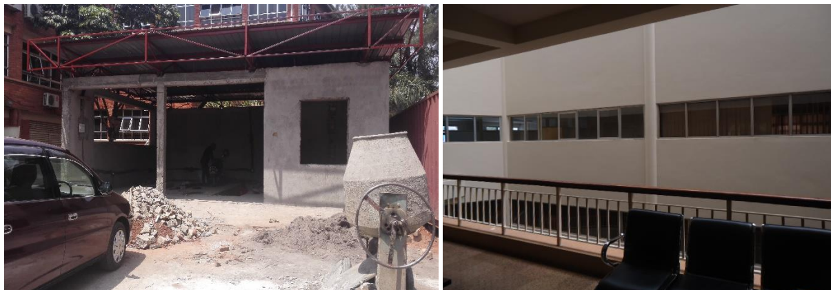
L-R: Service garage under construction and improved 3 rd floor of the MoH (initially affected by fire in 2017)
