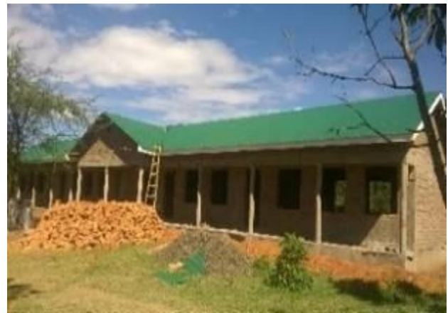
A three classroom block at Kamaturu Primary School in Lorengedwat sub-county, Nakapiripirit District
