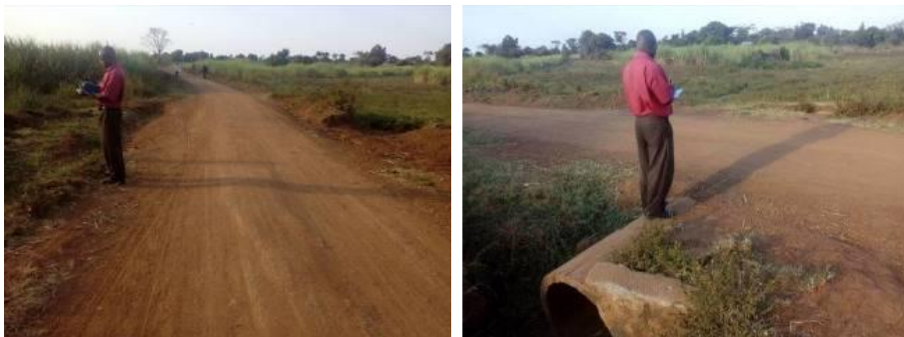
A graded section (L) and an exposed culvert (R) along Ndalike-Bugaya road in Buyende District
