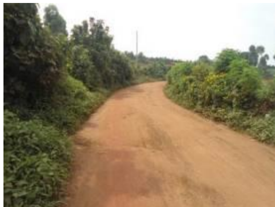
A section of Kachwekana-Rubinga-Kibuzigire Road at Km 4+800 where potholes were developing on the road and routine manual maintenance works were not done
