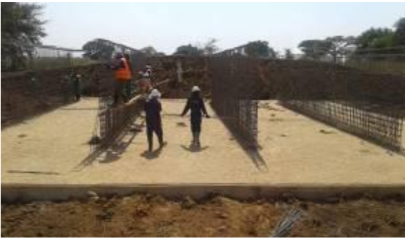
Finished foundation and reinforcement works for the Lopei Bridge along Moroto – Kotido Road
