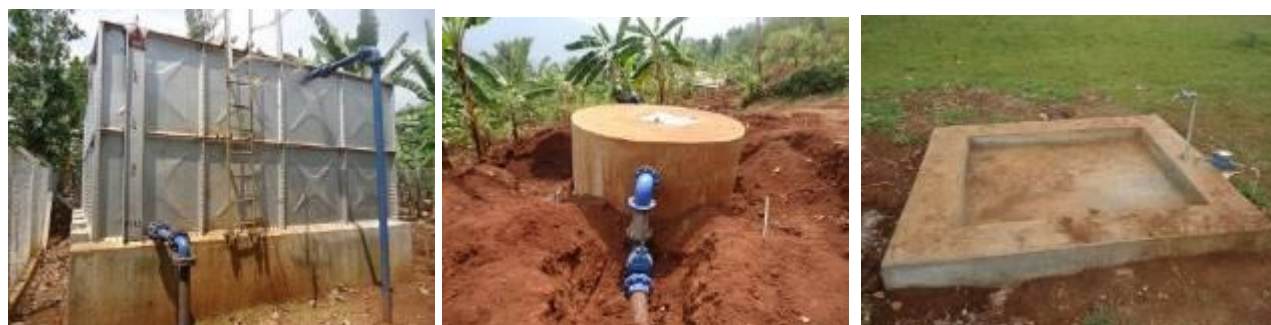
L-R: 50m 3 reservoir tank at Nabweya sub-county; 2.5m 3 BPT at Bulukyeke sub-county; Yard tap at Bulukyeke sub-county headquarters in Bududa District
