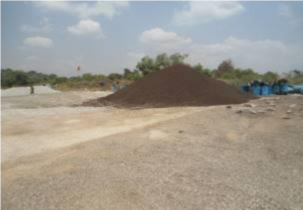
Pre-coated aggregates to be used for the surface layers on Rushere-Nshwerenkye (11.1 km)
