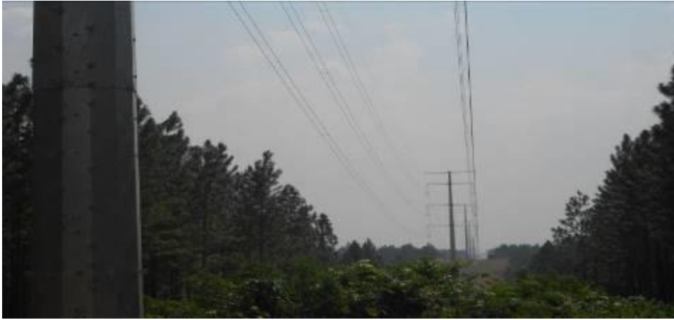
Completed section of Monopole towers on the Hoima-Nkenda Transmission Line in Hoima District
