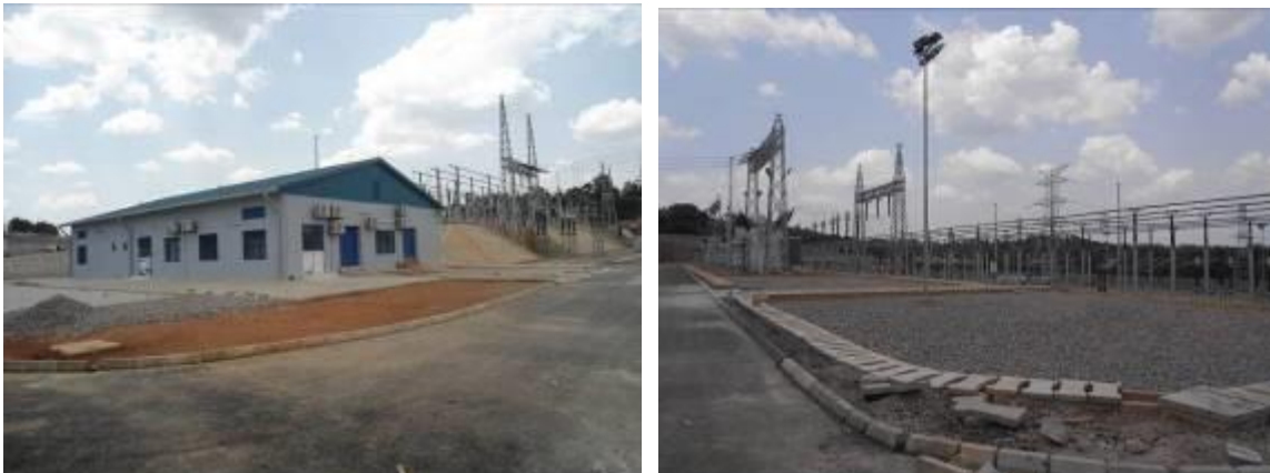
L-R: Completed plant house; Partially completed switchyard in zone 3 at Masaka substation
