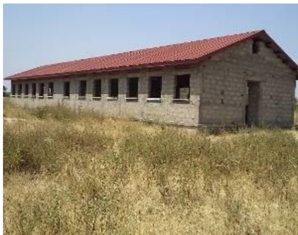
Rollover project of girls' dormitory at Lolachat Primary School in Nakapiripit District
