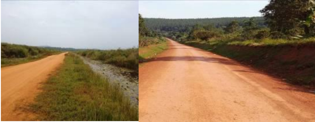
A swamp crossing at km 13+000 where river training was done along the Kayabwe-Nkozi-Kabulasoke Road (42km)
