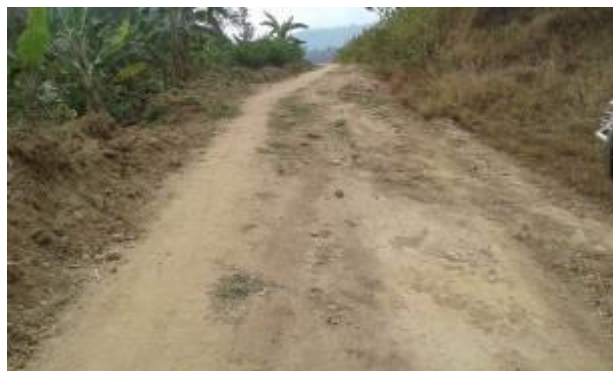
A graded section along the Nakiwandye – Bugibuni Road with grass already growing due to lack of gravel
