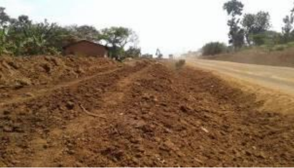
A house yet to be compensated within the RoW along Bumbobi – Lwakhakha Road at Km13
