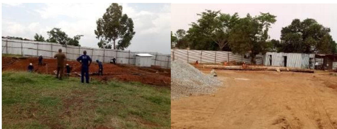
Kbisi Rusozi; Kaliro sub-county; Lyantonde District at ground excavation; Magoma Orthodox P/S; Kikamulo P/S in Nakaseke District at slab level
