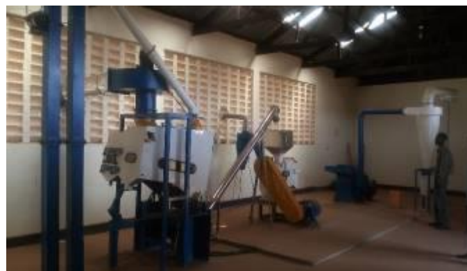
Installed maize mill machinery but non-functional in Siduka sub-county, Busia District
