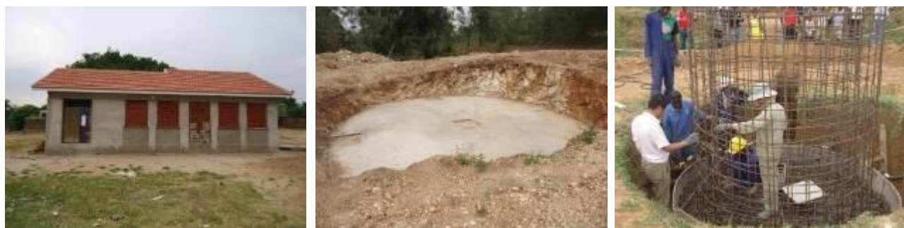
L-R: Water office; Foundation (blinding level) of 119m 3 water tank at Sibanga Sub-county; Ongoing construction of BPT at Butiru Town Council, Manafwa District
