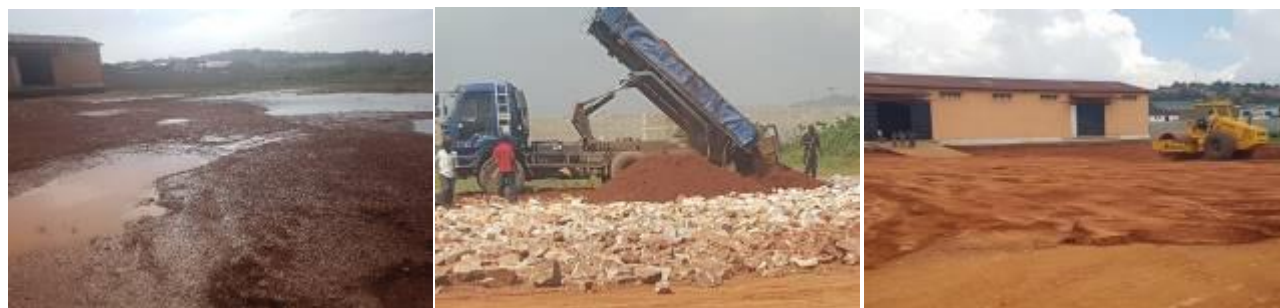
L-R: Parking yard at Namanve stores; Pouring of hard core and murrum at the park yard; Levelled park yard at Namanve stores
