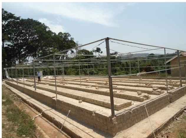
The screen house that was pulled down due to shoddy works at NACORI Mukono District
