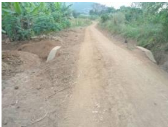
A road section of Kagorogoro Road at 0+500 with a culvert of 600mm diameter installed
