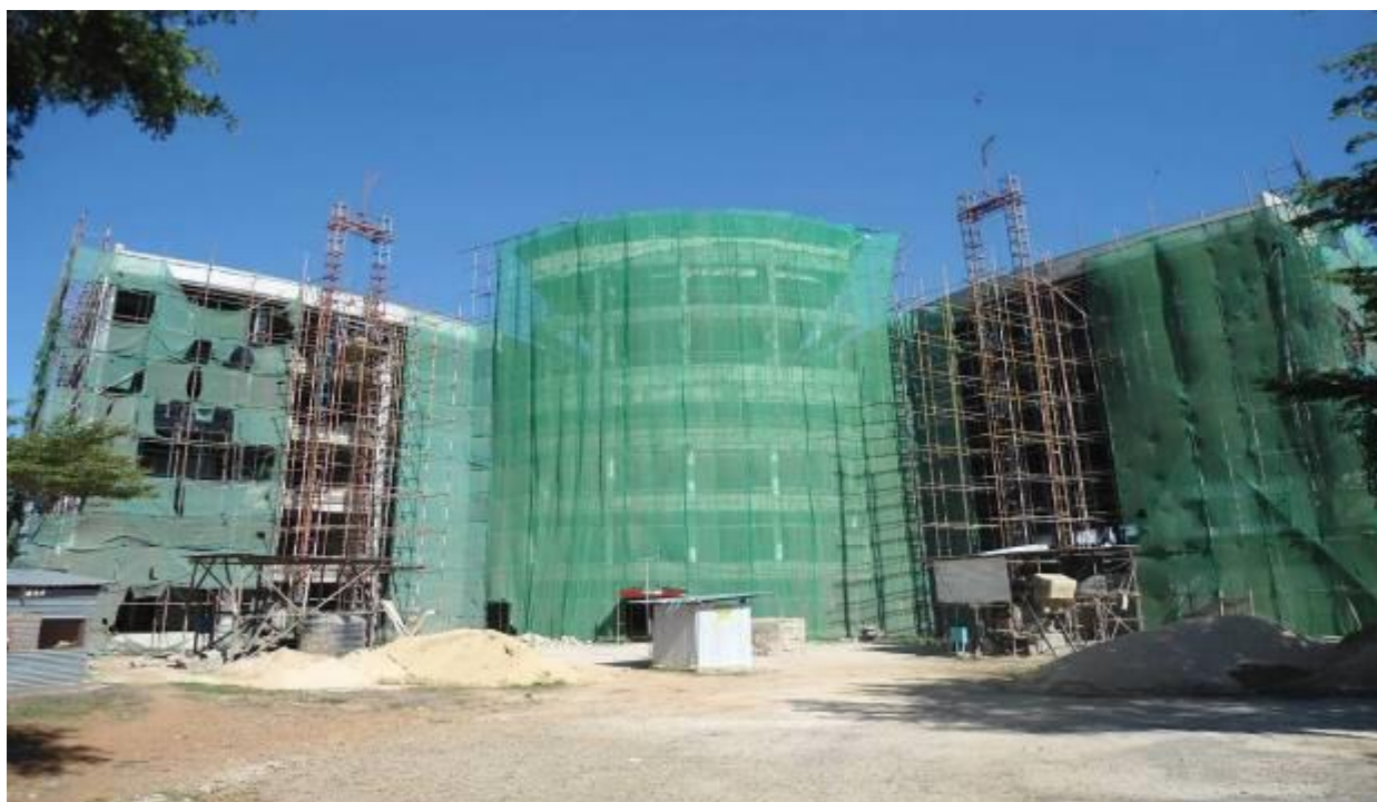
On-going finishing works on phase 3 of the new Petroleum Directorate building in Entebbe
