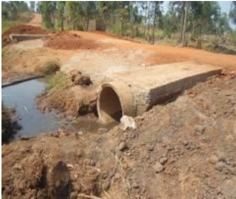
Two lines of culverts of 900mm encased in concrete at km8+100 along Kigoroby-Buseruka Road
