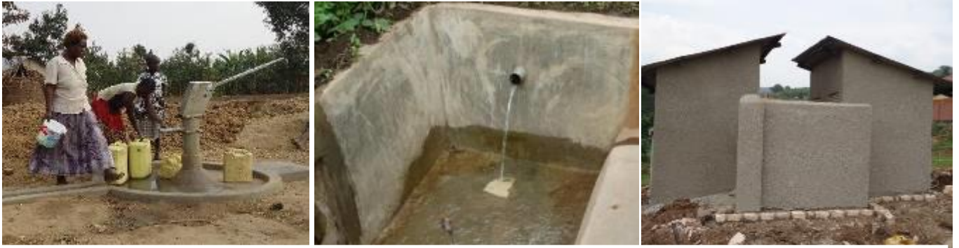
L-R: New borehole in Namukalo village, Tademeri sub-county (Budaka District); New Spring in Nyakakiri village, Rwegwe sub-county and contracted water borne toilet at the district headquarters (Rukungiri District)
