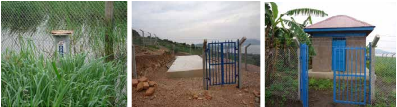
L-R: Production borehole; Pump house; and Reservoir tank base of Ntovu Small Scale Irrigation Scheme in Rakai District
