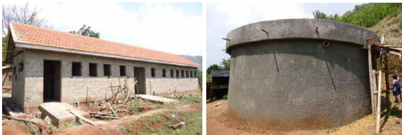
L: 22 stance water borne toilet; and R: Busuku concrete reservoir tank of Lirima II WSS in Manafwa District
