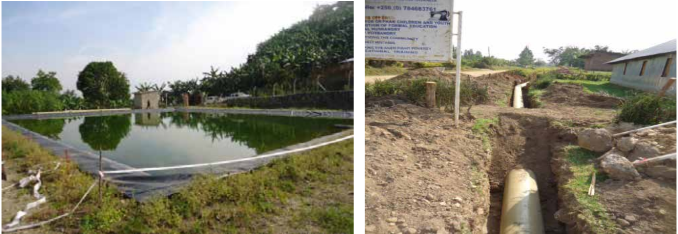
L-R: Storage reservoir at the source; and a section of the transmission main pipeline of Rwengaaaju Irrigation Scheme in Kabarole District
