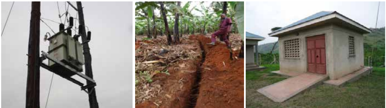
L: Transformer at the pump station; C: Excavation for the intensification lines; and R: Terrazzo flooring at the pump house of Nyamiyonga-Katojo WSS in Isingiro District
