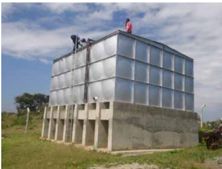
A reservoir tank of Binyiny Water Supply System in Kween District
