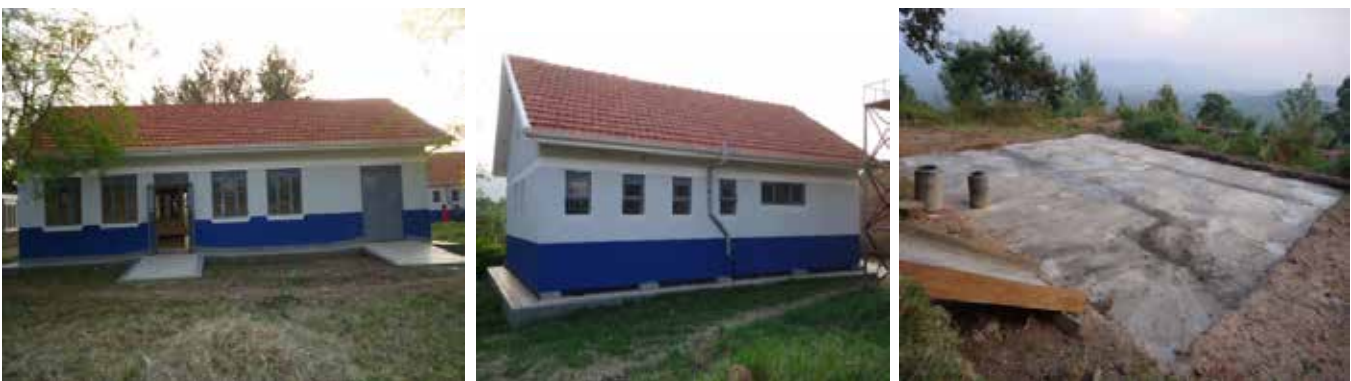
L: Water office; C: Public water borne toilet; and R: Blinding at the reservoir tank site of Kabuyanda WSS in Isingiro District
