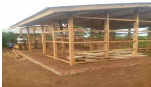
The structure for briquette machine constructed by Busheeka Briquette Making Group in Kikagata Sub-county, Isingiro District
