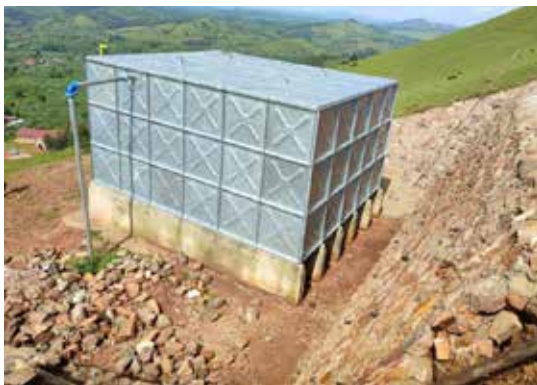
Rwabiko reservoir tank Ntungamo District
