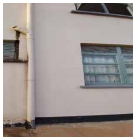
A leaking sewer pipe flowing with fecal matter at the newly constructed male hostel at UTC-Lira
