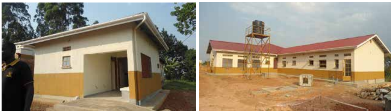
L-R: Progress of works at the General/maternity ward and standalone laboratory at Rutete HCIII Kabarole District under Lot 4
