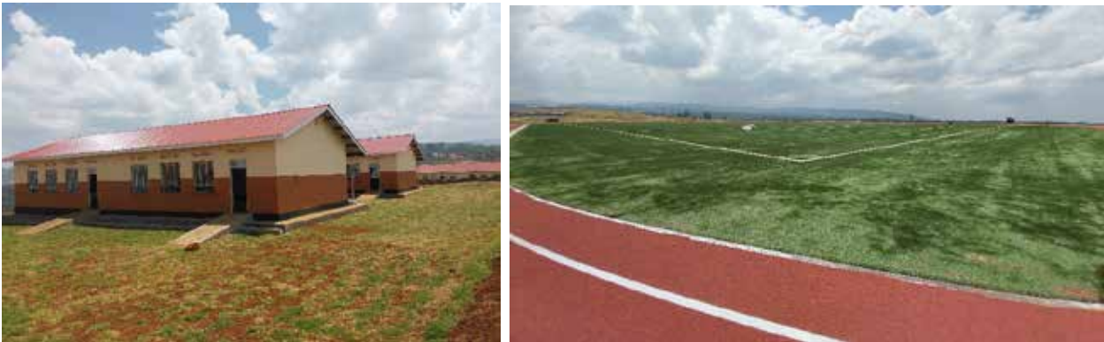
Left: Completed artificial turf field with soak pads and artificial grass; Right: Some of the Completed classrooms at Teyret Seed Secondary School in Kapchorwa District
