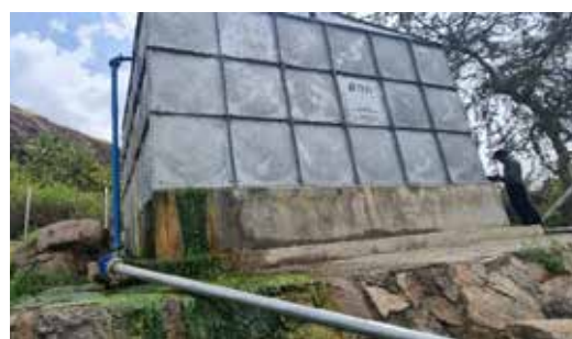
Leaking tank of Kagulu WSS in Buyende District
