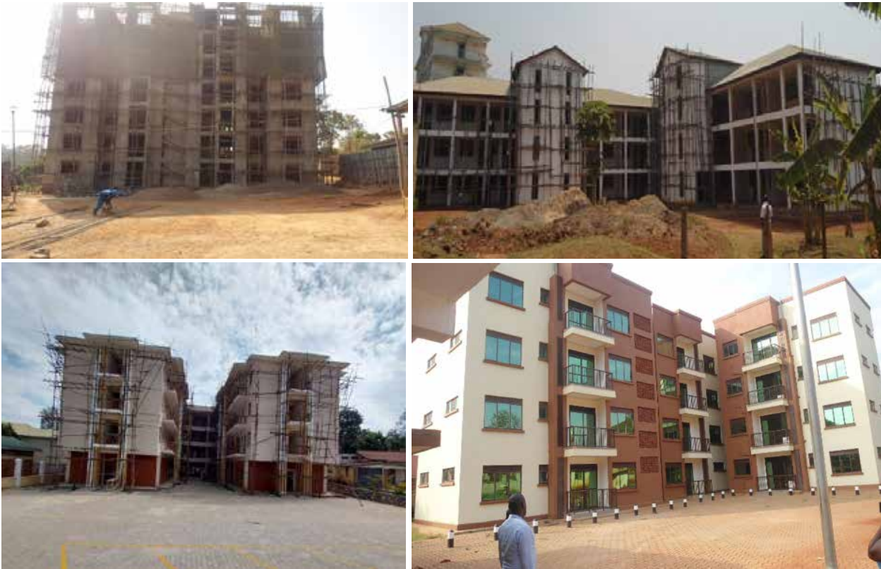
Clockwise: Ongoing staff house construction works at Arua RRH, Gulu RRH, completed intern’s hostel Kabale RRH, and completed staff house at Jinja RRH
