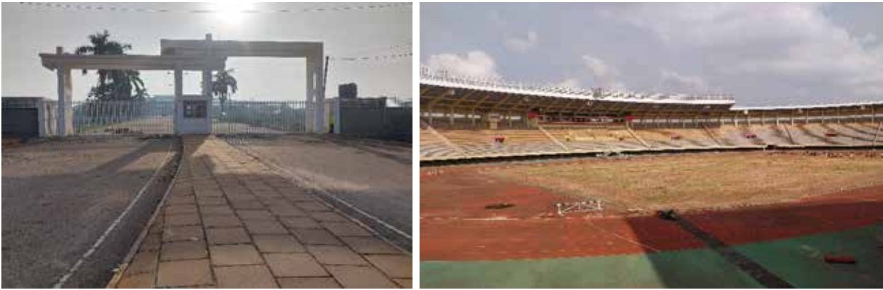
Left-Right: Ongoing upgrading and renovation; Completed front gate at Mandela National Stadium, Namboole
