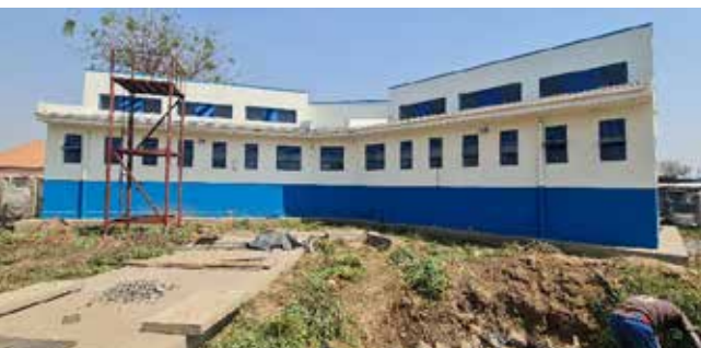
A 14-stance Water Borne Toilet at Elegu Border, Amuru District
