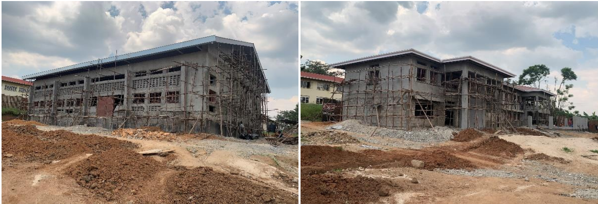
Left: A multi-purpose hall at 58% progress Right: A girls' dormitory at 63% progress at Lwengo TI. The site was behind schedule
