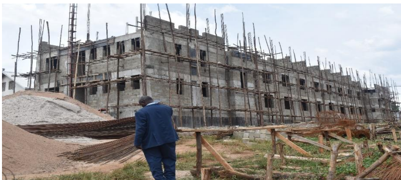
The ongoing construction of the girls' dormitory at Hoima School of Nursing and Midwifery
