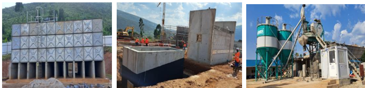
L-R: 2500m 3 at Kajaro; intake, inflow, and grit removal chambers; Concrete batching plant
