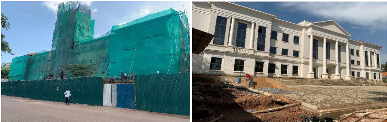
Left-Right: Ongoing construction works for the Makerere University Main Building at 44% progress; Right: Front side of the Makerere University School of Law building nearing completion at 95%
