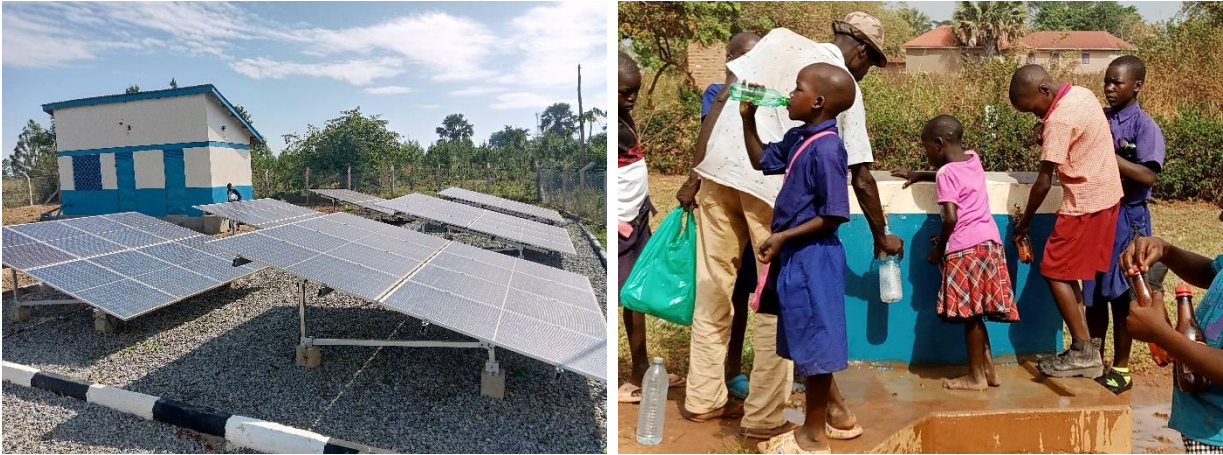
L-R: A pump house and solar array; A Public Stand Post for Awaldek solar powered water system in Nambieso Sub-county, Kwania District
