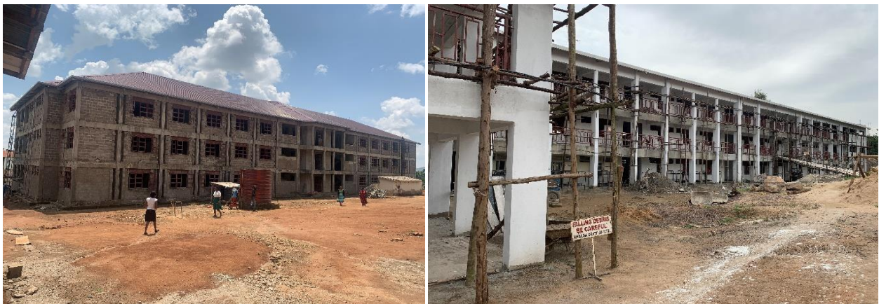
Left: Ongoing construction of the girls' dormitory at Tororo Girls in Tororo District at 83% progress; Right: The 480-bed boys' dormitory at Ntare Senior Secondary School at 80%, Mbarara District under Development of Secondary Education Phase II
