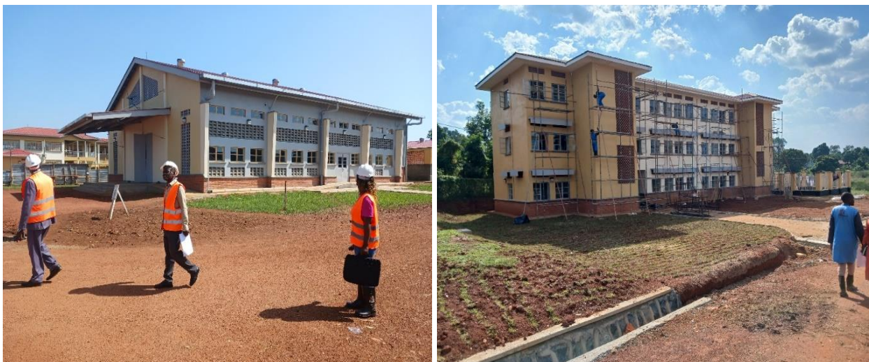
Left: A multipurpose hall at 92% progress, Nawanyago Technical Institute in Kamuli; Right: Renovation of the boy's dormitory at 95% progress, Basoga Nsadhu Technical Institute, Namutumba District
