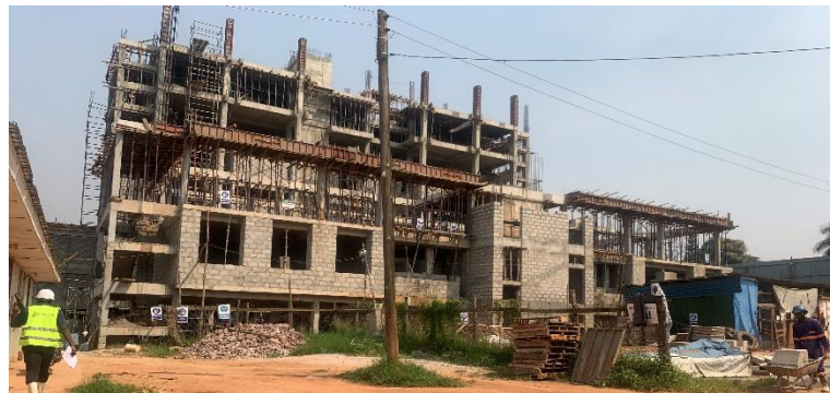
The ongoing construction of the five-storey UBTEB Assessment Centre in Kyambogo at 32% progress
