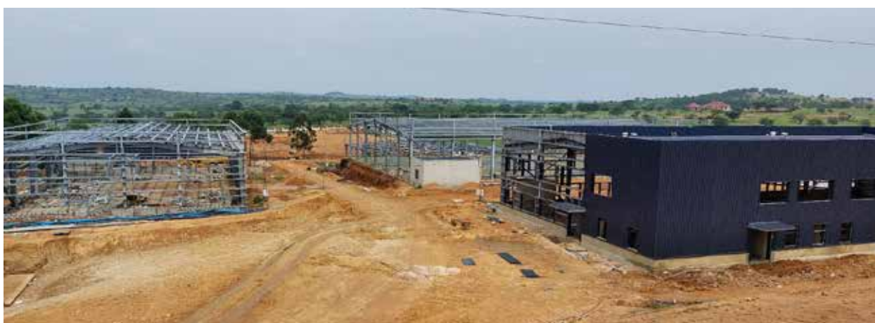
Top to bottom: Completed and equipped heavy duty machinery workshop at TIBIC in Namanve and ongoing construction of training workshops at NSTEIC in Rwebiteete in Kiruhura District
