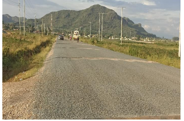
A section along Busia-Malabo Road at Km 17+312 with the 1 st seal works of DBST
