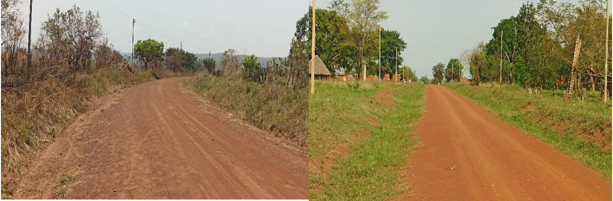
Palabek-Atiak Road: A well-graded motorable section under framework contract at Km 30+00 with overgrown grass on the roadside
