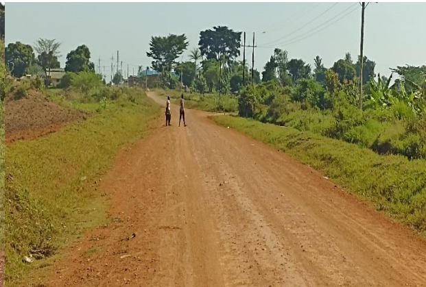
Jinja UNRA: A section in good condition at Km 21+200 near Namwiwa TC along Kaliro-Namwiwa Road – Contract by Tegeka Ent. Ltd
