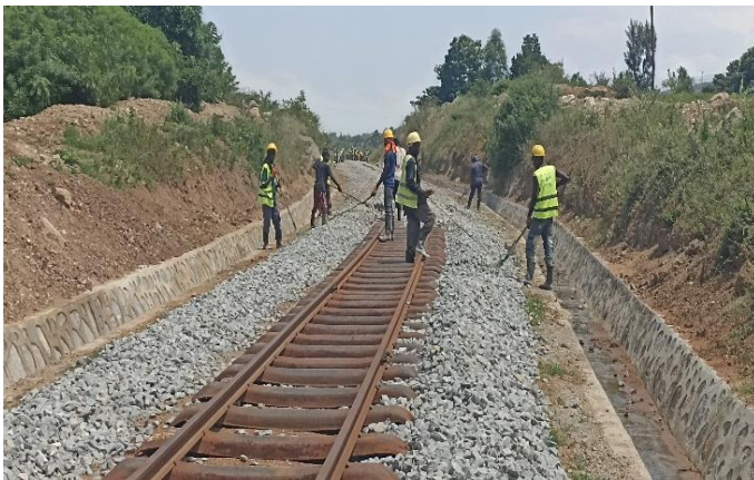
Completed storm drainage stone pitching works and laying of the rail track at Km 23+100
