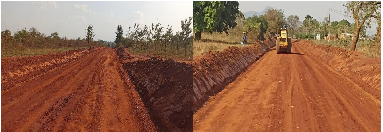
Padibe-Paloga-Madioppe: Road section in Lamwo District under Framework Contract: Ongoing works of grading and shaping at Km 5+000
