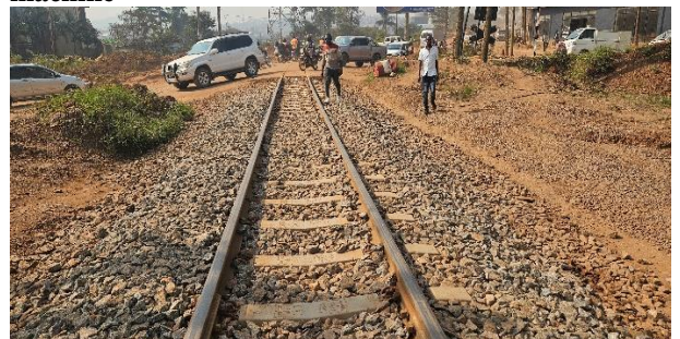
Pedestrians walking along the completed track which contaminates the ballast
