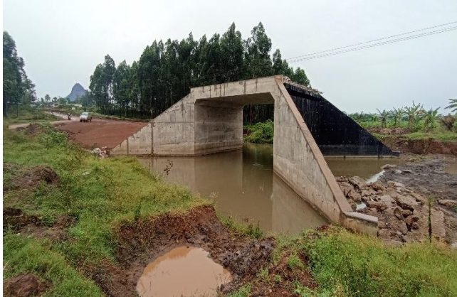
Completed 12m span Rubongi bridge structure along the Nagongera-Tororo Road in Tororo Municipality with pending works on the approaches
