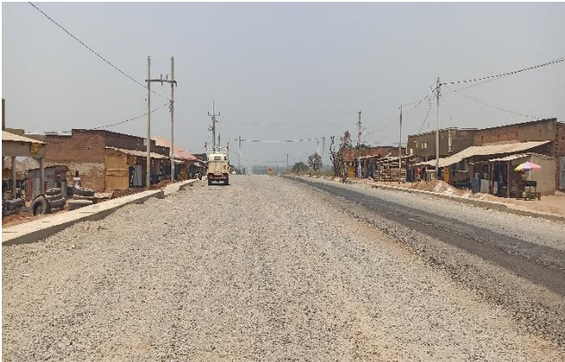
Agum Town Council section at Km 44+266 with covered side drains and unprocessed subbase along Olwiyo-Packwach Road
