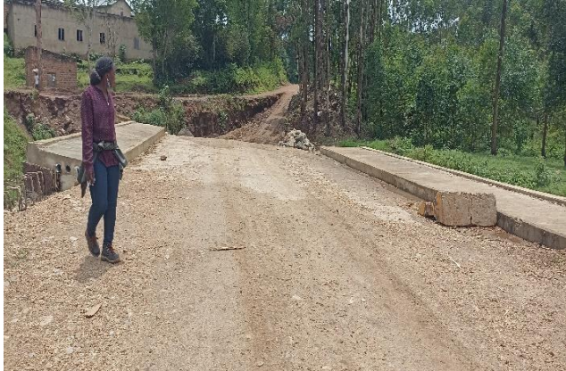
Completed 12m Khamitsaru bridge structure along the Kufu-Magale Road in Namisindwa district with pending approach road works
