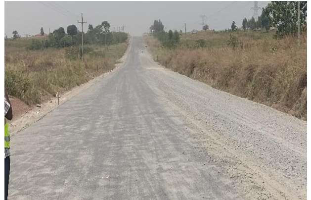
Primed section on the LHS between Km 47+100 to 48+600 of Olwiyo-Packwach Road
