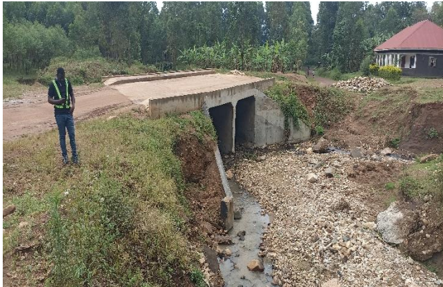
Completed 3m by 2.5m skewed Nambola double cell box culvert along the Kufu-Magale Road in Namisindwa District
