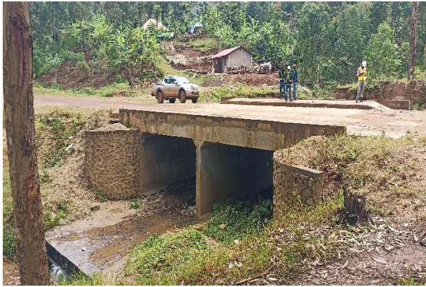
Completed 11m span by 10.6 m width Namisere bridge structure along the Kufu-Magale Road in Namisindwa District
