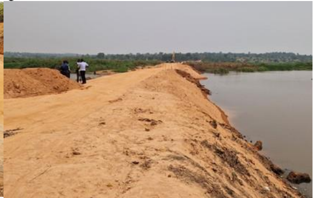
Hoima UNRA Station: Emergency works across Mpongo swamp along Kyenda-Mpong-Kisiita Road were done under force account
