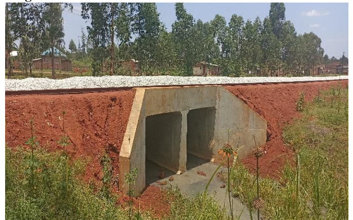
Double cell box culvert and ballasting (1 st layer of track formation) at Km 58 in Mbale Municipality
