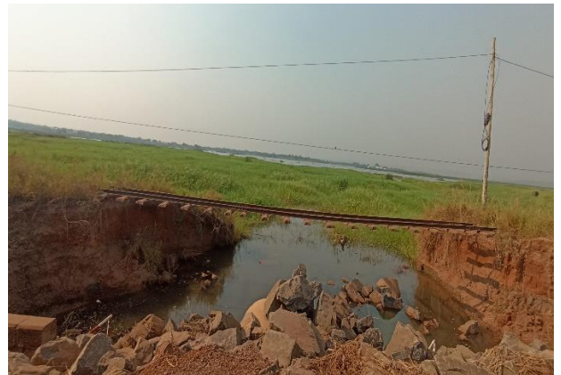
A section of Olwiyo-Packwach Road at Km 104 destroyed by the floods
