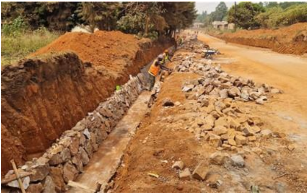
Hoima UNRA Station: Stone pitching of side drains along Katasiha-Bugambe-Mairirwe was done under a framework maintenance contract
