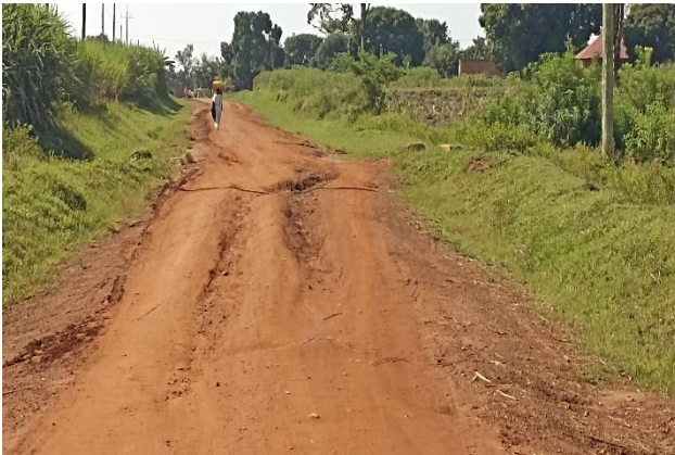
Jinja UNRA: A deteriorated section at Km 10+00 along Kaliro-Namwiwa Road – Contract by Tegeka Ent. Ltd
