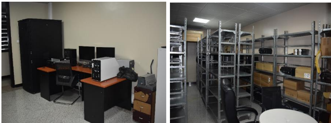
L-R: Installed ICT equipment for data storage; A view of the installed storage shelves for data tapes
