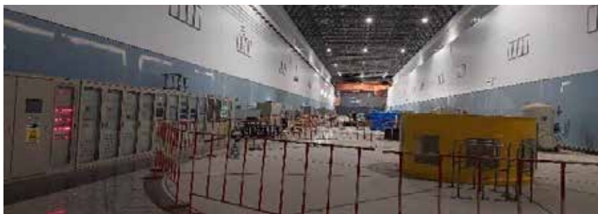
Completed electromechanical and electrical equipment installation in the Karuma HPP powerhouse
