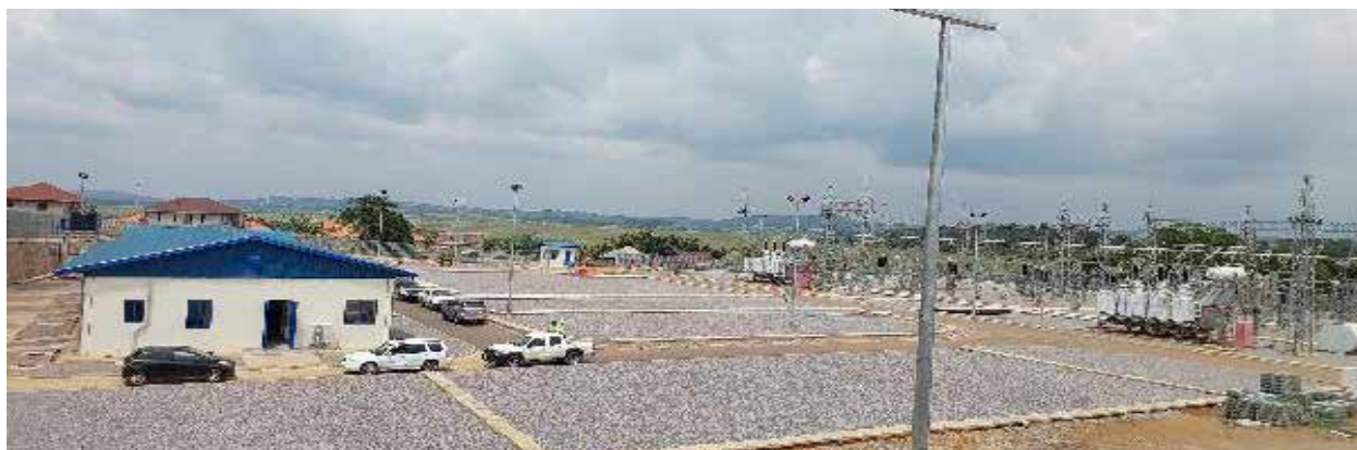
Completed Entebbe 132kV substation at Kabale in Entebbe Municipality
