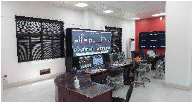
Completed central control room (CCR) for the Karuma HPP
