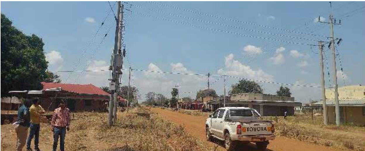
Completed grid extension at Acumet TC in Amuria District under UREAP Lot 3
