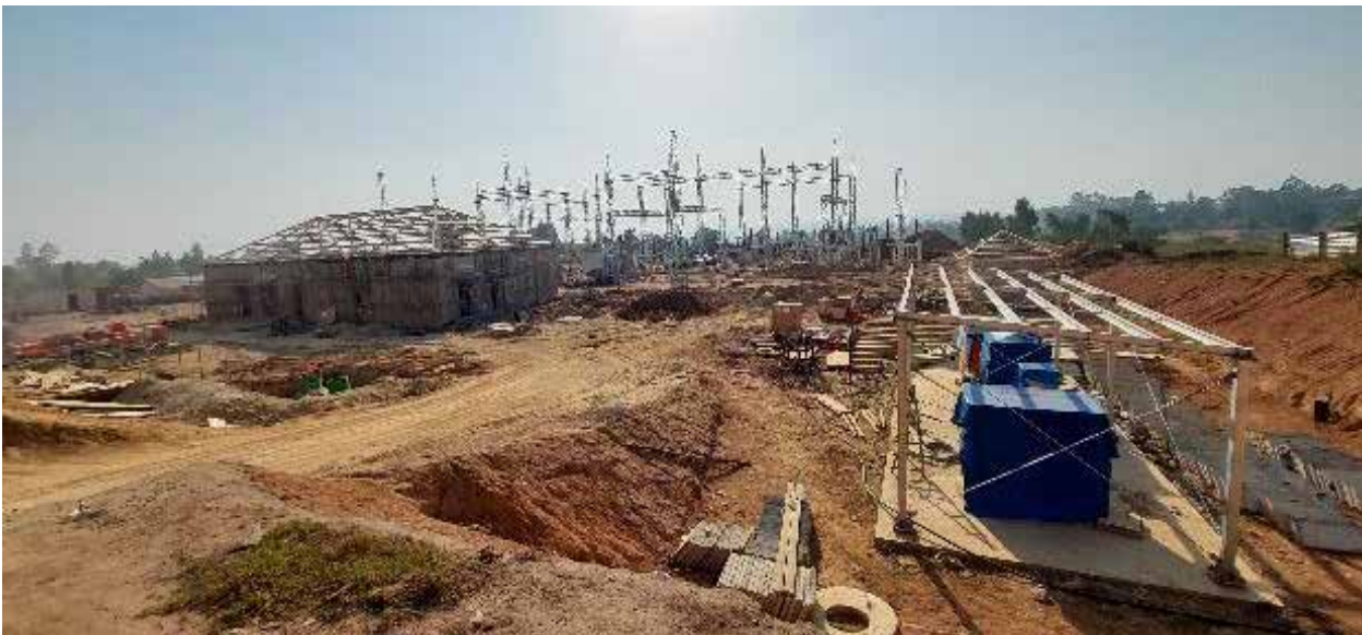
Ongoing works at the 132kV Arua substation at Muni in Arua Municipality
