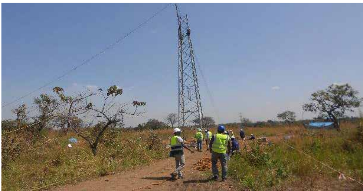
Ongoing tower construction works on the Gulu-Agago transmission project in Agago District
