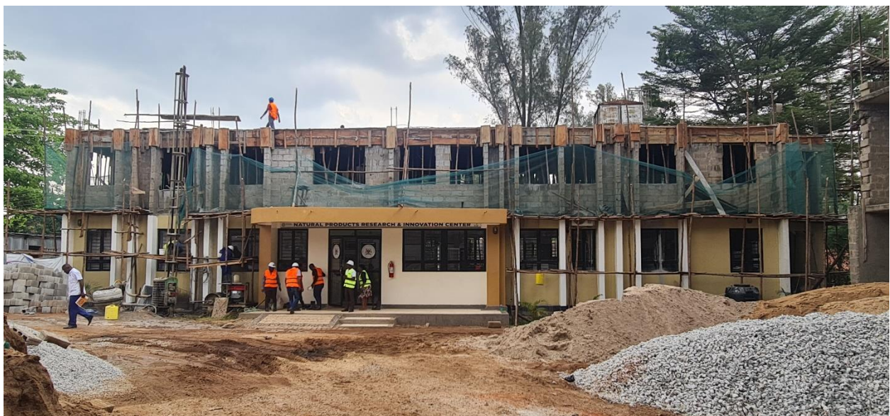
The Good Laboratories Practice facility under construction at the Busitema University Natural Products Research and Innovation Centre in Mbale District
