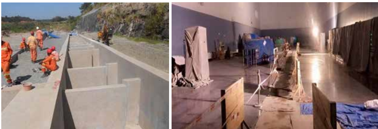
L-R: Partially complete works on the Fish Ladder; Final finishing work on the floor in the powerhouse
