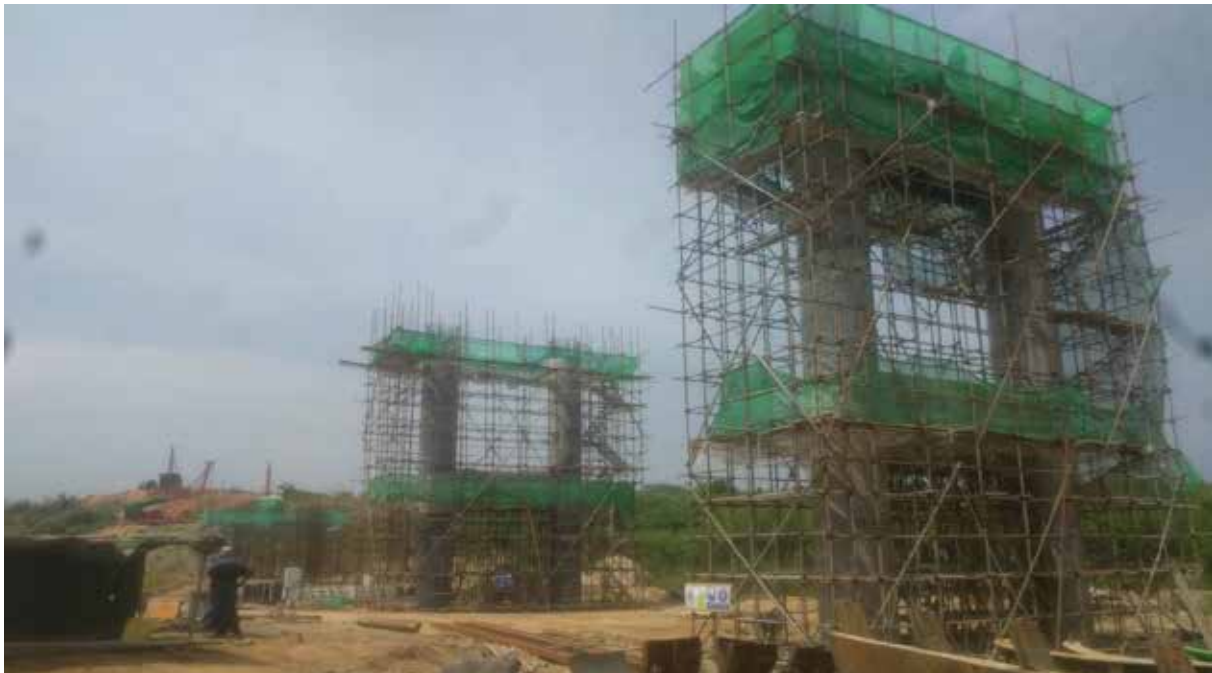
On- going civil works on the concrete support piers for the Bridge at Isimba HPP
