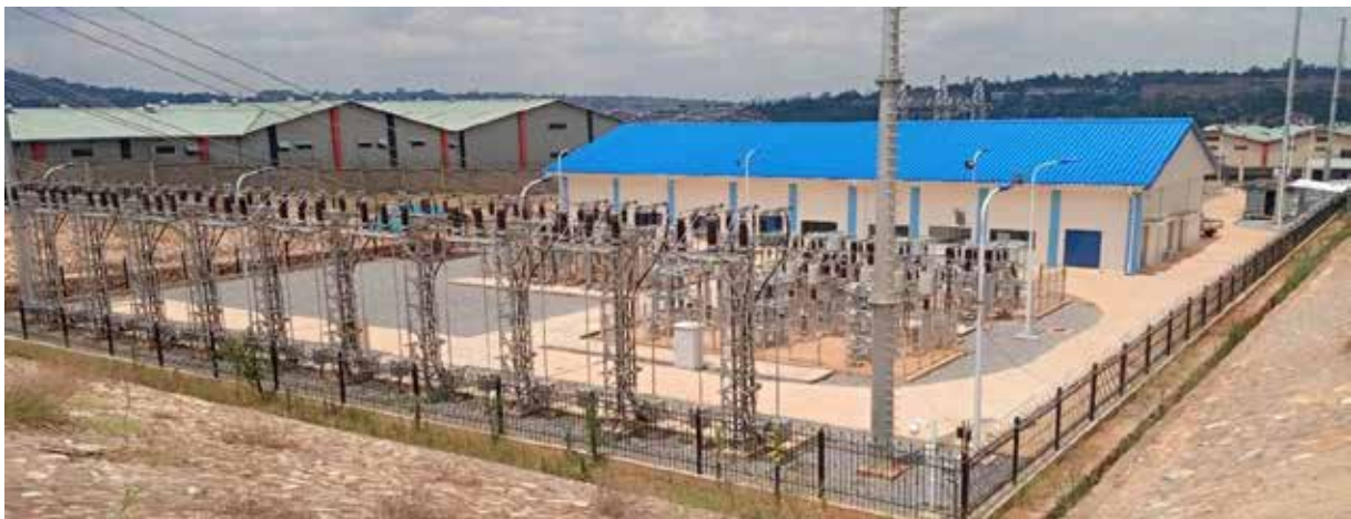
An aerial view of the plant house and outgoing 33kV feeders at the completed 132/33kV Luzira substation
