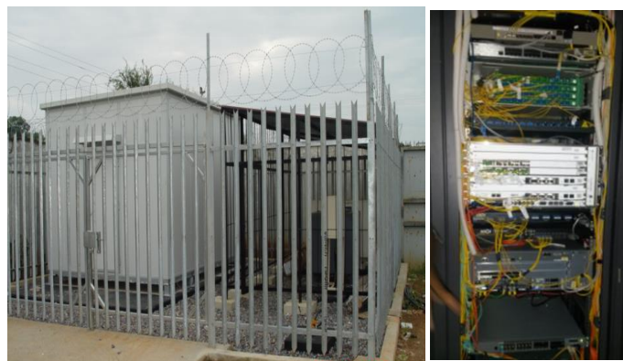
A completed NBI site in Kasese and switches mounted at the NBI Data Centre
