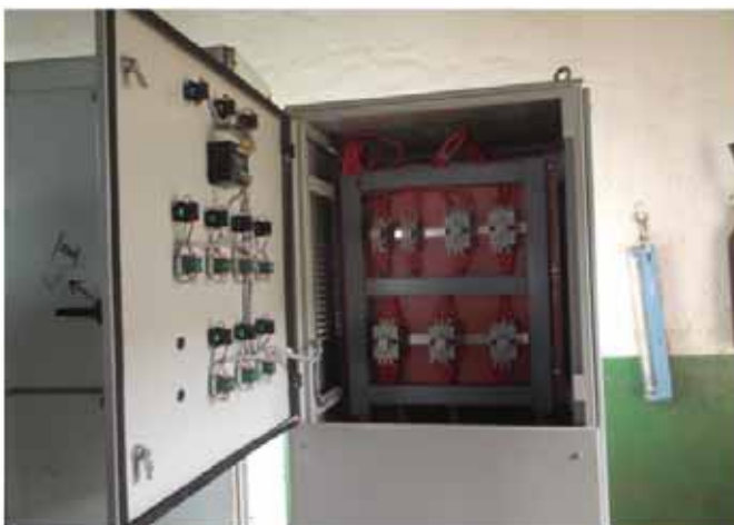
Power factor equipment installed at factory.
