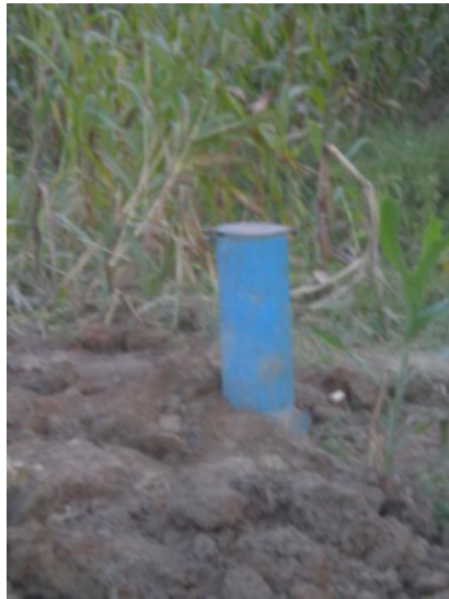
Left: Production well of Ongino water supply system in Kumi district. Works had temporarily stalled as the land owner demanded compensation
