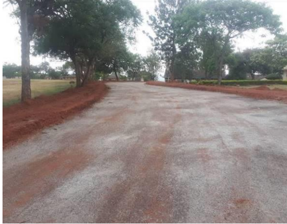
Primed section along the access road to Busoga College Mwiri in Jinja
