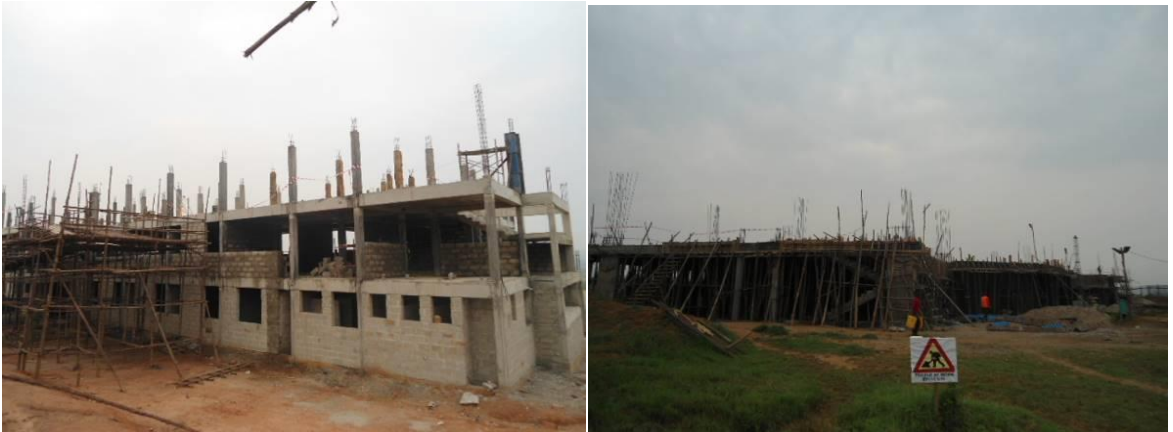
L-R: Construction of the students' hostel, and Construction of the Faculty of Computing at Mbarara University of Science and Technology
