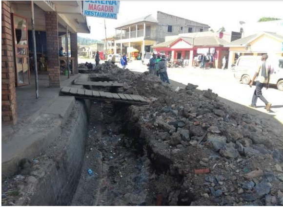
Excavation for the side drain on Bishop Kivengere road (0.3km) at Km 0+000
