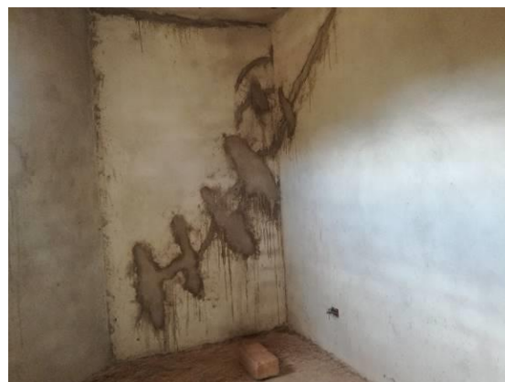
Repair work on the cracks in the walls caused by settlement at the Katuna OSBP
