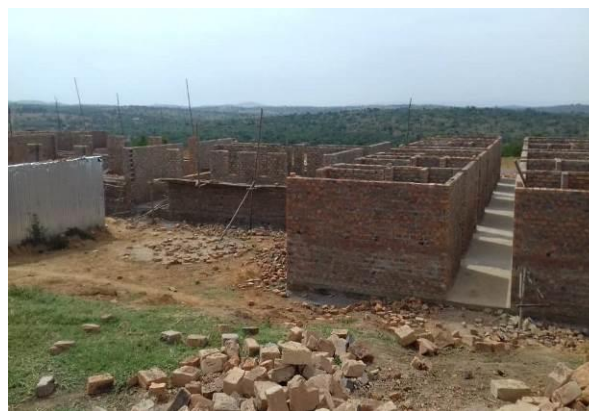
Artificial insemination staff hostel under construction at Ruhengyere Field Station in Kiruhura District
