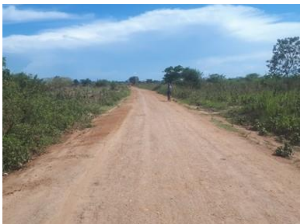
A section of Amolator-Acamulum Road (4.4km) after RMeM in Q2. The road lacks proper drainage structures
