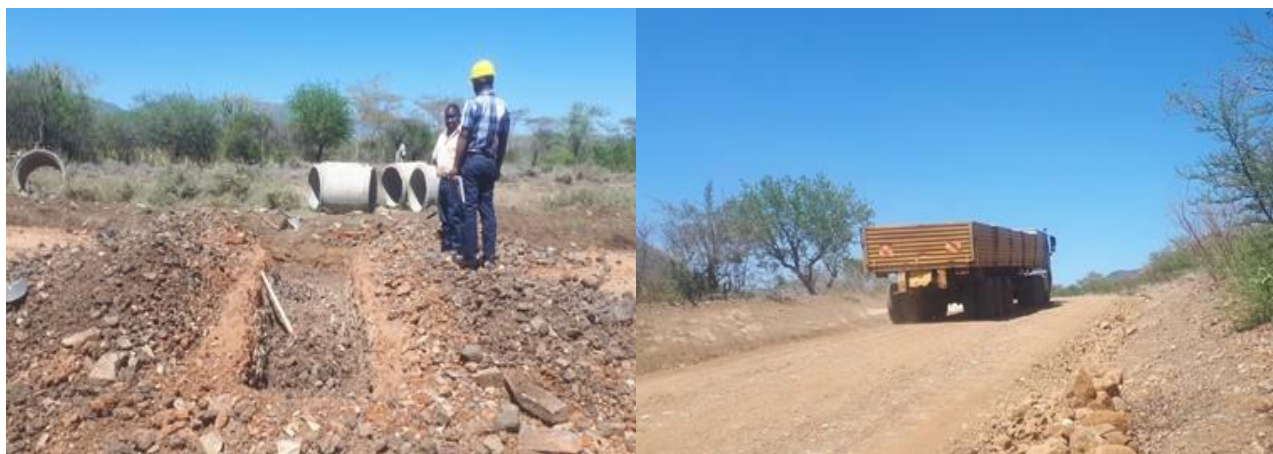
Culvert installation was ongoing along Moroto-Lokitanyala Road during the of 5 th cycle of term maintenance
