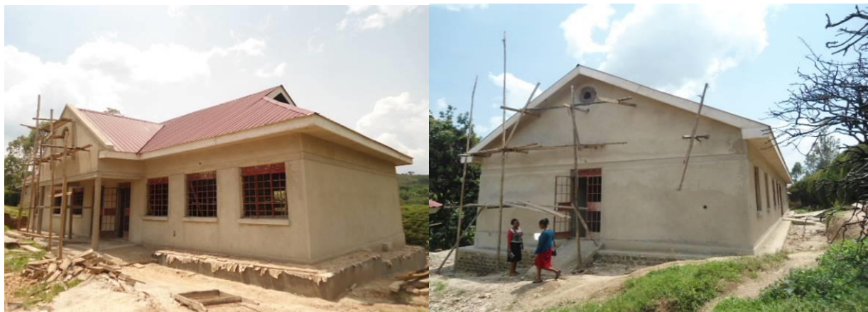
Left: Construction of an administration block at finishes level, Right: Construction of a dormitory at finishes level at Bikungu PTC, Mutara S/c, in Mitooma District
