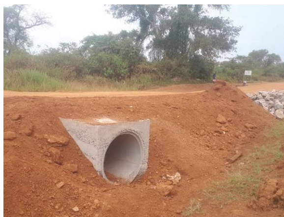
Soroti-Serere Road (27km)-900mm diameter encased culvert installed at km 22+450 in Q2 FY 2018/19; pending construction of end structures
