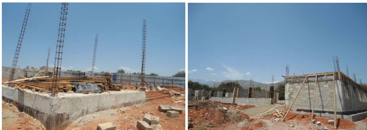
Left: Construction of BCP at sub-structural level and an Electrical Installation and Renewable Energy Workshop at ring-bim at Kasese Youth Polytechnic as at January 2019
