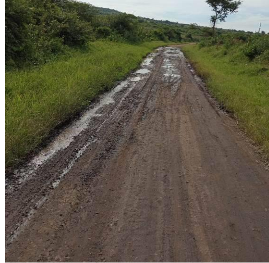
A water logged section with clayey soils on Rugaga-Rushaha-Endiizi road
