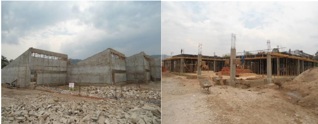
Left: Renovation of the lecture room complex at roofing stage; Right: Construction of the Library/Resource Centre at Kabale NTC as at January 2019
