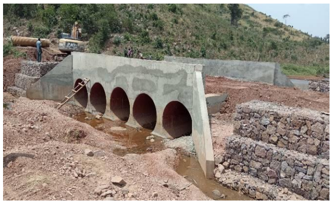
Bambala bridge: Construction of a five cell of 2.1m diameter ARMCO culvert crossing in Kyankwanzi District
