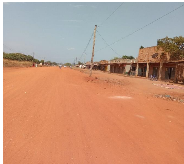
Power lines pending relocation along Bulima-Kigumbe road at km 11++000
