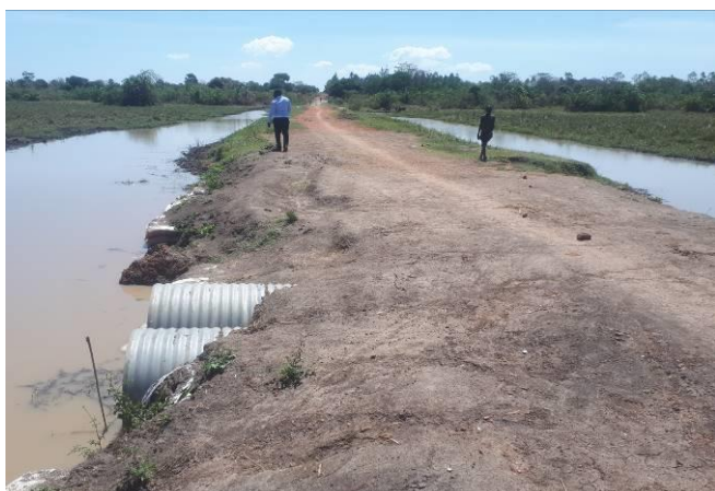
A 1.2km swamp section of Apenyoweo-Regprego road that was raised and installed Armco culverts in Q2
