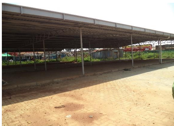
Incomplete paving works on parking area at the Nyendo market as at February 2019
