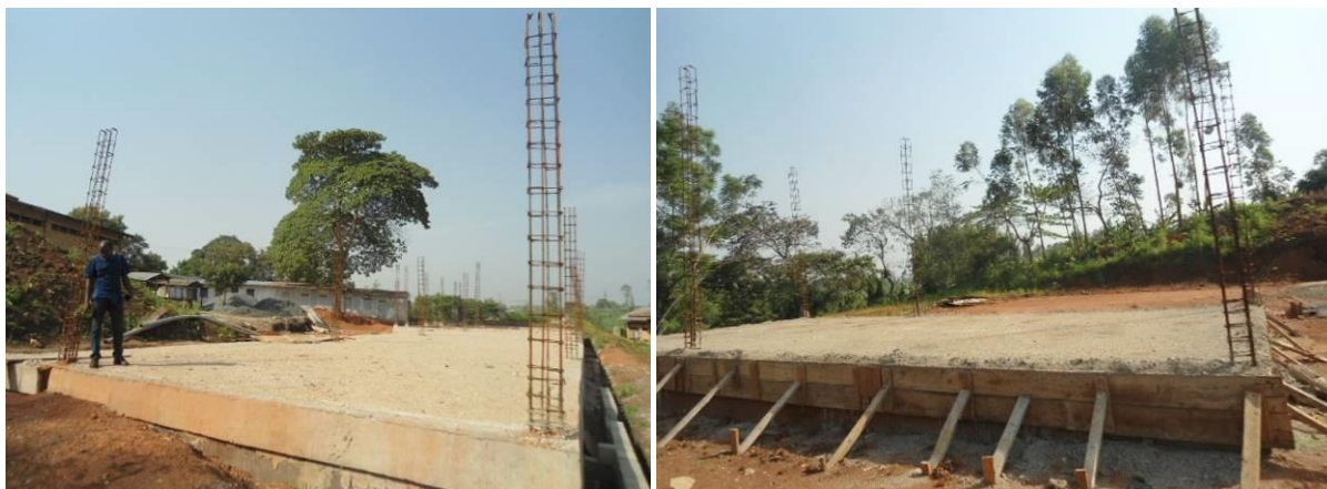
Construction of an MV workshop and a 2 classroom block at St. Joseph Virika VTI at DPL level as at January 2019
