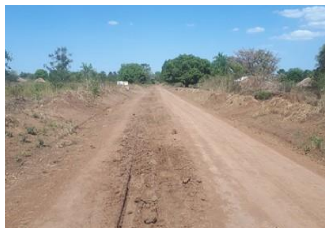
A section of Adwoki-Bata Road (10km) that had deteriorated because it was not compacted during RMeM in Q2
