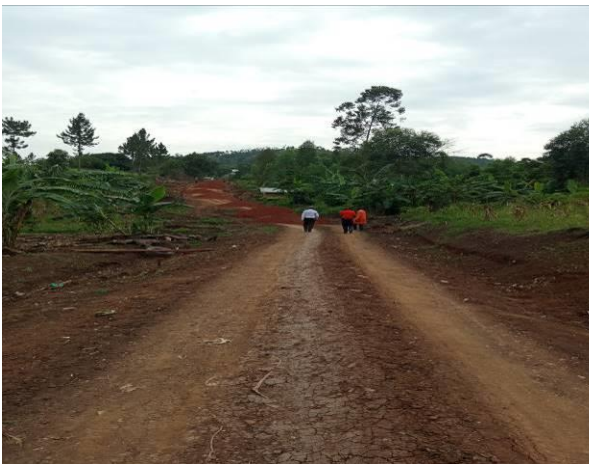
A section of Bulopa-Mpumudde road with dumped gravel
