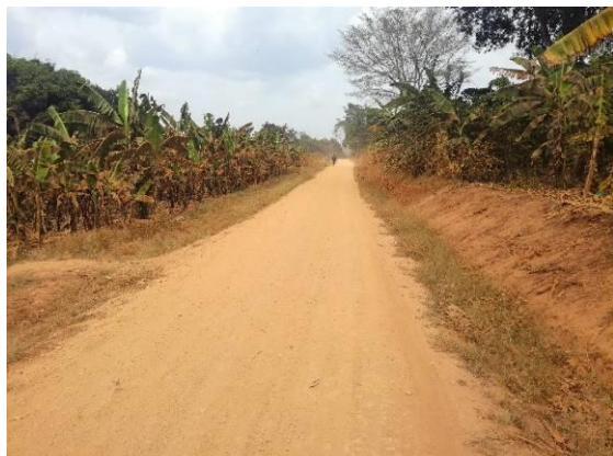
Nabutongwa-Kalungu road (3.5km): A well graded road section with over grown grass in the side drains at Km 2+800
