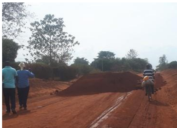
Ongoing gravelling works on Lira-Aduku-Apac road that was under mechanized maintenance using term maintenance contract
