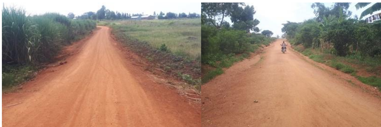
A graveled section of Bufulubi-Bukomya-Mayuge Road (6.6km) that was worked on under emergency works in Q1 & Q2 Kityerera-Kibungo Road (9.59km) that was graded under RMeM in Q2
