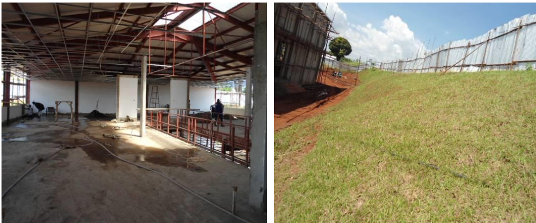
Ongoing internal works and grass planted on a side embankment at the ICT hub in Nakawa
