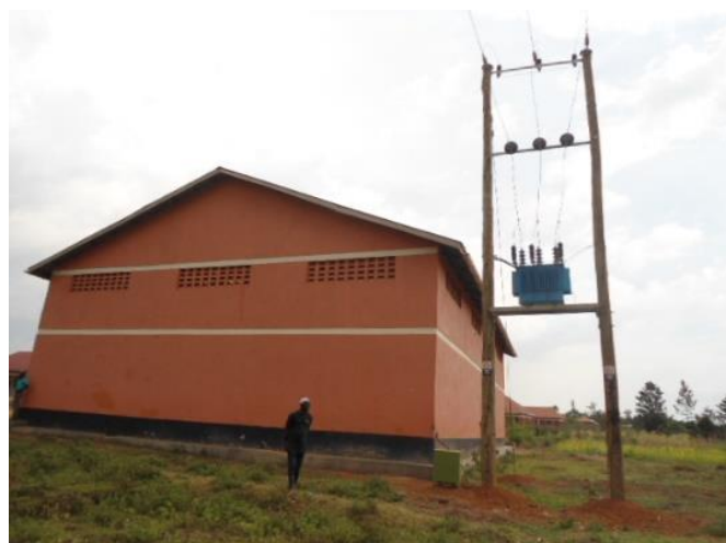
Installed 100 kva transformer in Butaleja District
