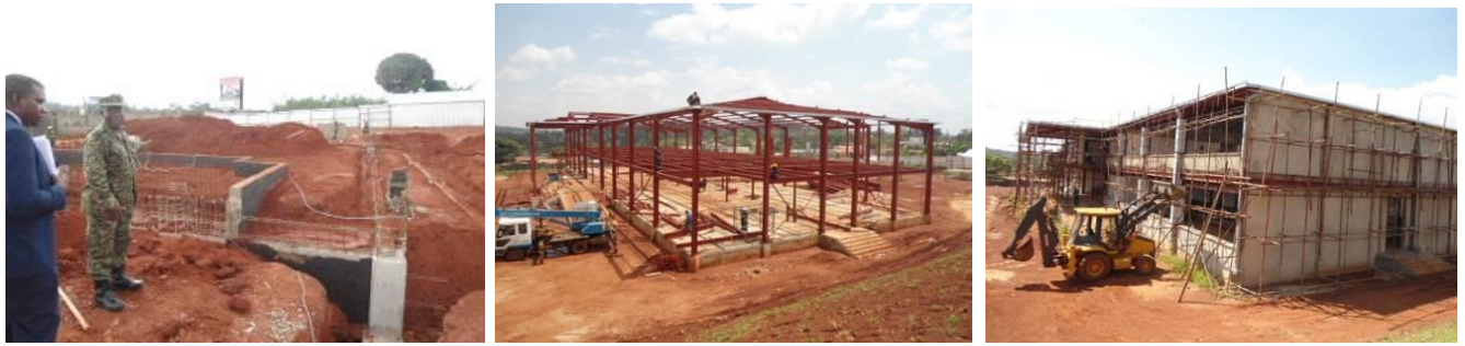
L-R: Progress on construction of the ICT Innovations Hub at Nakawa in February and July 2018; and February 2019
