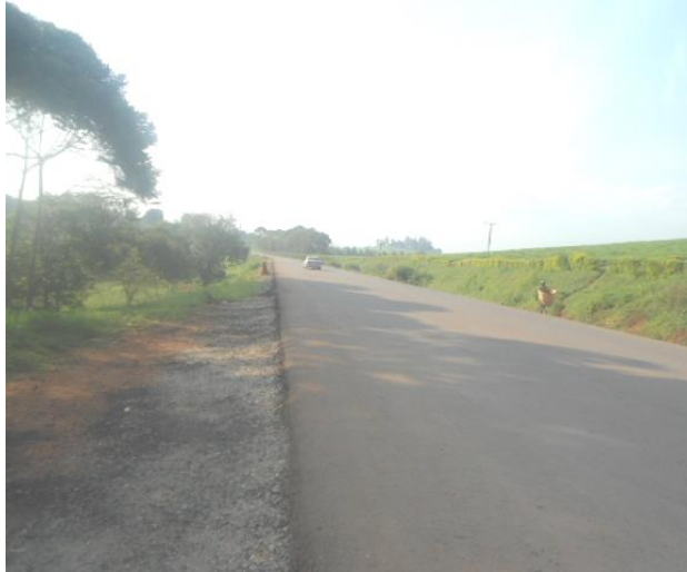
A section of laid asphaltic concrete surface at km 37+000 on Kyenjojo-Fort Portal Road
