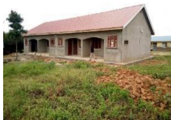
Incomplete four unit staff house at Kamaturu Primary School in Lorengedwat Sub County, Nakapiripirit District as at January 2019
