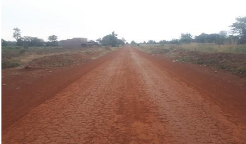
A section of Kapir-Ngora-Mukongoro (44km) in good condition after the 5 th cycle of mechanized maintenance under term maintenance
