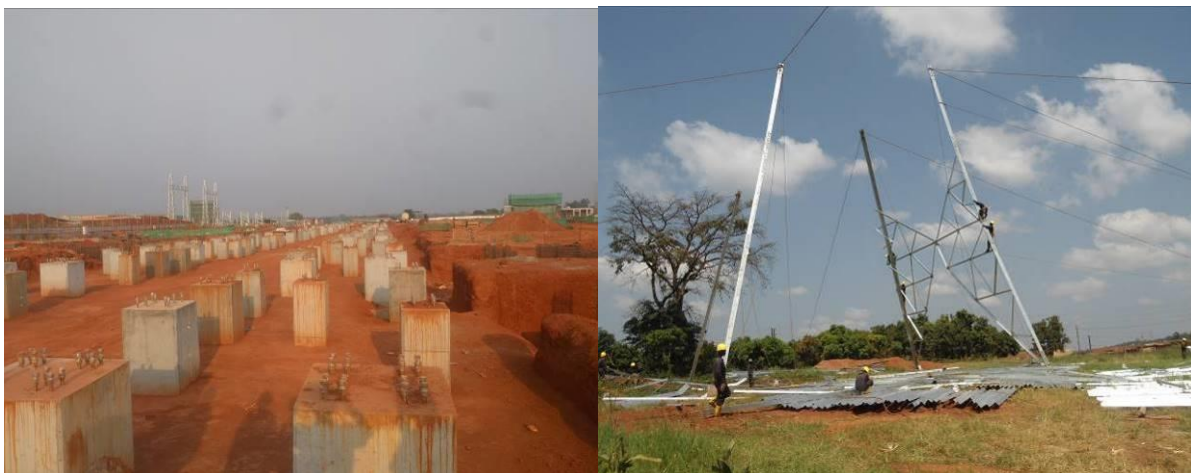
L-R: Completed foundation works at Karuma substation, Contractors undertaking tower erection works on the Kawanda-Karuma T-Line
