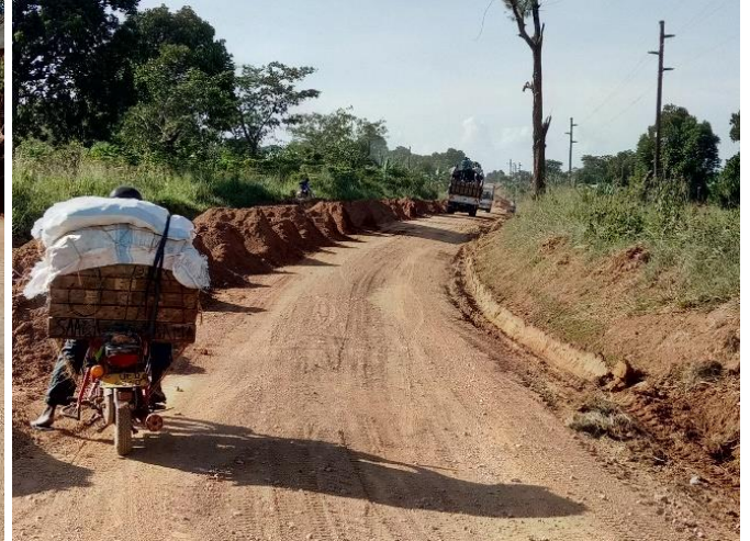
Dumped gravel heaps at km 5+400 along Taba-Kyesiga-Dimo road
