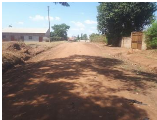
Opolot Odelle Road (0.3 km) that was worked on under RMeM in Q2
