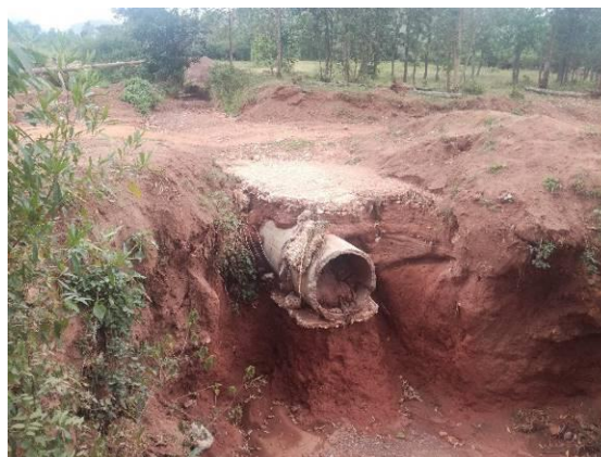
Omungyenyi-Nyanga-Ruyonza road (10.3km): A damaged drift at Km1+300 at a point with a seasonal stream
