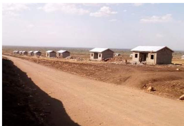
Superstructure of resettlement housing units constructed by Uganda Police in Bulambuli district as at January 2019
