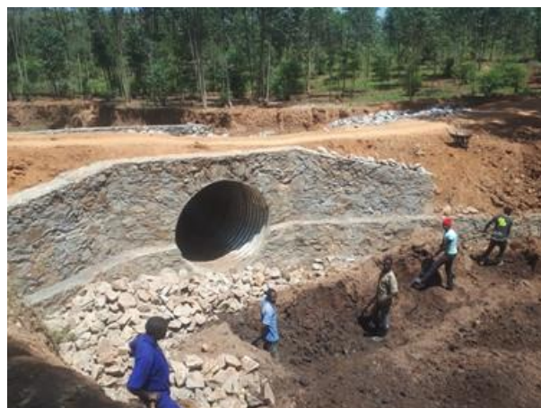
Installation of a 1.2m diameter armco culvert crossing on Mulatsi-Bukiende Road (7.1km) under periodic maintenance
