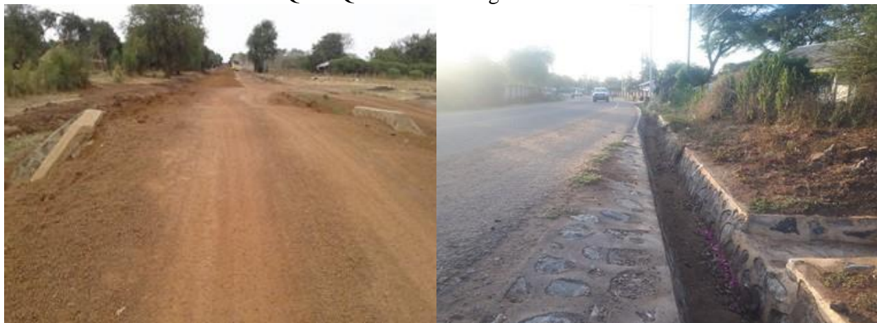
Ongoing gravelling works along Nabilatuk – Angatun Road (25.6km) – Stone pitching works on Moroto Municipal roads under RMeM in Q1
