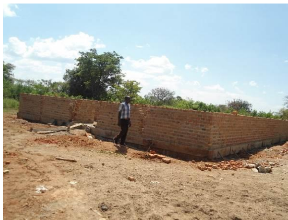
NAGRC financed pig sty under construction at Kasolwe Stock Farm in Kasolwe village, Kamuli District
