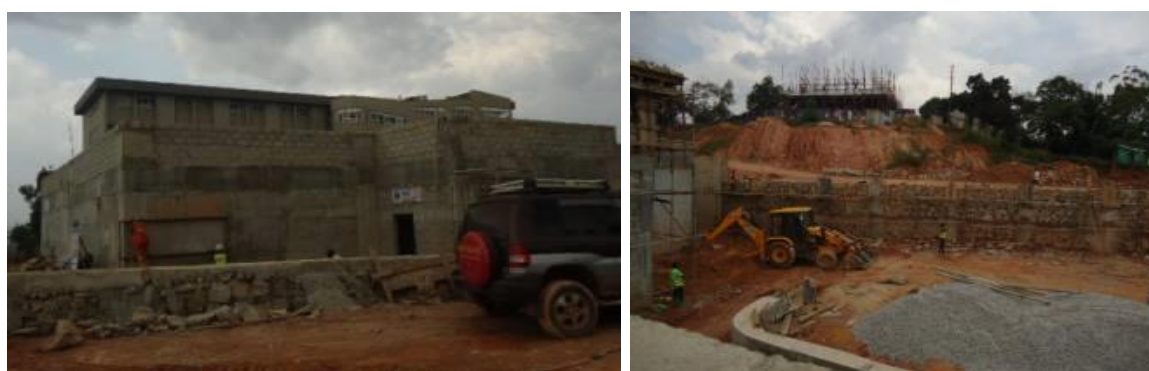
Left: Part of the Radiotherapy bunker under construction. Right: Ongoing external works at the Radiotherapy Bunker Structure-Uganda Cancer Institute. Mulago
