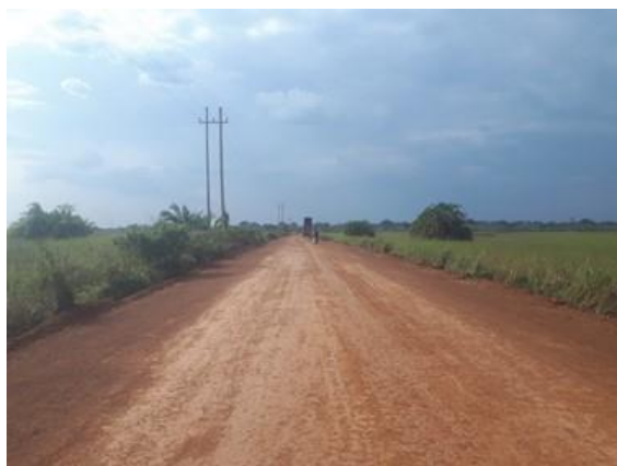
A swamp section Amii - Kidilan - Atura-Aber-Atapara road that was raised and widened during mechanized maintenance under the term maintenance contract in Q2 FY2018/19
