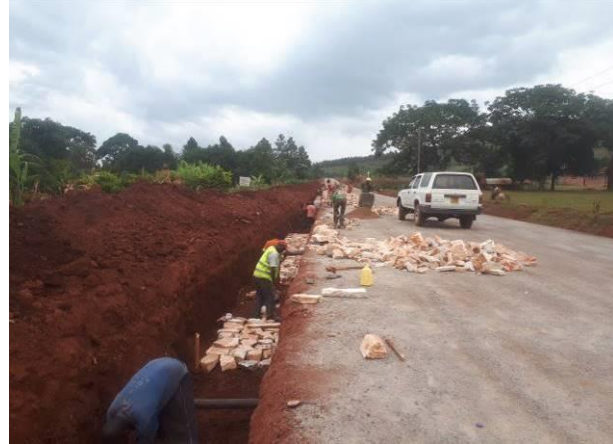
Stone pitching works along the access road to Busoga College Mwiri in Jinja in progress
