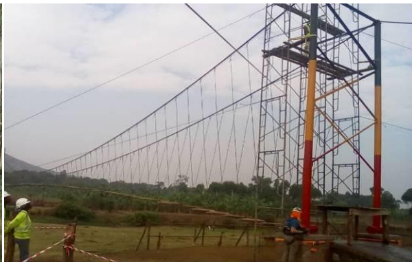
Erection of cables at the Tongole cable bridge site in Manafwa District in progress
