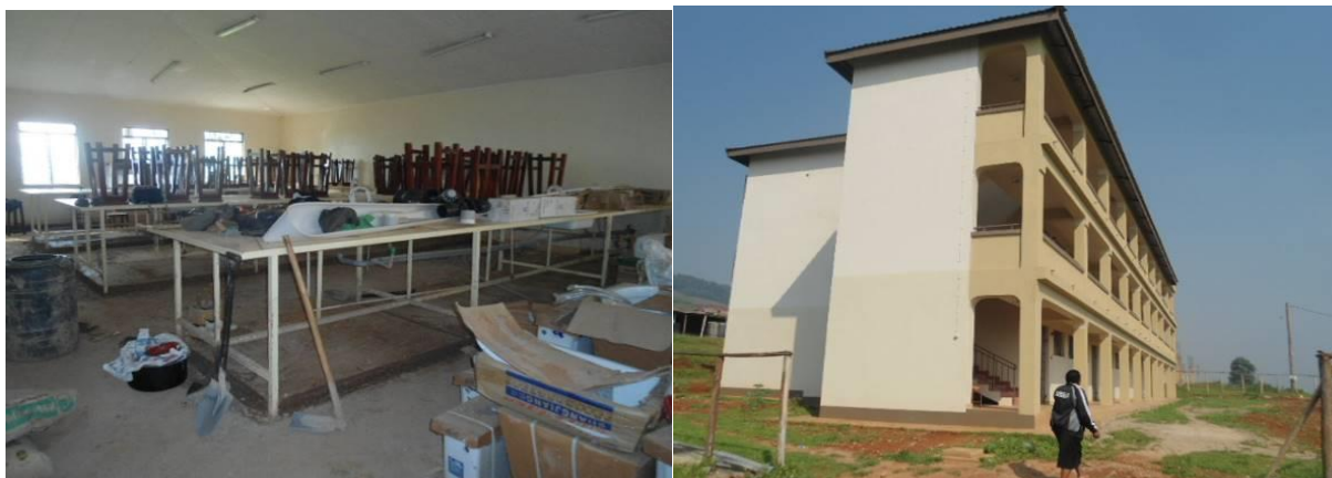
L-R: The biology laboratory under renovation: The General lecture block at Kabale University
