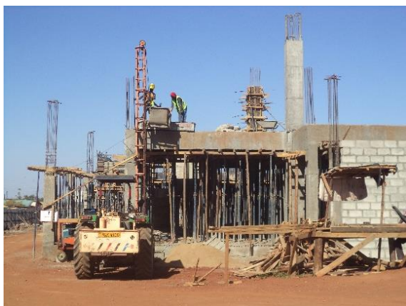
Ongoing construction works: Raising columns to roofing level at Lopedero main market, Moroto Municipal at at January 2019
