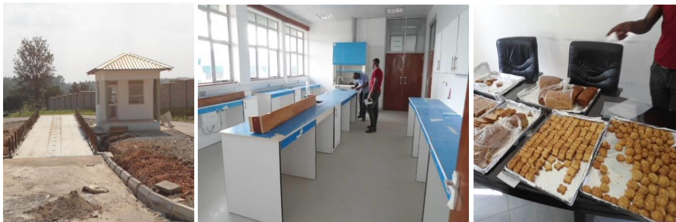
L-R: Installed weighing bridge, furnished laboratories and bakery items presented for sensory tasting at PIBID
