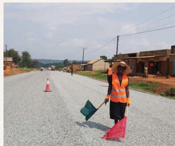
Female Involvement: A flag girl controlling traffic flow on Musita-Lumino road construction project
