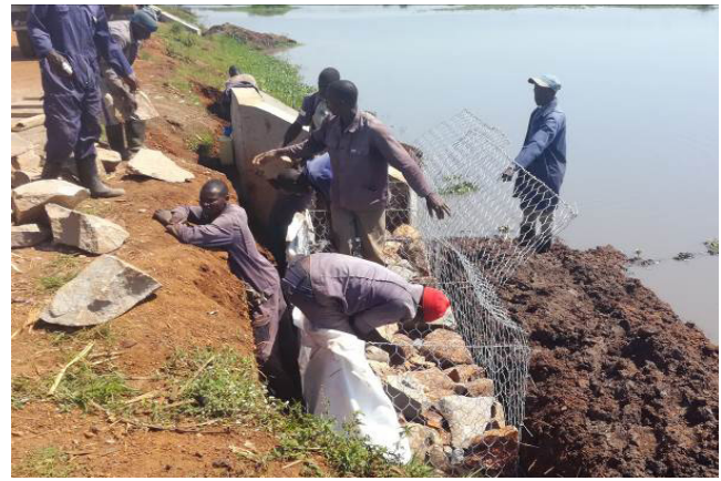
Gabion protection works of the raised embankment undergoing at the Nsokwe swamp crossing
