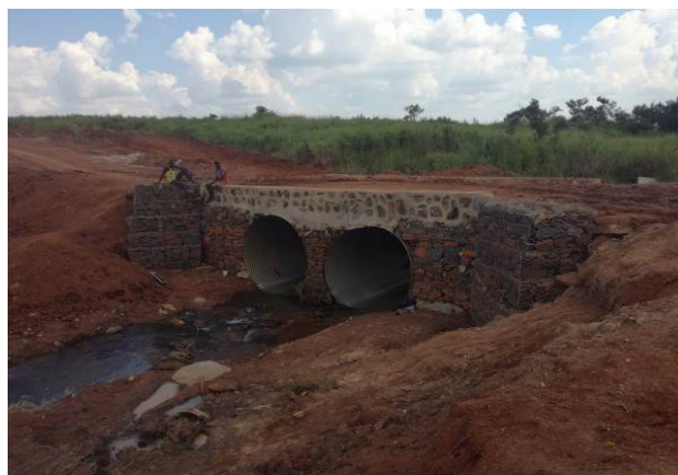
Two lines of 2100 diameter armco culverts completely installed with gabion protect works at the first major crossing on Lungulu-Lebnyec-Arana road
