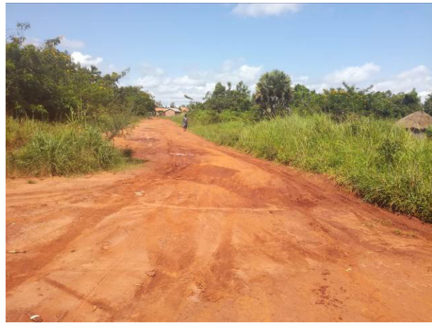
Pece Road: A section of the road whose surface is damaged by surface run off
