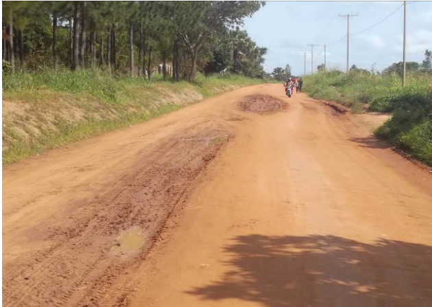
A section of Gulu-Opit-Rackoko Road at Km 4+600 which was defective having been worked on during the rainy season
