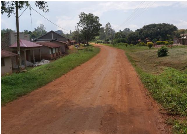
A well gravelled section of Butiiti-Ruhoko Road (25.8 km). works done in Q2 FY 2019/20
