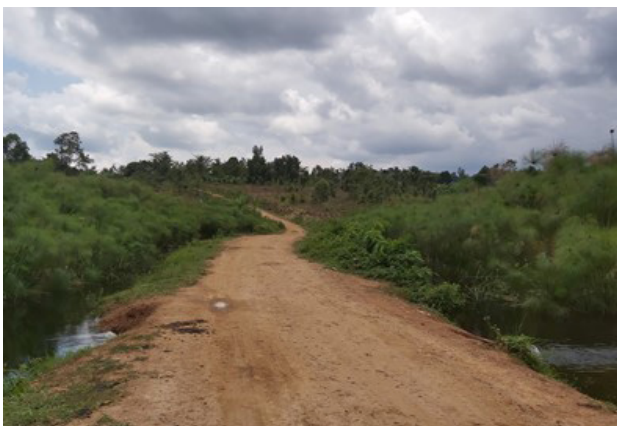
Raised swamp section of Kitenga-Lulongo Road (18.5 km) at km 7+900 – km 8+300. Works were done in Q2
