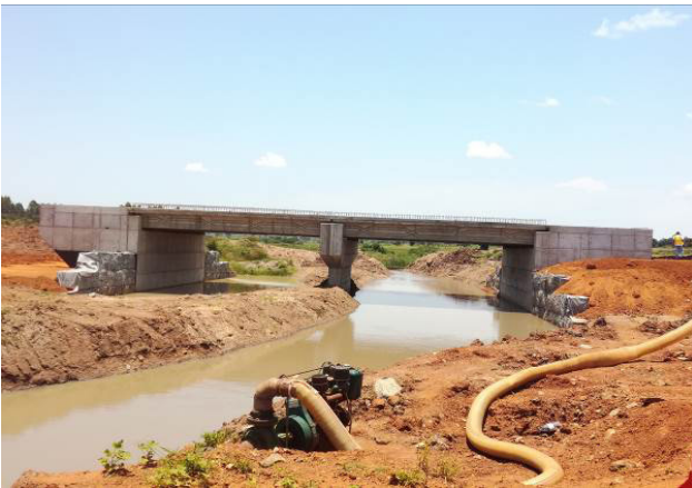
The concrete 24m 2-span bridge at Km 58+711-742 along the Tirinyi-Kumi-Pallisa Road section
