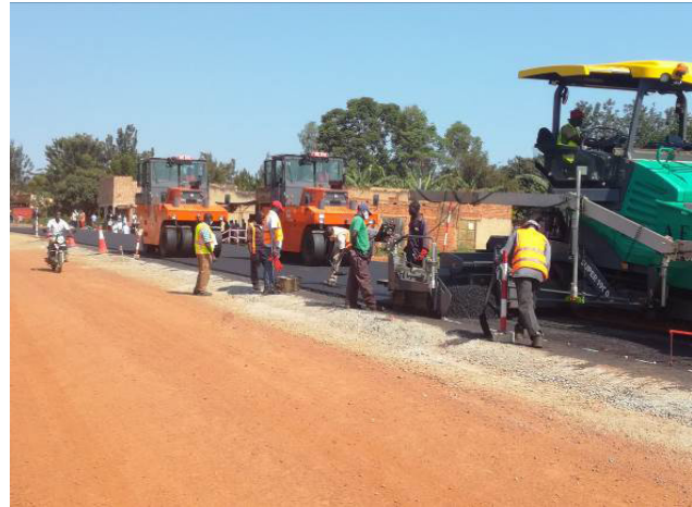
Laying of the asphalt concrete layer at Km 33 along the Pallisa-Kamankoli Road
