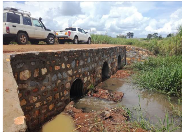
Emergency intervention of two 1.5m and one 1.2m diameter Armco culverts on Wante-Nabalongo road at km 0+600
