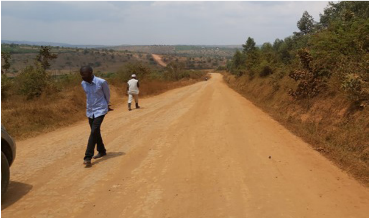
A graded section of Rugaga Ntantamukyi Road(30km) awaiting gravelling works under the framework contract
