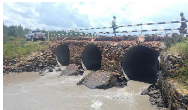
The 2.5m diameter Armco culverts installed at the Komorotot Bridge on the border of Bukedea and Pallisa District
