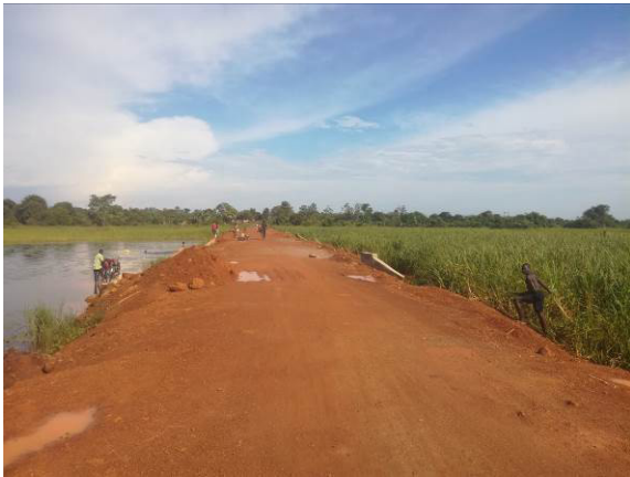
A raised section of the Kangai Swamp crossing at the border of Dokolo and Kabermaido District
