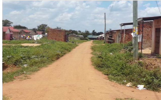
Ekemu Road: A graded carriageway with over grown grass in the road side drains
