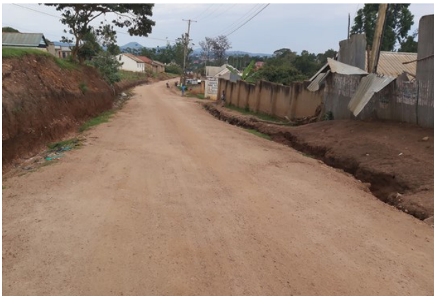
Nkanaga-Kyamakansi Road (2.5 km) received periodic maintenance. The sides were eroded by surface runoff
