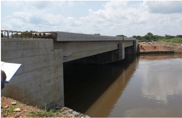
Waiga bridge on Hoima-Wanseko Road at km 69+100. Bridge concrete works were completed
