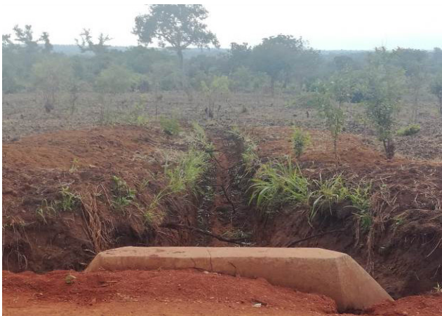
A section of Katikati-Tenamu-Nwoya Road at Km 13+100 where a culvert was installed and a mitre drain excavated
