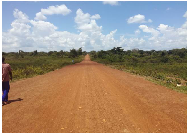
A section of the well graded and graveled approach road to the Ojonai bridge
