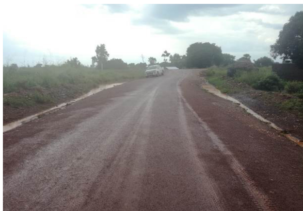
A well-shaped and graded section of Patira Junction-Anaka road at Patira in Nwoya District with water stagnating in the side drains
