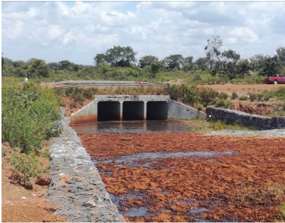
Gabion protection works along the spillway and the Tripple cell Box culvert (3m*3m) of Ojonai bridge in Amuria District
