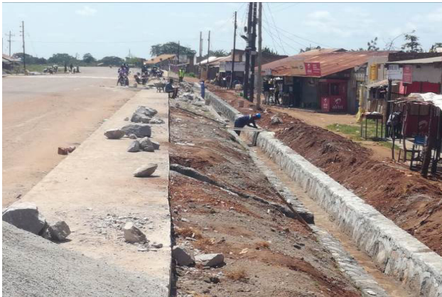
Drainage works of stone pitching to protect water from the road getting to the communities at Were Town Council at Km 20 along Soroti-Akisim Road
