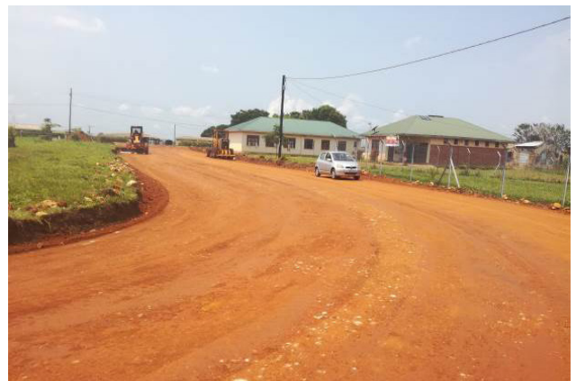
Construction of the subgrade of Erinayo Oryema Crescent (0.35km) at the Nwoya District headquarters as one of the Olwiyo-Gulu town roads
