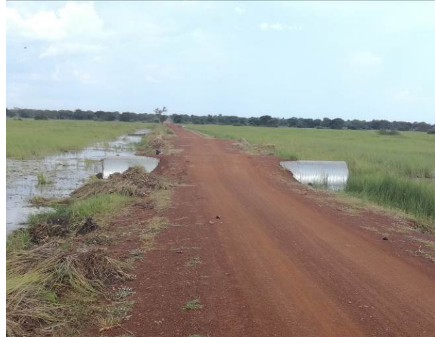
River training, culvert installation and swamp raising works at Km 47+00 in the Amusiya swamp along the Sororti-Gweri-Kapujan-Toroma-Magoro (54km)
