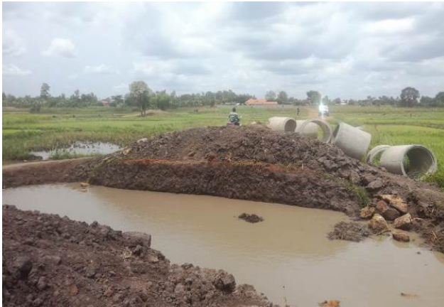
The abandoned culvert installation works at the swamp section a Km 1+000 along the Mugiti-Sekulo-Jami Road
