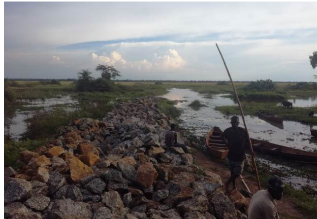
Dumped rock fill at the start of the Amodo Swamp crossing from the Agwata side in Dokolo District
