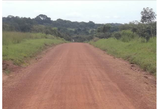
A well graded section of Amuru-Rhino Camp Road at Km 11+ 400A section
