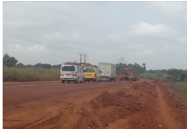
Raising of a swamp section between Km 13 to 14 along the Nakalama-Tirinyi-Mbale Road
