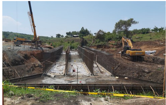
Construction of a three cell box culvert across river Hohwa on Hohwa-Butole Road at km 1 + 465
