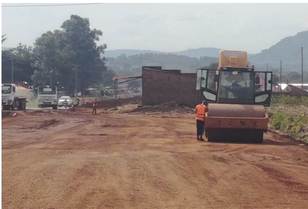
Pavement construction works ongoing in a section with encumbrances at Km 42 along Bumbobi-Lwakhaha Road
