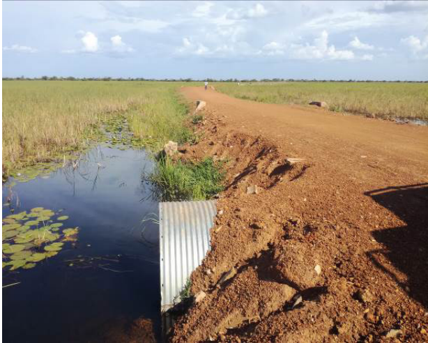
A raised swamp section and an installed culvert in the 6km long swamp of Kapujani at Km 15+200 on the Sororti-Gweri-Kapujan-Toroma-Magoro (54km)
