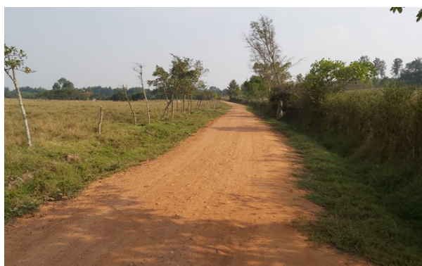
A well gravelled section of Kitokye-Rwenshanku Road (12km), works done in Q3 FY 2019/20
