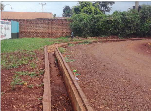
A section of Wange road in Jinja West Division that is well graded and graveled with a concrete lined U-drain.
