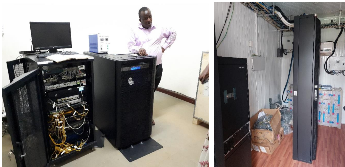
L-R: A compact aggregation site installed under RCIP at Kiryandongo District, and upgraded transmission site with solar power system
