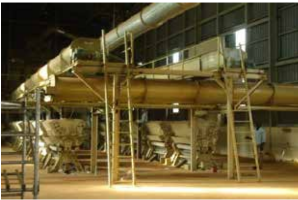
Installed and functioning machinery that required new delinter and grading machines at Pajule Ginning Factory in Pader District for increased production
