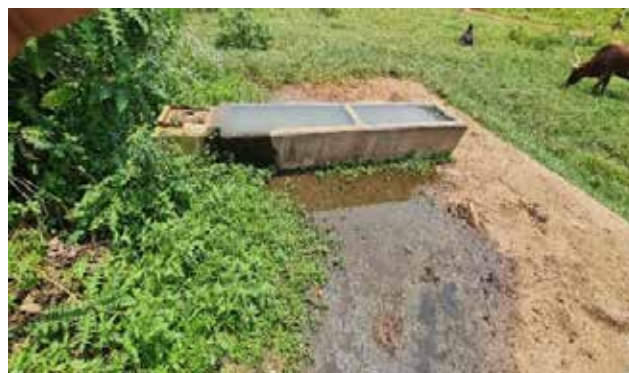
Kagango cattle trough depicting lack of maintenance
