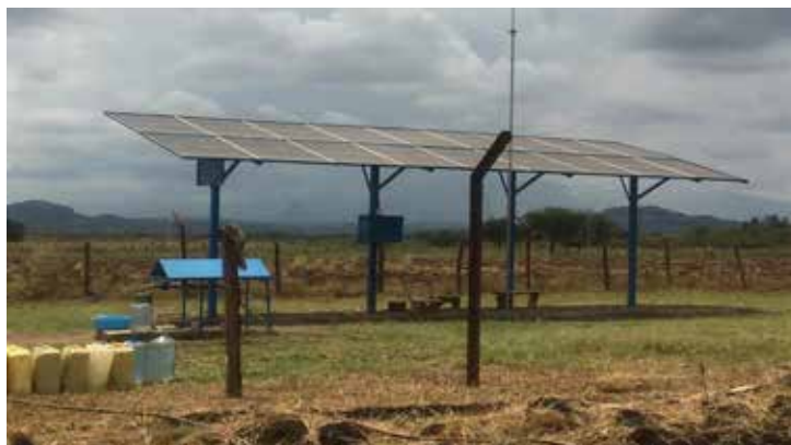
NAADS solar powered irrigation system was installed in Kween District and was functional
