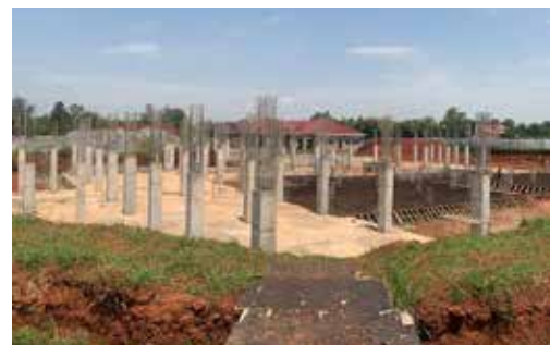
The six-floor Business Development Centre/Centre Teaching Facility stalled at 20% progress at Gulu University 3
