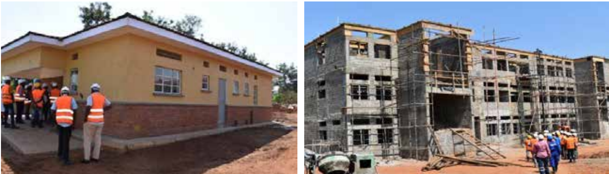
L-R: Construction projects under OFID-Phase II - Multi-purpose hall at 56% progress sickbay at 89% progress and at Nawanyago TI in Nawanyago Town Council, Nawanyago Parish, Kamuli District
