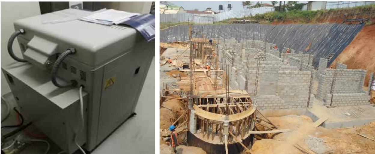
L-R: Construction of laboratories at Fort Portal RRH and a procured autoclave at Mbale RRH
