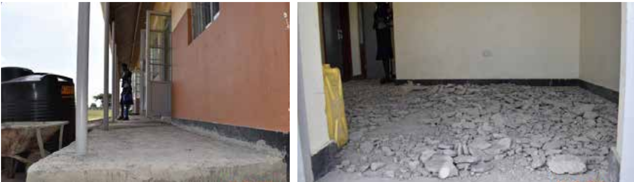
L-R: Failed floor hacked for rehabilitation at Priscilla Girls Comprehensive Secondary School in Katakwi District
