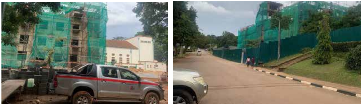
Left-Right: Construction and restoration of the Main Administration Building at Makerere University at 40% progress
