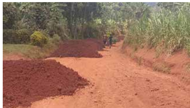
Lugazi Municipality: Gravel heaps damped on a graded and shaped section of Dangale-Kimwany road in Najjembe Division
