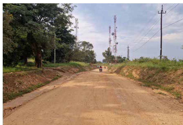
Arua UNRA Station: A section of Nebbi-Goli Road (17kms) after routine mechanised maintenance
