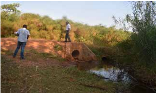
Kakumiro district: A culvert installed at a section along Bukuumi-Kibijjo-Isunga Road at kms 2+000
