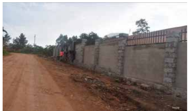
Ongoing construction of a boundary wall aimed at widening the road at Kms 2+680 along the Bulindo-Nsasa-Namugongo (4.56kms) Road in Kira Municipality
