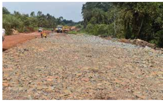
Rock fill in a section with a high water table in the Budongo Forest at Kms 31+620 along the Masindi-Biiso (43kms) Road Project on Oil Road Package 5
