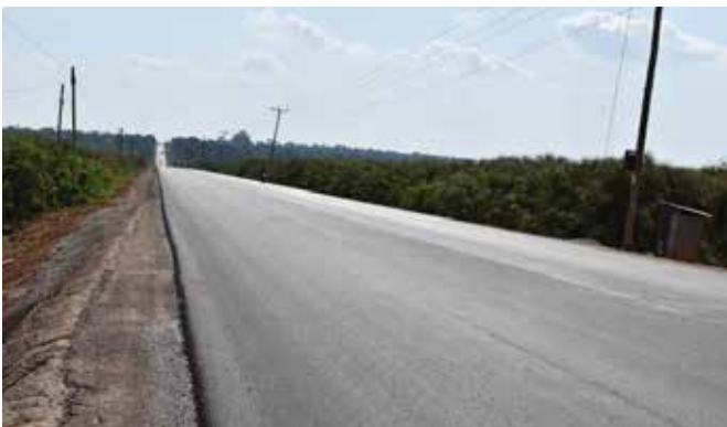
Mityana-Mubende Road: Asphalt surfacing between Kms 11 to 12 with a site toilet in the background
