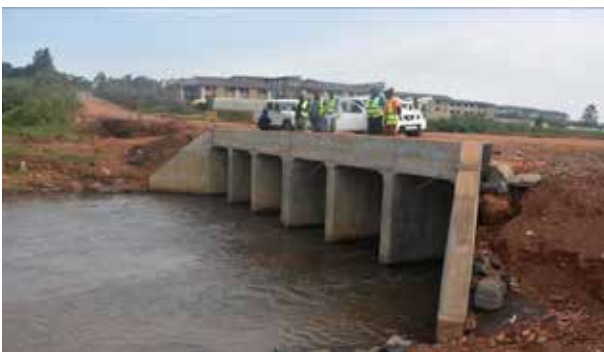
A 2.5m by 2m six-cell box culvert in a swamp crossing along the Kitukutwe-Kiwologoma (4.54kms) road in Kira Municipality
