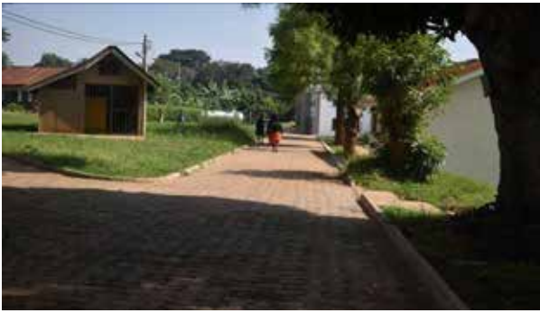
One of the completed walkways with pavers and kerb lines at Gayaza High School in Kasangati Town Council
