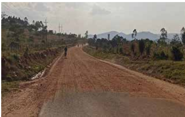
Mbarara UNRA Station: A well-graded and shaped section at the start of the Kikagati-Kafunjo (30kms) Road
