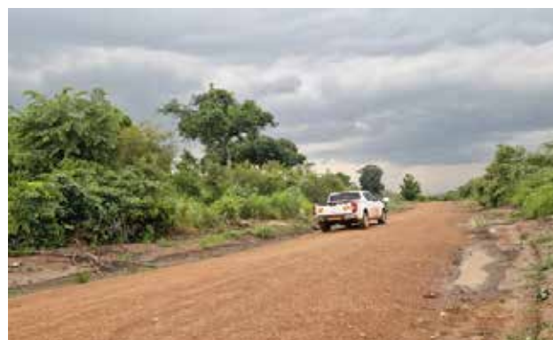
DRRU-North: Ibibiaworo Pakele road (7kms) was rehabilitated in Adjumani District (fully gravelled)
