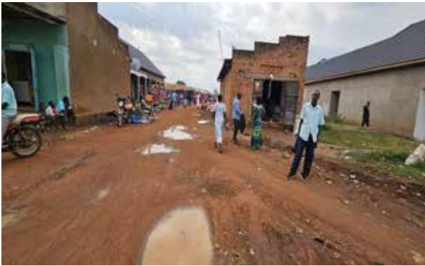
Unstabilised base and house on RHS within the road alignment at Kibuku TC roads along Market Street Road
