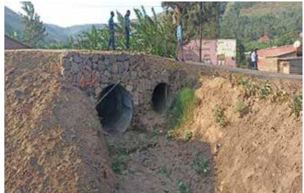
Mbarara UNRA Station: 1.8m and 1.2m Armco culverts installed with gabion end structures at Ruborogota TC along Kikagati-Kafunjo (30kms) Road At Kms 10
