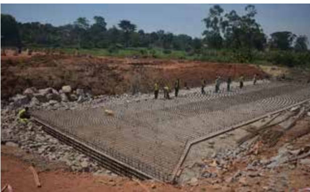
Foundation works for a box culvert along the Kasangati-Matugga Section on the Kira-Matugga Road Project
