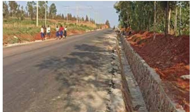
Ongoing stone pitching works of the side drains in a section that has received asphalt at Kms 2+580 long Kafunta–Buwampa Road (9.5kms) in Njeru Town Council
