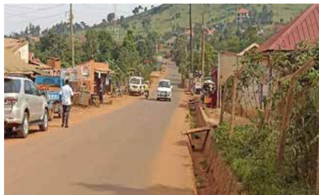
A completed paved section with a stone-pitched side drain on the Nansana-Kireka-Bbira Road in Nansana MC constructed using Probase Technology
