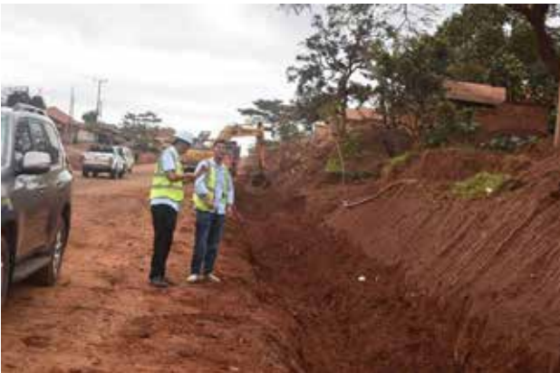
Excavation works for the roadside drain at Ggangu along the Munyonyo Spur on the Najjankumbi-Busabala Road Project
