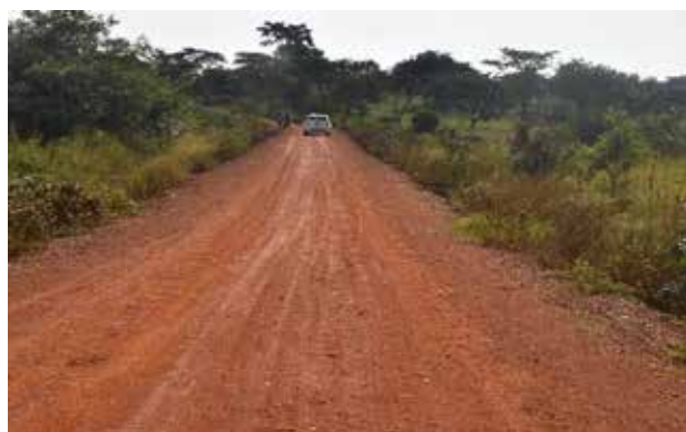
DRRU-Central: A completed section at Kms8+000 on Bbaale-Gira-Kanyogoga (10.3kms) used as access to the Bulwandi-Gyra swamp crossing from the Kayunga side
