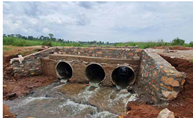
Jinja District: Three lines of concrete culverts installed on Busoona- Budiima road at Nabukosi swamp
