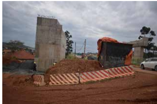
The abutment and pier works for the Lweza-Lutembe Vehicle Overbridge at Kajjansi along the Munyonyo Spur on the Najjankumbi-Busabala and Munyonyo Spur Interchange Project
