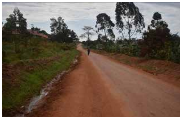
Mpigi UNRA Station: A well-formed shaped section with a surface in good condition of Mitalamaria-Bulo-Kanoni Road at kms 27+800
