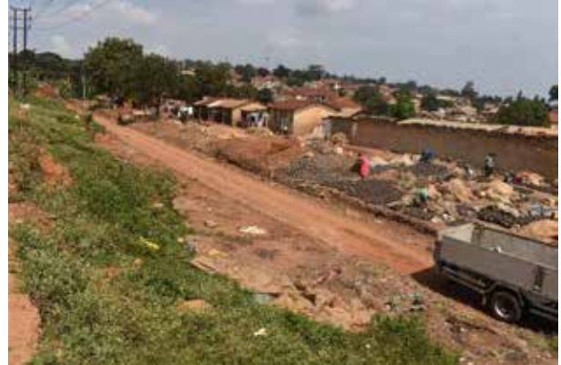
A compacted section where the old rail tracks were removed at Namboole
