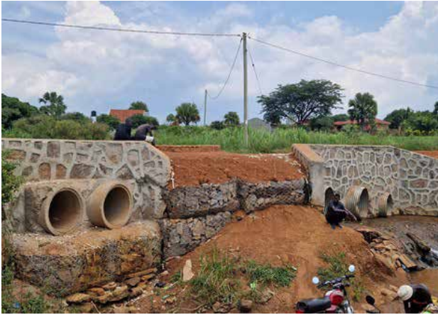
Gulu UNRA Station: Culverts installed along Gulu – Airfield road (4kms) as part of emergency intervention
