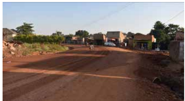
A prepared subbase layer in preparation for surface dressing and an installed Armco culvert without end structures along Matu Road in Busunjju Town Council
