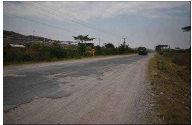
Kasese UNRA Station: A section of Kikorongo-Mpondwe road that was patched with gravel at kms 6+000
