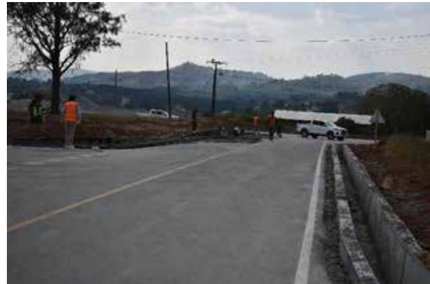
Ongoing works on one of the Kyamate Access roads in Ntungamo Municipality
