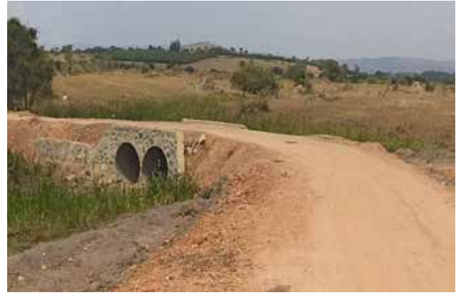
DRRU-West: A well-raised swamp section with two 1200mm diameter Armco culverts with headwalls along Mile 8-Katojo-Rwentanga T/C (5.2kms) Road in Mbarara District
