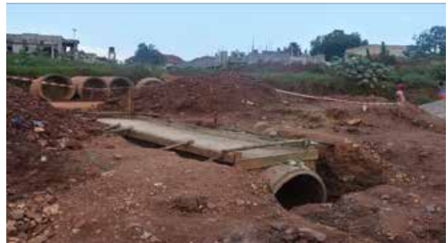
Installation at half road with an encased concrete pipe culvert installation of 900mm diameter along the Shimoni PTC (3.4kms) Access in Kira Municipality
