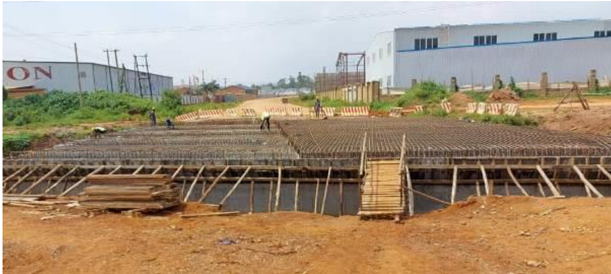
Box culvert construction in South A Estate of KIBP across Namanve River
