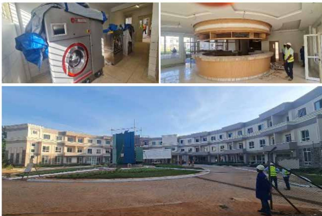
Top left: Some of the laundry equipment procured for the Uganda Hotel and Tourism Training Institute (UHTTI). Top right: Renovation works at the reception area of the UHTTI. Bottom: Front view of the UHTTI under renovation in Jinja District
