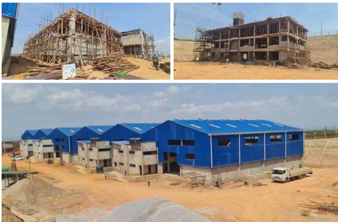
Top left: production unit 4 under construction. Top right: One Stop Center (trade house) at Entebbe under construction. Bottom: Substantially completed production units 1, 2 and 3 at the Entebbe International Airport Free Zone
