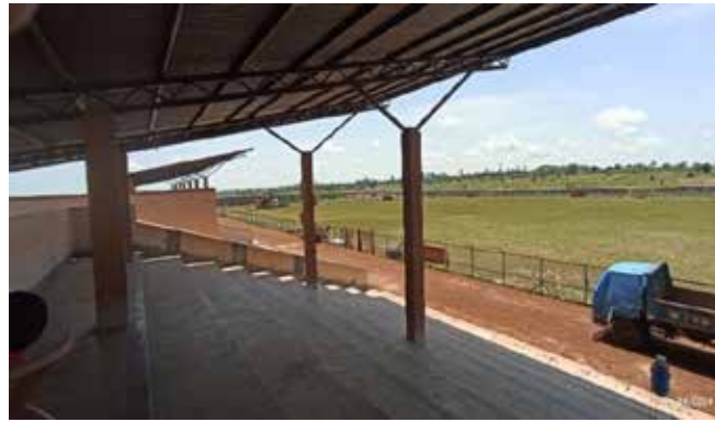
Ongoing construction of a play field at Leju Town Council in Terego District
