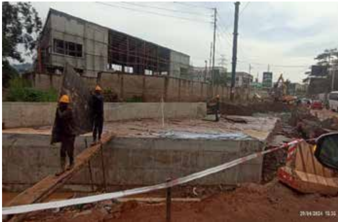
Box culvert works along the Old Port Bell/Spring road in Nakawa Division
