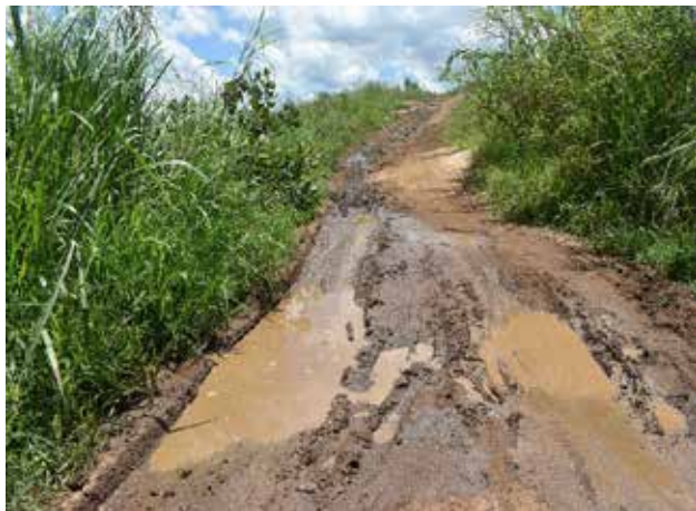
ACDP supported Karuteete-Rubona-Kyakazihire road choke in Kibaale district was in poor condition as rehabilitation was partially done and abandoned by contractors
