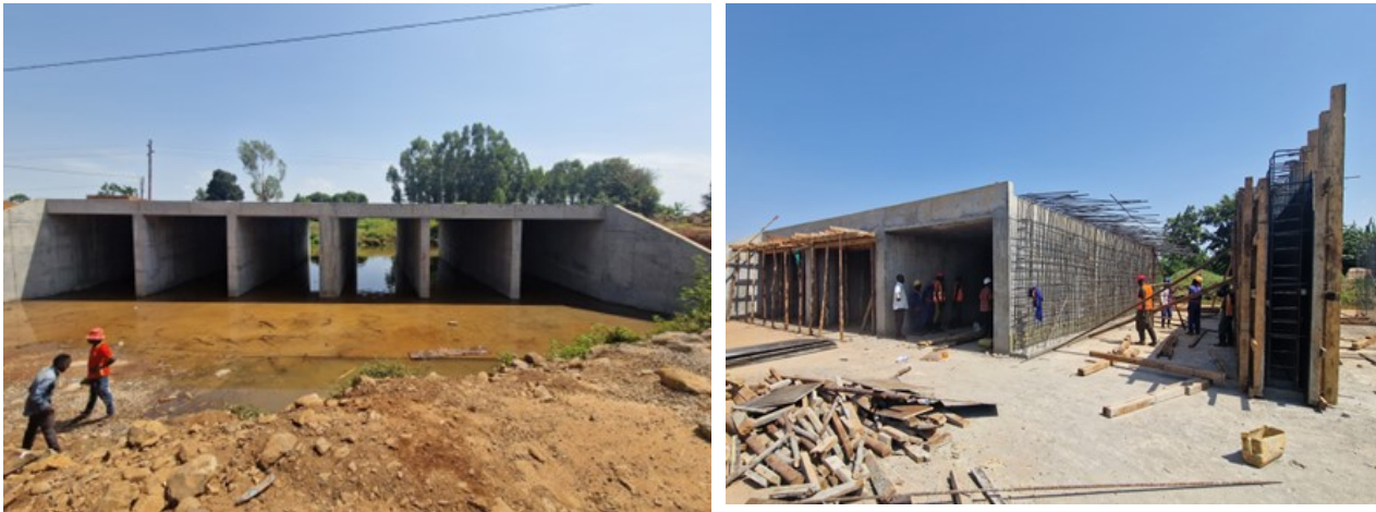
Muyembe- Nakapiripiriti Road Project: L-R: Completed six-cell box culvert along, Ongoing construction of a four-cell box culvert
