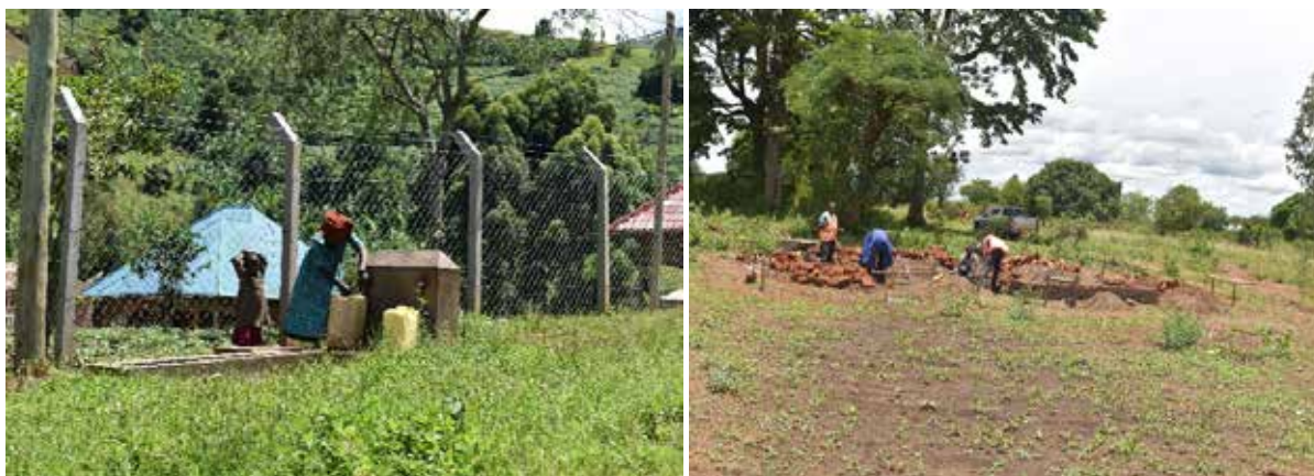
Left: Beneficiary fetching water at the free water point in Bunaiga in Bunyangabu district, Right: Ongoing civil works at Kanapa piped water supply in Kumi District
