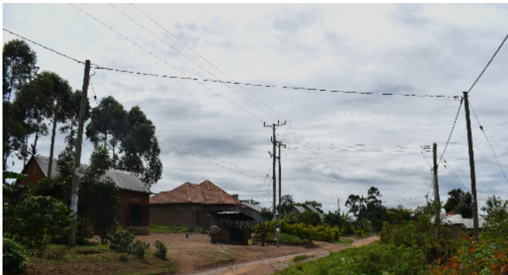
One of the completed grid extensions at Nsambya 2 trading centre, Kyotera under additional lots (Lot 12)
