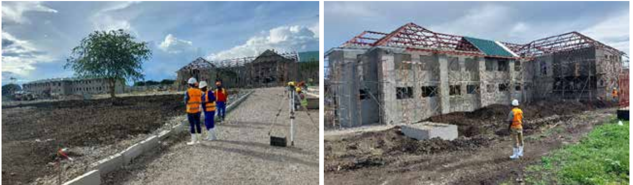
L-R: Landscaping of the front compound and a partially roofed UWRTI in Kasese
