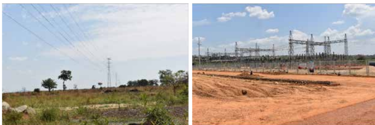
L-R: Completed Gulu-Agago transmission line; On-going civil works at the Agago substation switchyard
