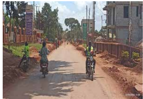
Ongoing works of the subbase along Ssuuna Road in Makindye Ssabagabo Municipality
