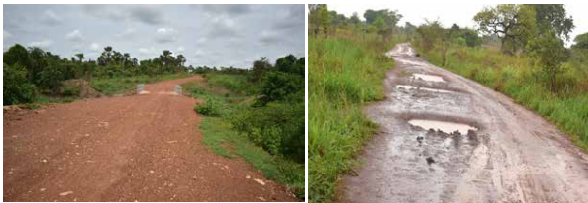
L-R: Rehabilitation of corner Pa Lagara-MonrocMarket(14.3Km) climate resilient CAR in Bugangatira subcounty Gulu Clogged gullies at corner-Agula-Dino-Malaba (35.5Km)
