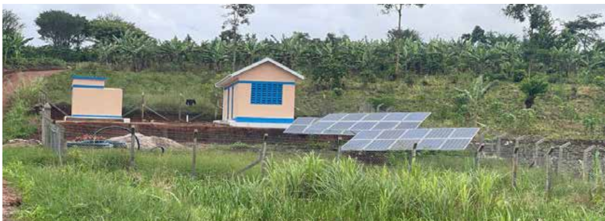
A pump station at Kvamusisi solar powered water supply scheme in Mitvava district
