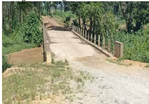
The Ishasha bridge at the border of Uganda and DRC which is among the works that are yet to be done.
