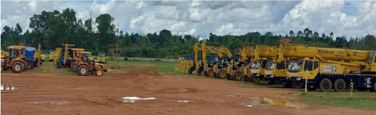
Technical Service Centre equipment at Lyantonde Parking yard
