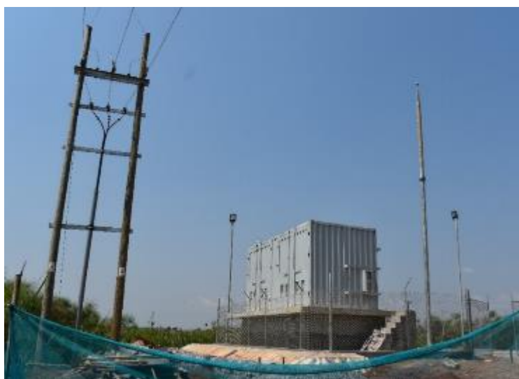
Bottom: A switching station for the submarine cable at Bukakata for grid extension to Kalangala (Lot 6)
