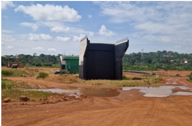
Completed abutments for a bridge interchange at km 28+00 along Busega- Mpigi Express Road Project
