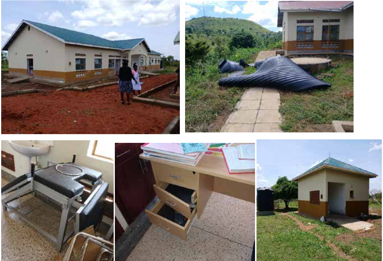
Clockwise: Incomplete Maternity ward at Binya HCII Omoro district, busted water tank at Mudande HCIII Kasanda district, stand alone laboratory at Awoo HCII Omoro District and Broken furniture and equipment at Mudande HCIII
