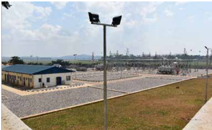
Newly completed 132/33kV substation at Kabale, Entebbe connected more than 15 MVA of load
