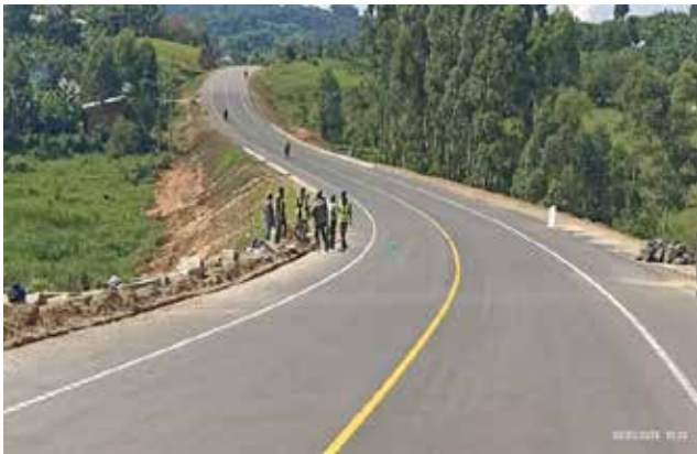
The section at Km 5 which was affected by delays in acquisition where works were ongoing
