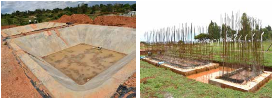
L: Constructed wetland ponds for the Ngora FSTP in Ngora district; R: Steel works for the intake and sedimentation tank for Namasale WSS in Amolator district
