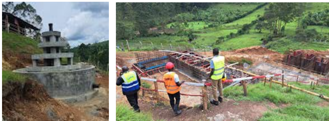
L: An aerator; R: Water treatment plant works for Bitsya GFS in Buhweju district
