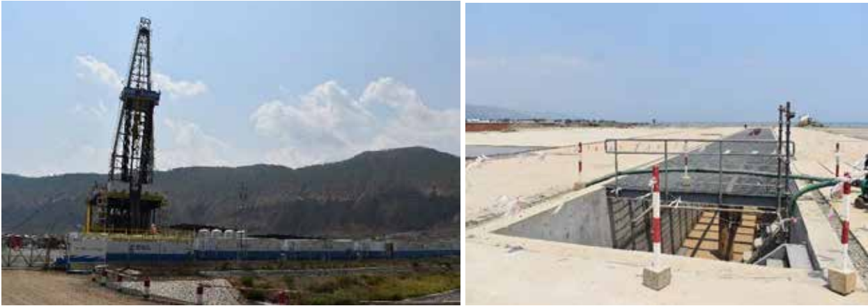
L-R: An operational drilling rig at well pad 2 in Kingfisher area; Ongoing civil works at well pad 1 for directional drilling in the Kingfisher area
