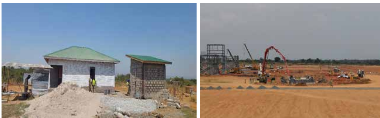
L-R: Foundations works for the main pipe rack at Tilenga CPF; Works at a resettlement house in Buliisa district
