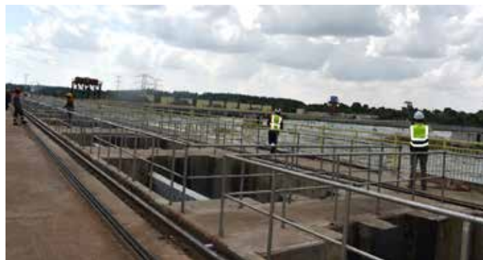
R: Karuma HPP intake section, with missing log boom
