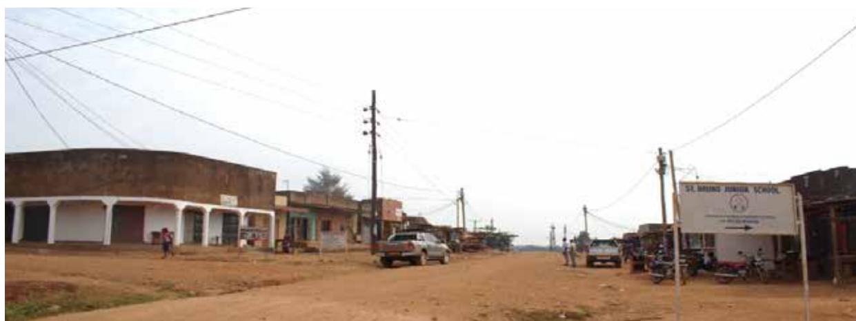
Completed grid extension scheme in Kiwumu TC, Mukono District under ERT III
