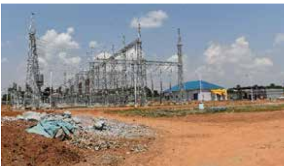
Completed plant house building, equipment structures and busbar gantries in the new 132kV Kole switchyard
