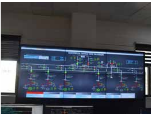
L: Installed plant operation and control screen for Karuma HPP
