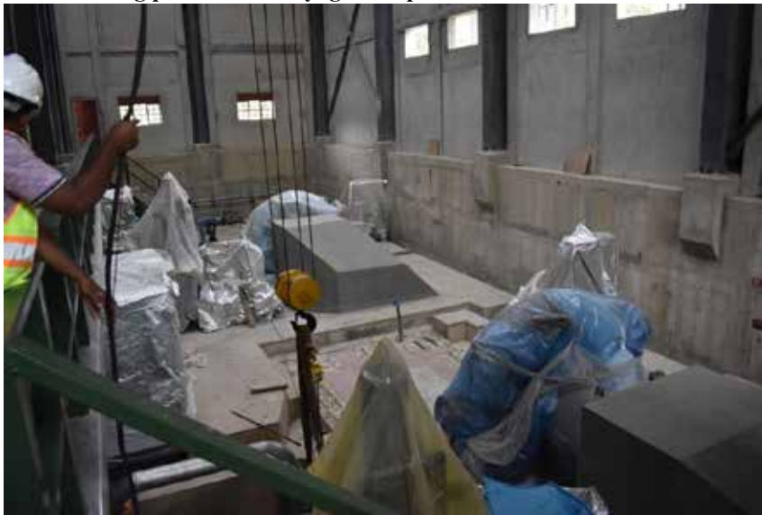
The two installed turbines in the Nyagak III HPP Powerhouse
