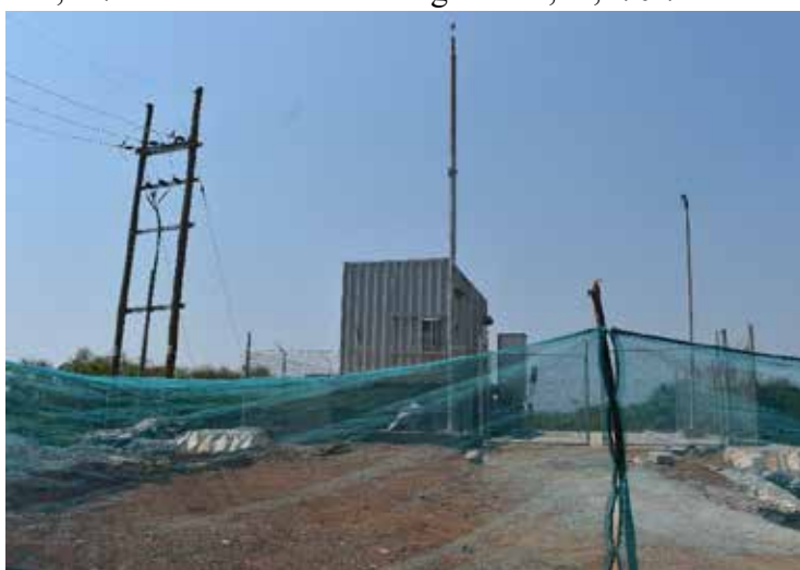
One of the two installed switching station for Bugala marine cable at Bukakata
