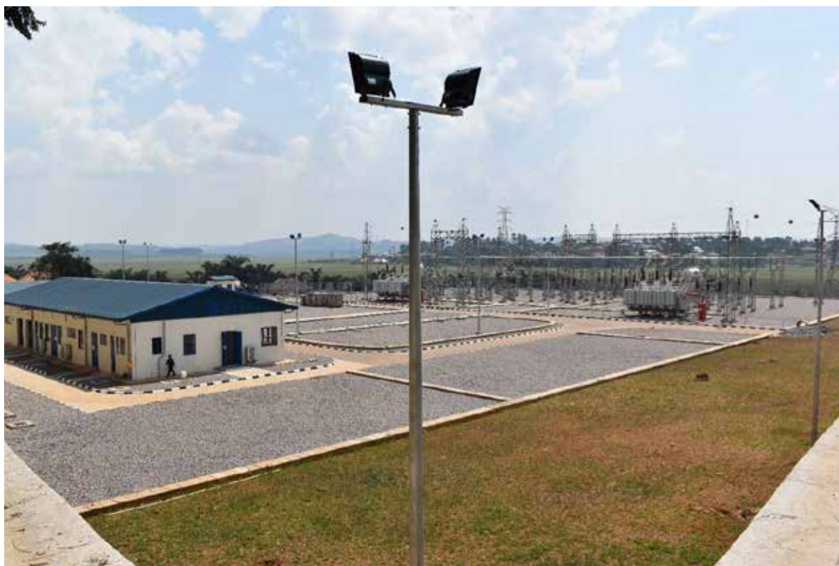
Completed 132/33kV Entebbe Substation
