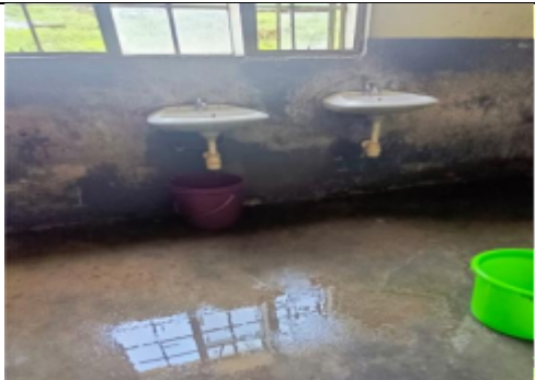
stagnant water seen in Ruth Okwele hall because of leaking sinks in the bathroom waiting area
