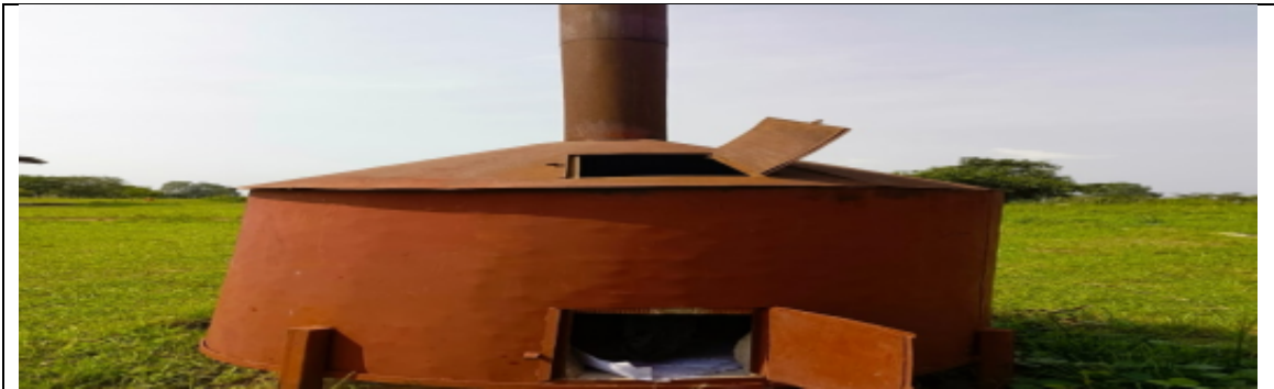
The non-functional incinerator above as seen at Augustine Ousban Hall Annex 1
