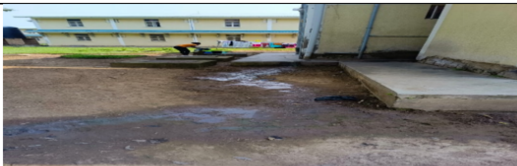
Sewer leakages seen from the rear view of Augustine Hall
