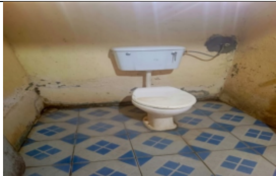
Water seen stagnated in a bathroom/toilet at Nagongera Campus- girls' hall
